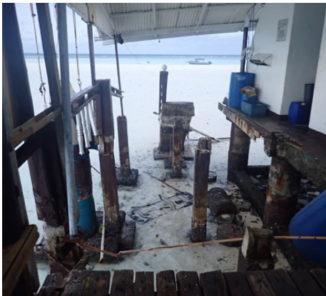
This is where our porch used to be. Our stairs (center) remain steadfast but now leads nowhere.
