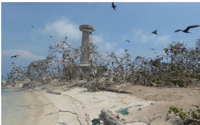
Plate 2. South Islet showing the exposed southeastern shoreline where the seawall has collapsed. Photo: Arne E. Jensen
