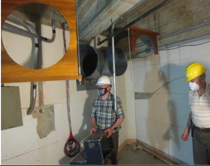
Blower Room with the two 20-HP blowers removed
