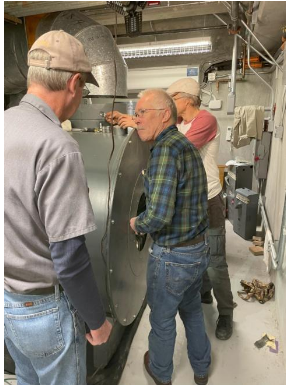
End cover in place, assembly completed. Wayne, Neal, and Ted. All buttoned up!
