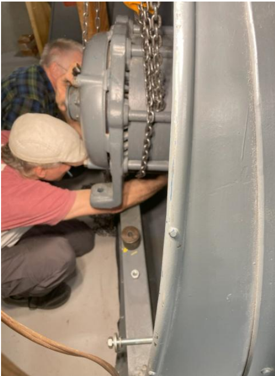
Ted and Neal slide the motor into the blower frame. The 20 HP motor is hanging from a chain hoist mounted on a wooden roll-around frame. The frame was designed and built by the late Bill Schotter. That motor is ?$@#!!! heavy.
