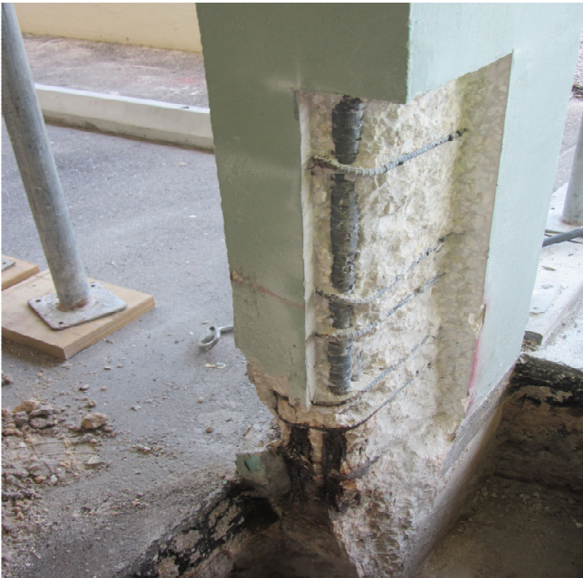
Condition of one of the columns supporting the 02 stack
