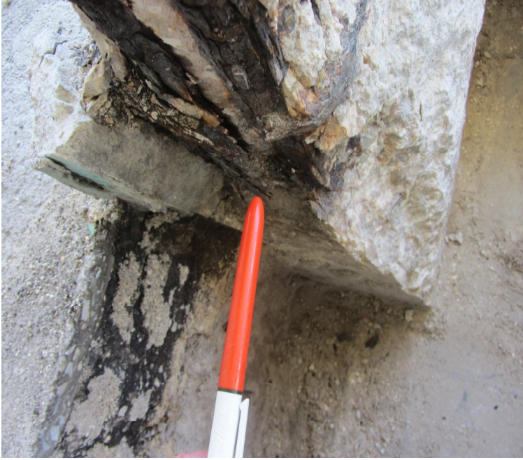
Damage to the 02 stack column.
