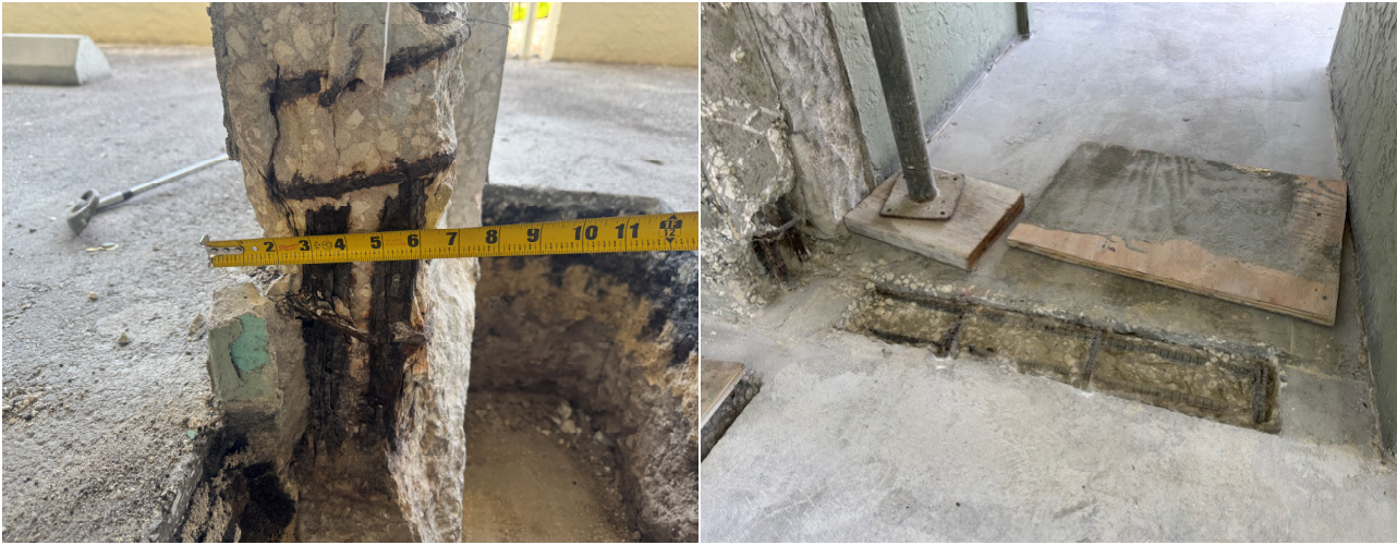
Condition of the column below the 06/07 stacks and concrete damage on various elevator lobbies
