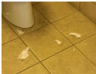
Debris on Floor
