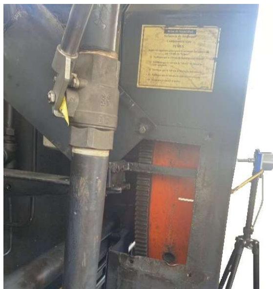
Matching the reference marks with Strobe Light
