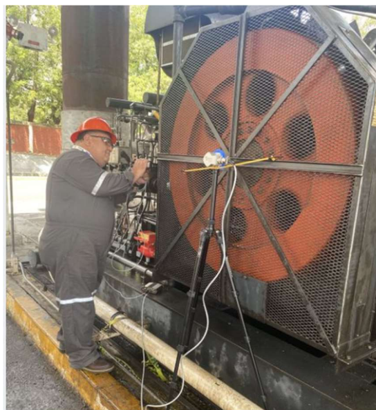
Matching the reference marks with Strobe Light
