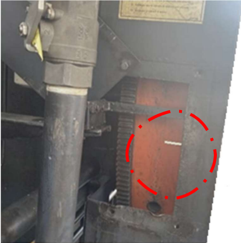
Reflective Tape Mounted on Flywheel.
