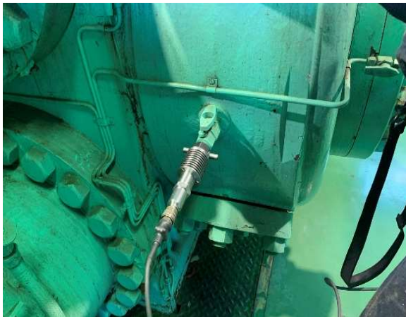
Connecting the Pressure Sensor to the Kiene Valve
