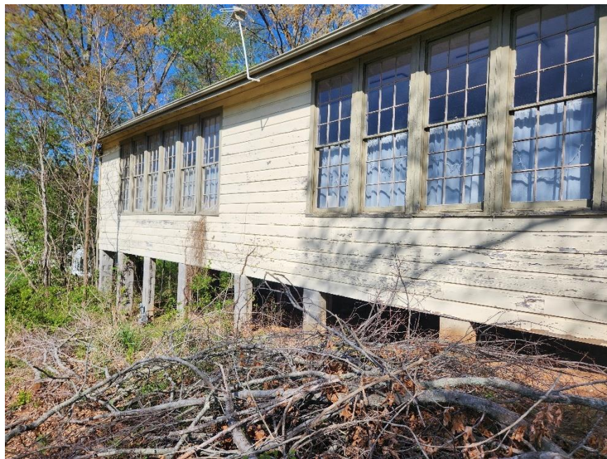
12 13 Figure 3. View of the southeast elevation (back) of the historic Weaverville Colored School. 14 (PSABC 2023)
