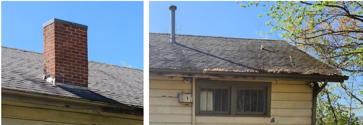
20 21 Figures 4 and 5. Left: View of the brick chimney. Right: View of the leaves and debris in the gutter along 22 the northwest elevation. (PSABC 2023)
