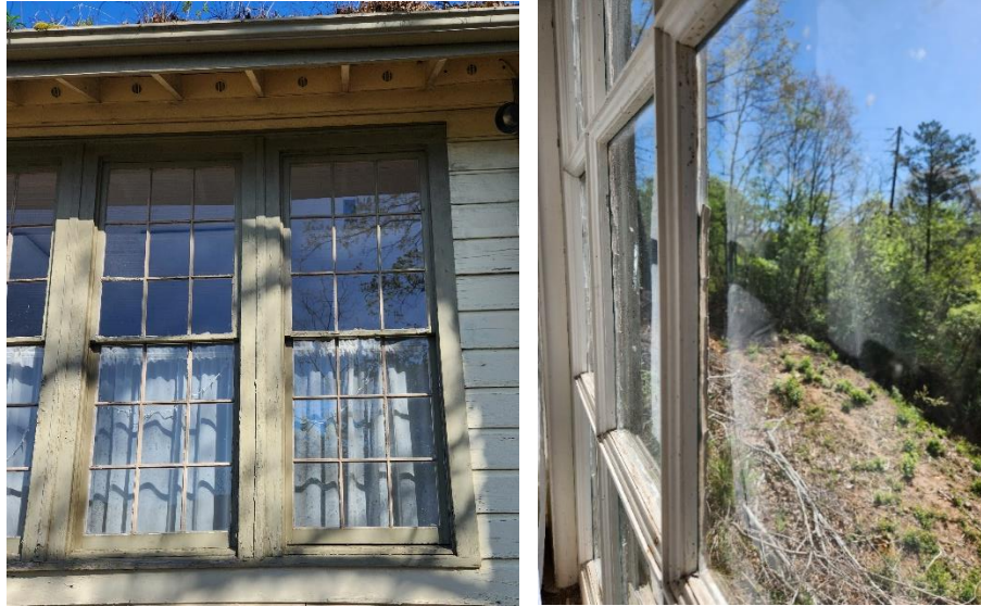
8 9 Figures 10 and 11. Left: View of the large original wood hung windows. Right: Detail view of the muntins 10 and the deteriorated glazing putty. (PSABC 2023)
