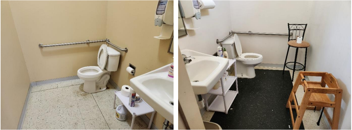
9 10 Figures 18 and 19. Views of the two restrooms within the historic Weaverville School. 11 (PSABC 2023) 12
