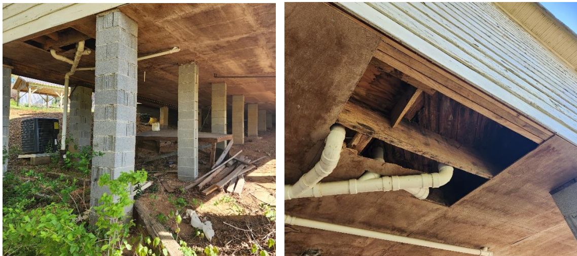
22 23 Figures 8 and 9. Left: View of the CMU piers. Right: View of the hole in the sheathing on the underside of 24 the floor structure. (PSABC 2023)
