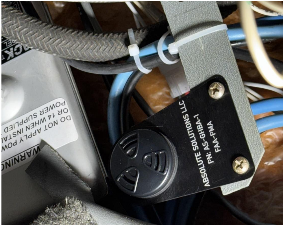
Figure 3-3. AS-GHBA-1 gear horn installed.
