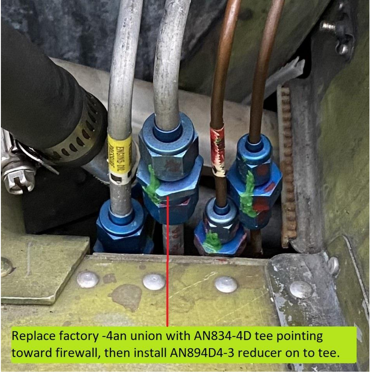
Figure 1-2. Factory Manifold Pressure Union
