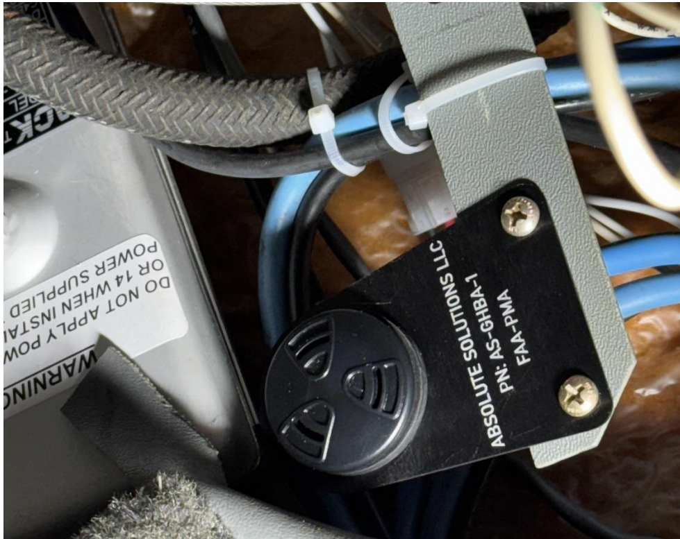
Figure 3-2. AS-GHBA-1 gear horn installed.
