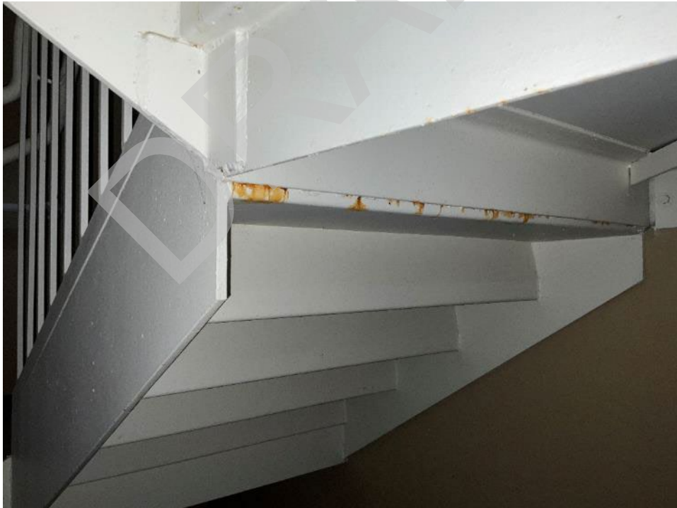
32. View of corrosion under stairs in stairwell.
