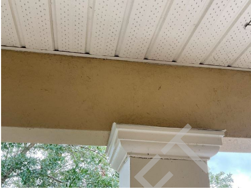
99. View of cracks in the interface of the column top and the column.
