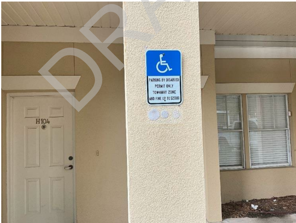
90. View of unrepaired column section unit H104.
