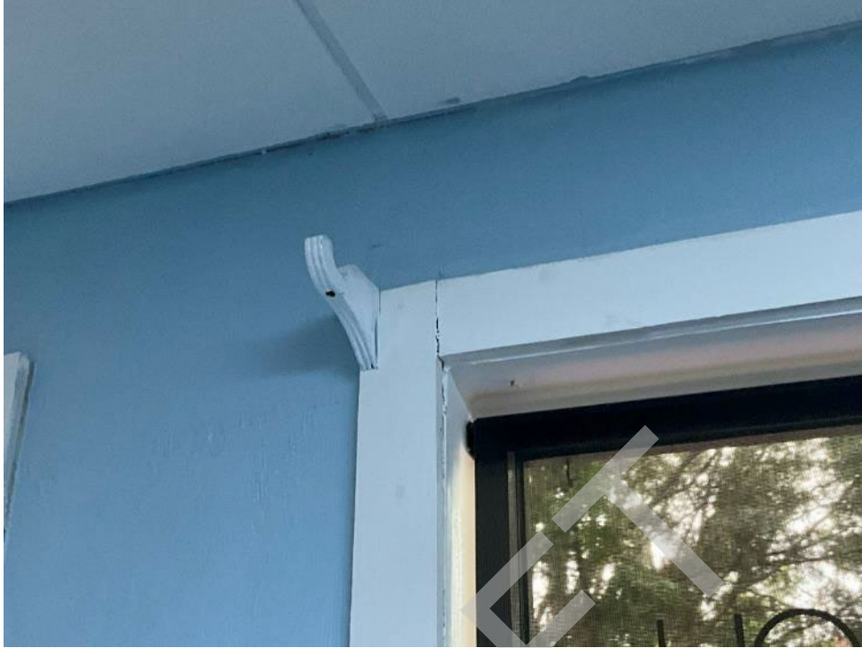
41. View of crack in the finish around a window in suite B-103.
