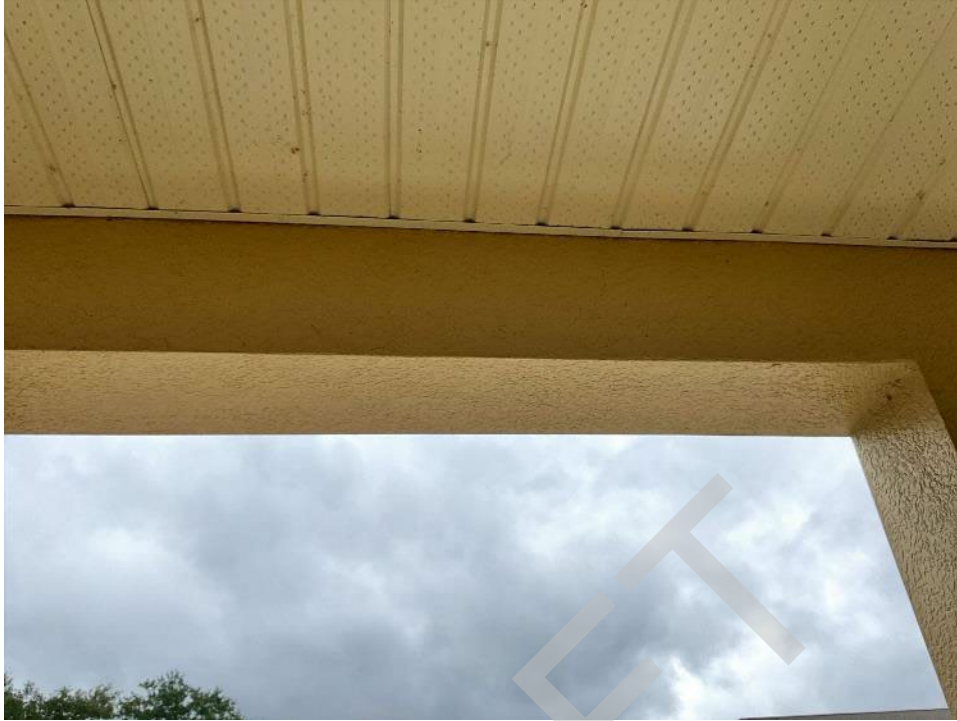
77. View of cracked section along the beam near unit G201. The stucco will need to be removed to expose the beam for Phase II.
