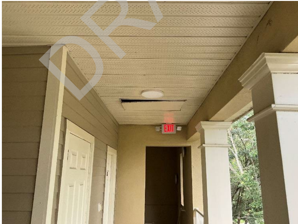
70. View of an opening that is observed to be left open.
