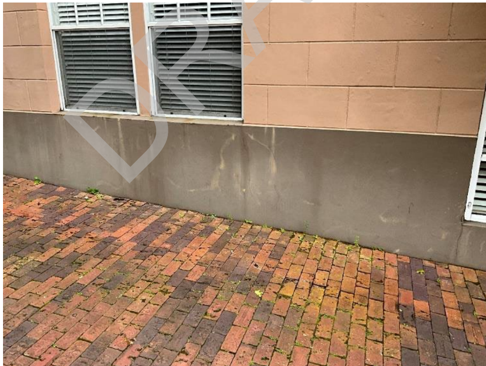
56. View of staining and cracking along the base of the walls around the building.
