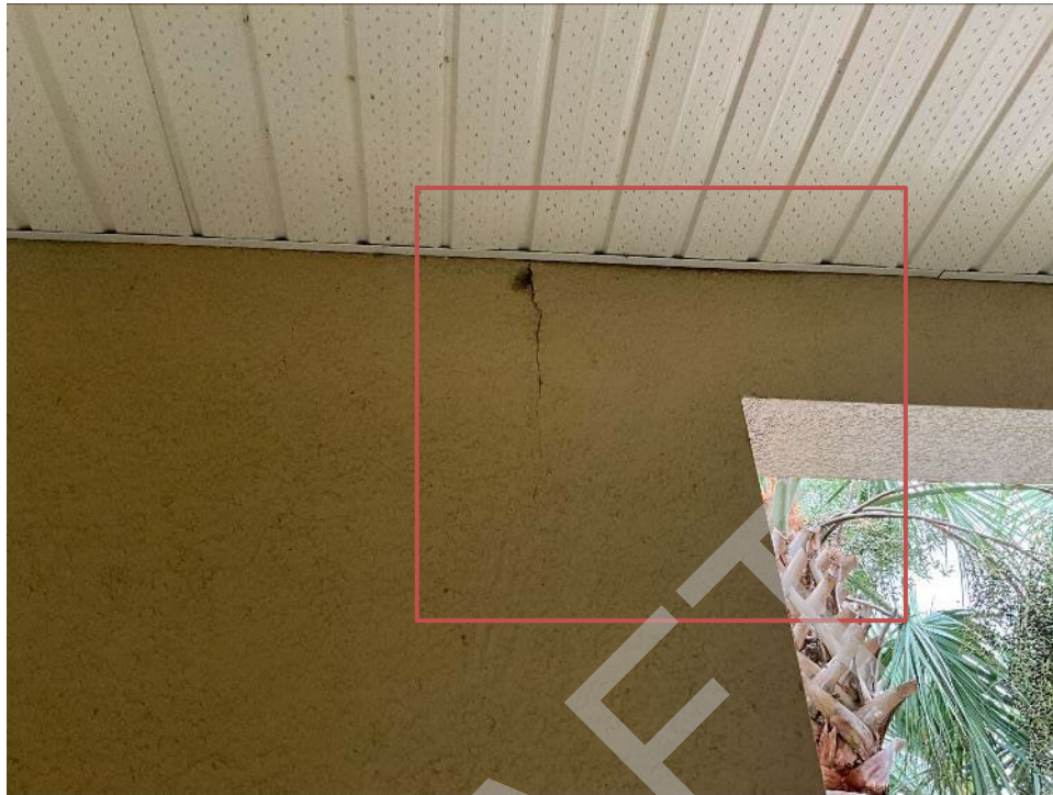
67. View of cracked section along the wall between units F201 and F202. The stucco will need to be removed to expose the column for Phase II.
