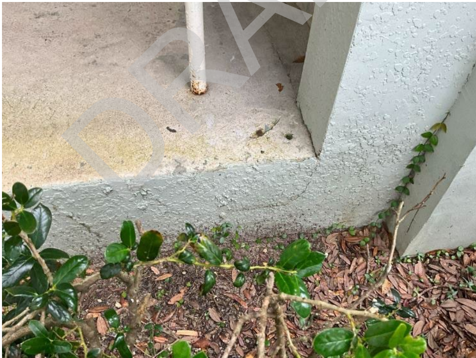
112. View of cracking in the stucco in front of the bottom slab.
