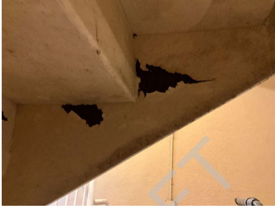
21. View of paint delamination along the stairwells.
