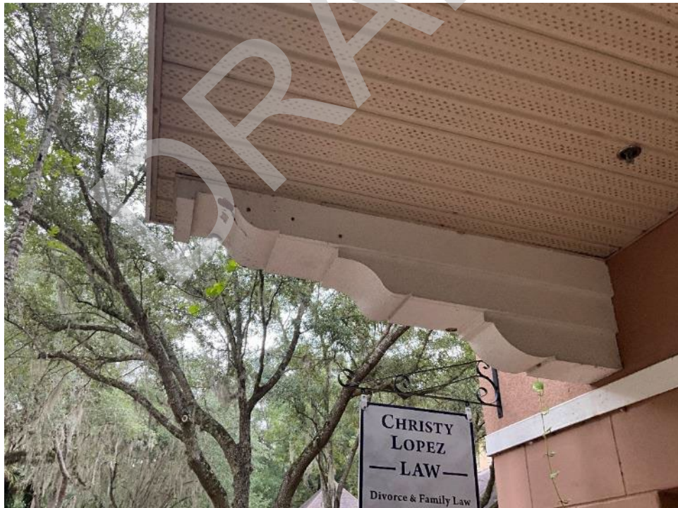
44. View of holes and cracks in the finish for the beams above unit C101.
