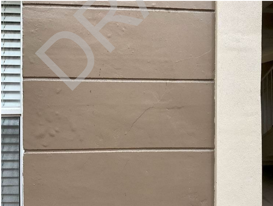
118. View of paint bubbling and finish cracks in multiple areas around the building.
