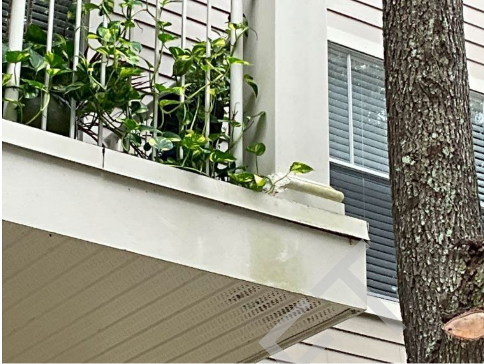
93. View of missing section of bottom of column in balcony near unit H201.
