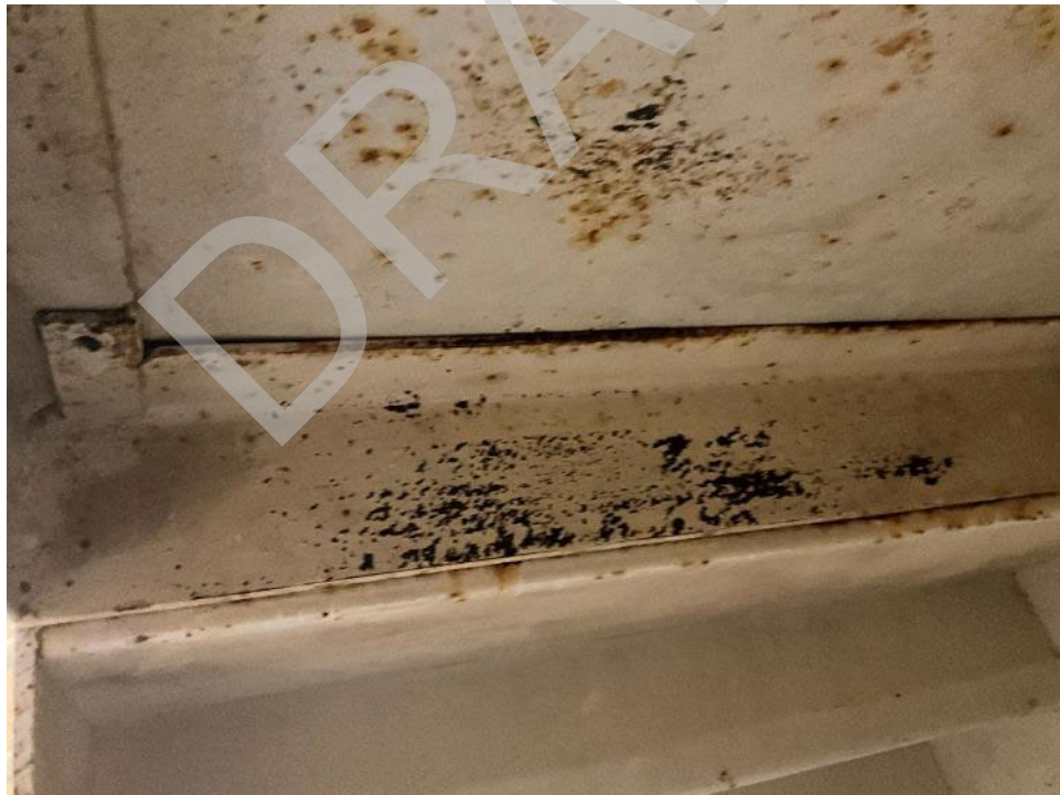
22. View of corrosion below the metal stairs.
