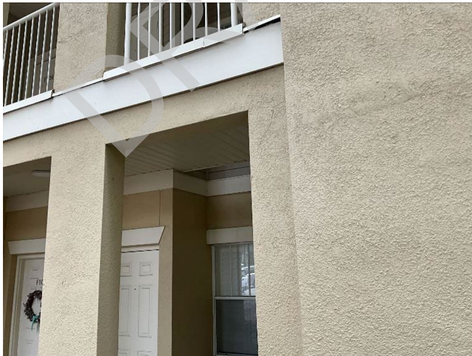
64. View of cracked section along the exterior column near F103. The stucco will need to be removed to expose the column for Phase II.
