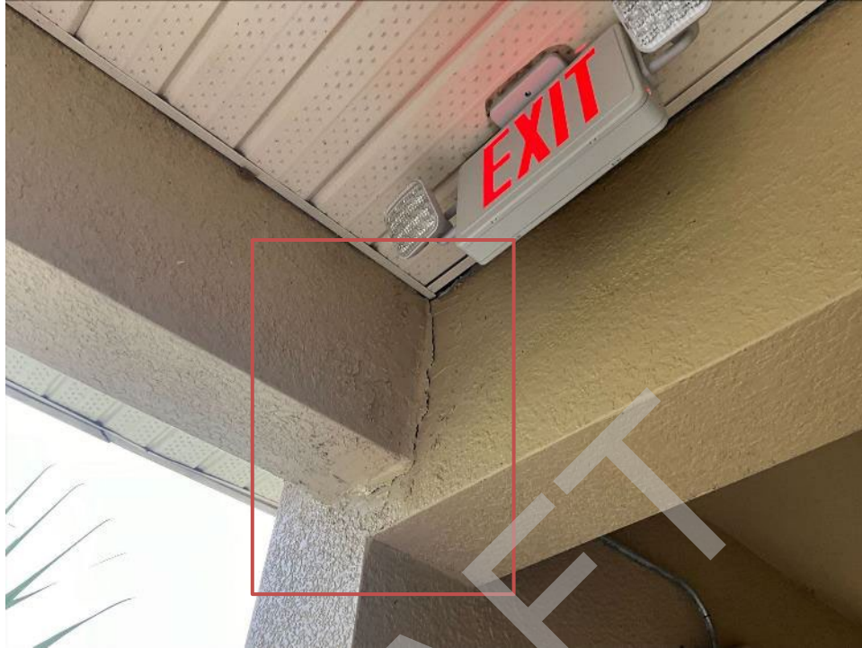
69. View of cracked section along the beam to wall interface near unit F301. The stucco will need to be removed to expose the interface for Phase II.
