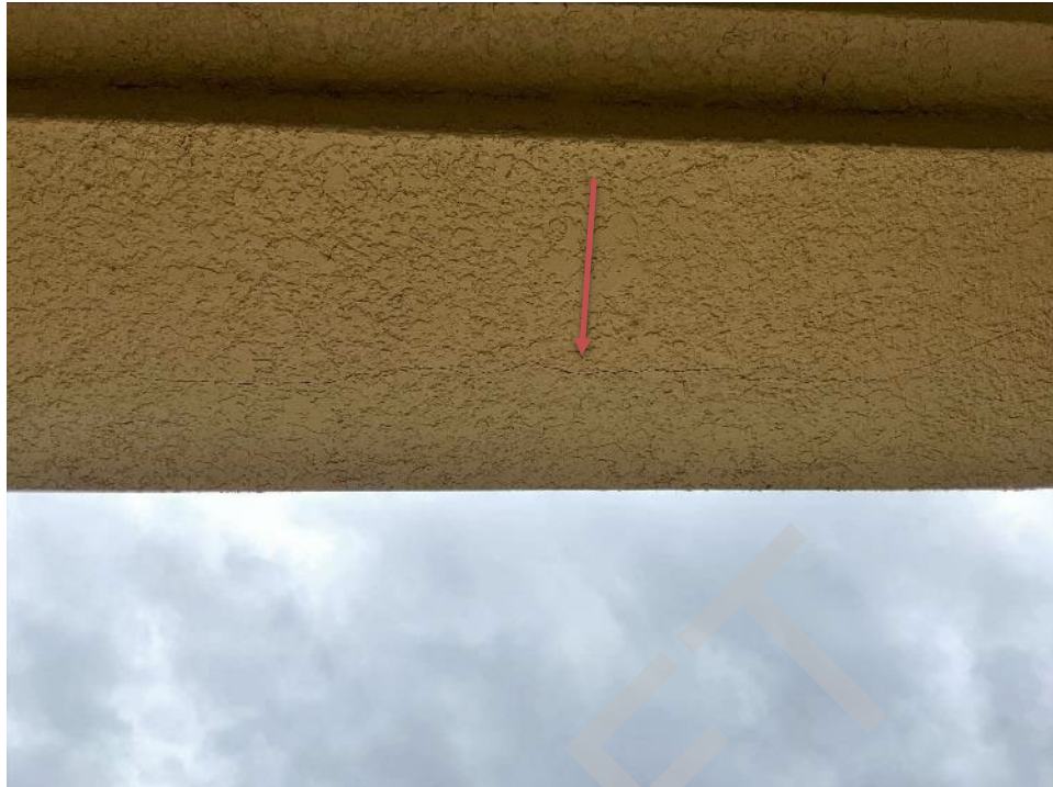
73. View of cracked section along the bottom of the beam near units G302 and G303. The stucco will need to be removed to expose the beam for Phase II.
