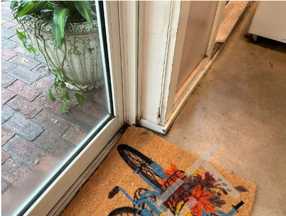
37. View of cracking along the finish around the entry door to suite B-102
