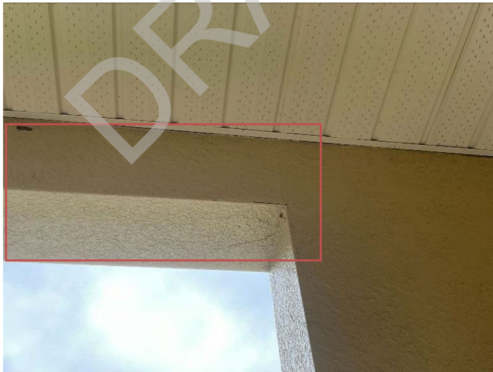
86. View of cracked section along the beam near unit H102. Cracks are observed along all faces of the beam. The stucco will need to be removed to expose the beam for Phase II.
