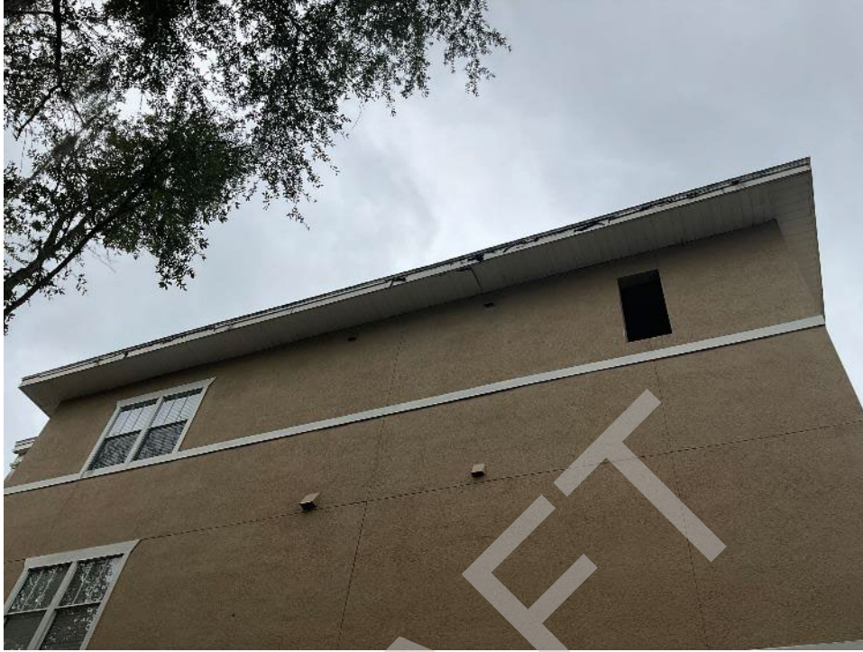
53. View of cracked section along the west elevation fascia. The fascia will need to be removed to expose the trusses for Phase II.
