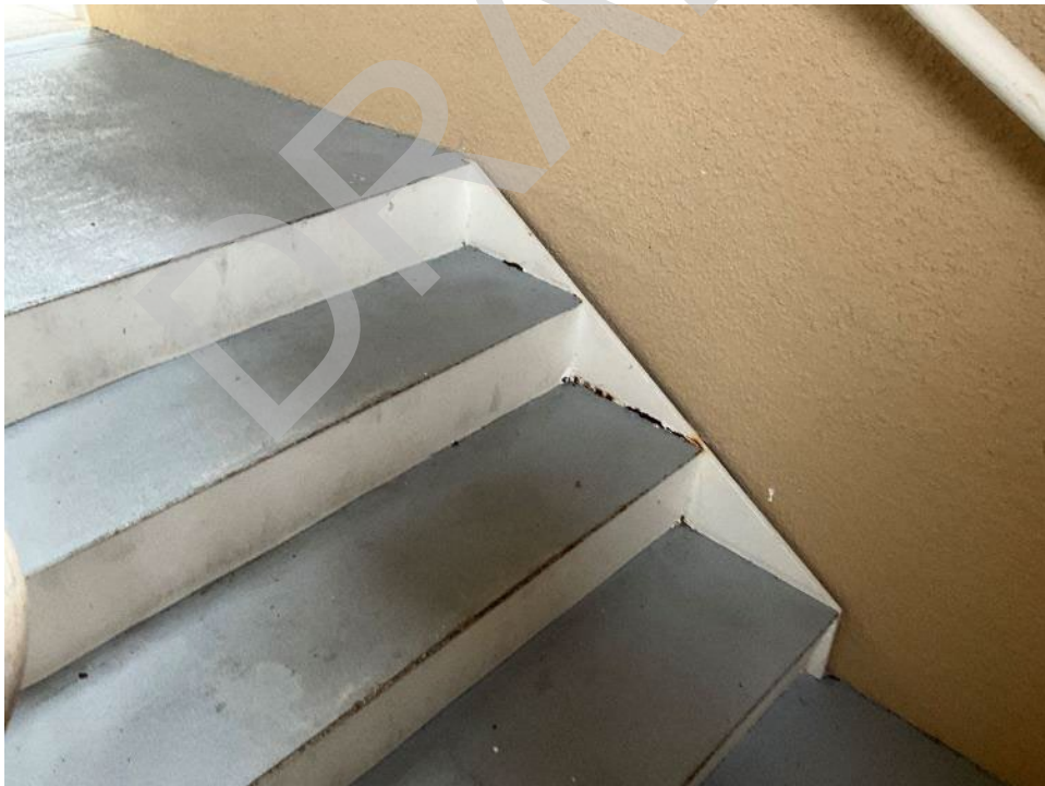
48. View of corrosion along the stairs.
