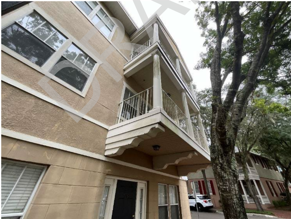
8. View of staining observed along the walls, columns, and beams of the balconies of all buildings.
