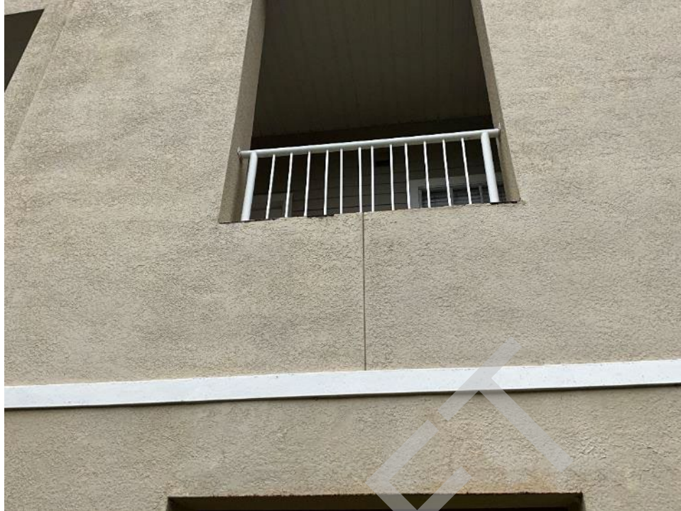
63. View of corrosion around the railing alcoves around the building.
