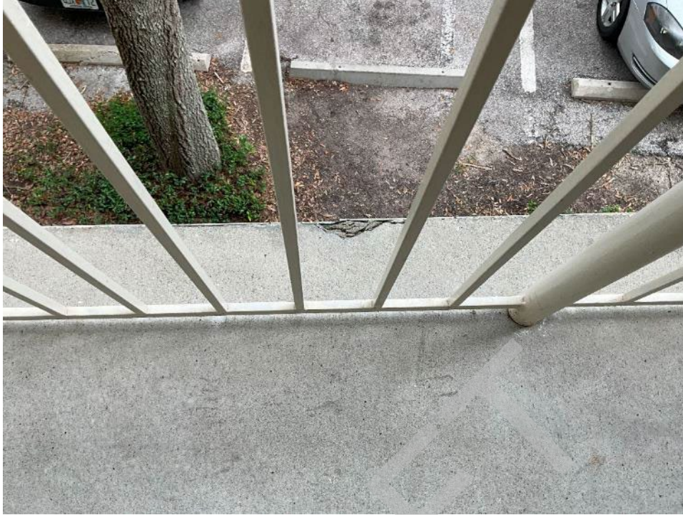
117. View of crack in the edge of the second level breezeway floor.
