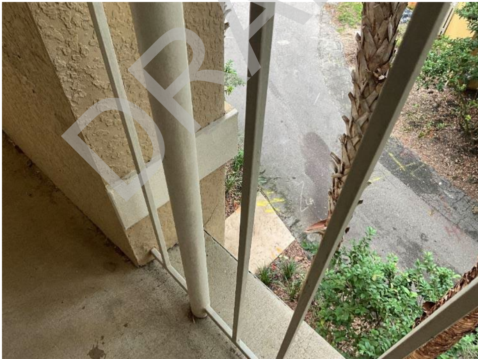
26. View of cracking in the column next to the third level breezeway.
