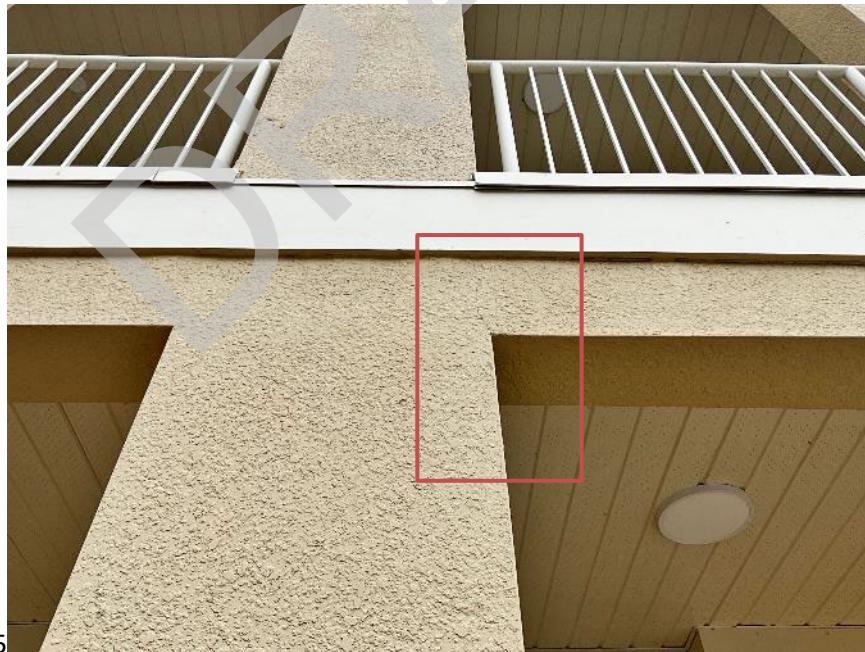
72. View of cracked section that runs along each side of the beam to column interface near units G102 and G104. The stucco will need to be removed to expose the interface for Phase II.
