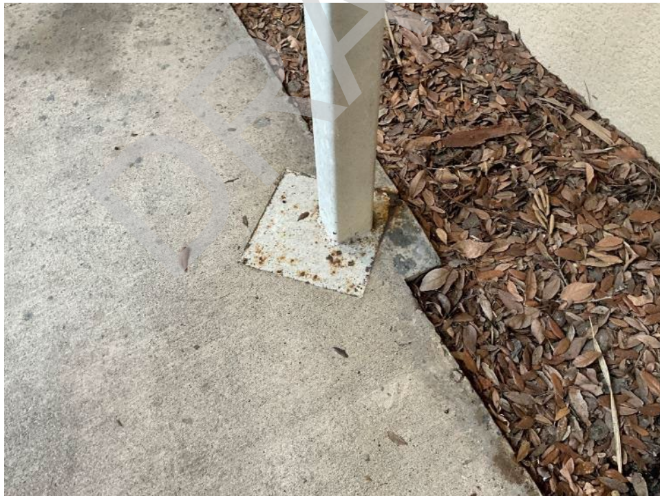
18. View of corrosion observed at the base of the metal columns along the rear of Building A.
