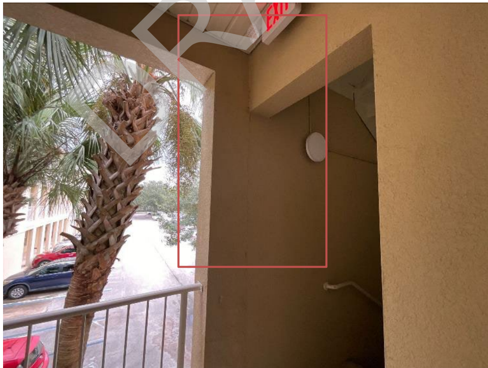
68. View of cracked section along the wall and beam near unit F201. The stucco will need to be removed to expose the interface for Phase II.
