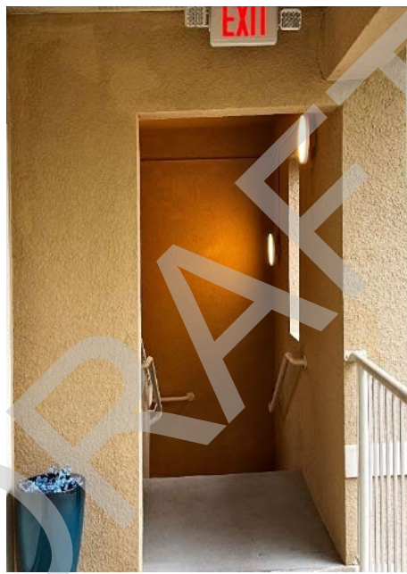
20. View of cracked section of wall next to unit A303. The paint and stucco will need to be removed to expose the wall for Phase II.
