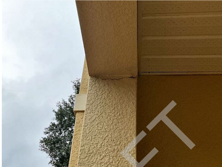
71. View of cracked section along the beam to column interface near unit G104. The stucco will need to be removed to expose the interface for Phase II.
