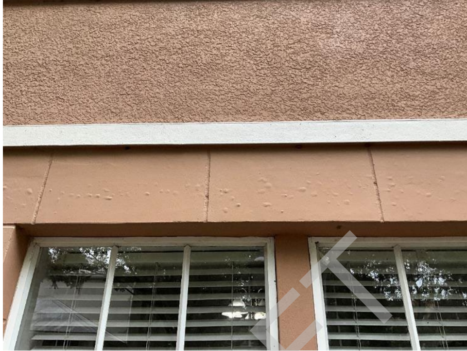
43. View of paint bubbling along all the walls.
