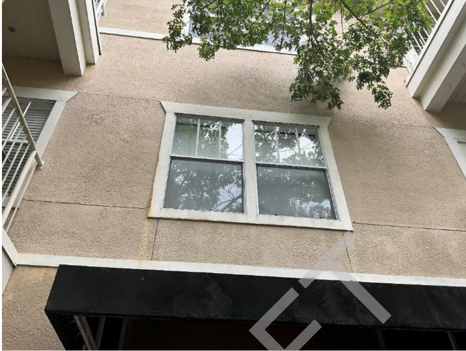
7. View of staining along the finish around the windows.
