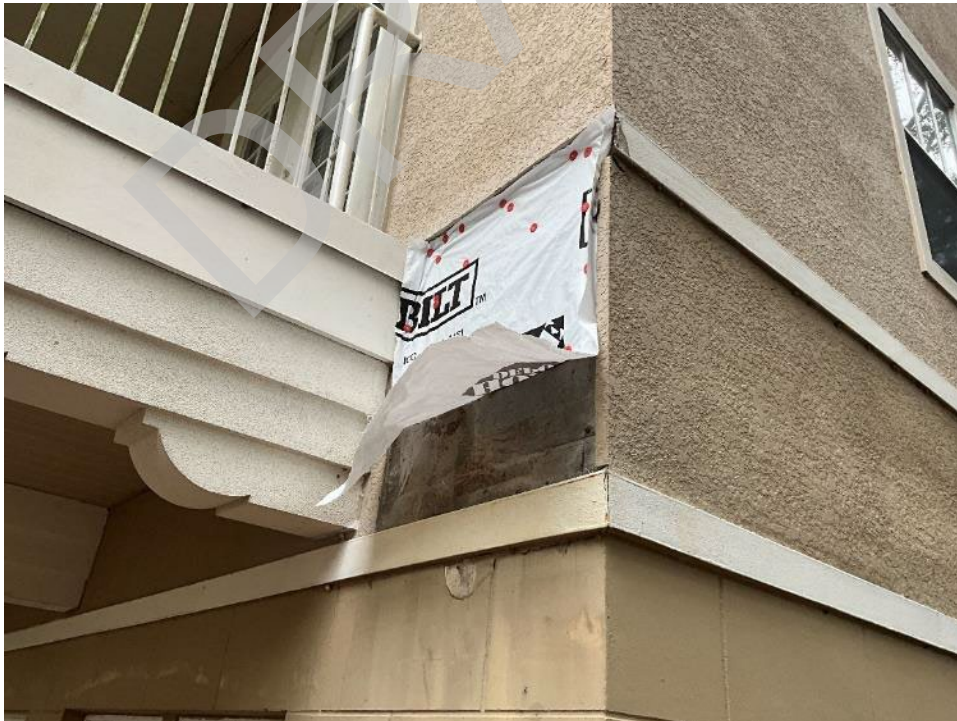
14. View of an area of Building A where stucco is unrepaired and paint delamination below.
