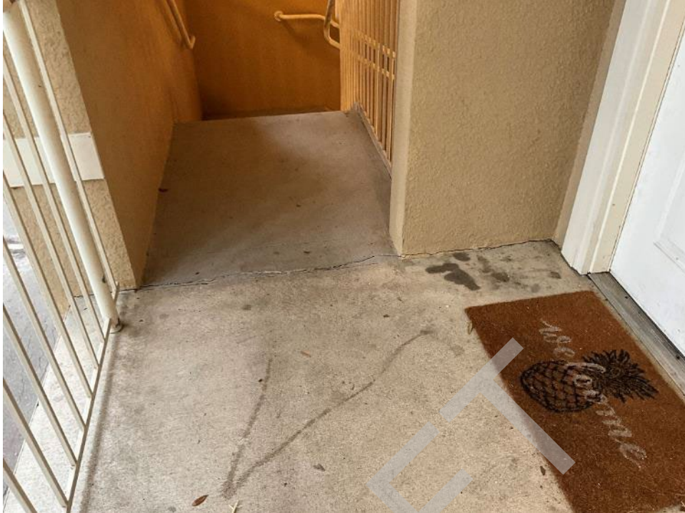
25. View of cracking along wall and breezeway slab flooring that extends through the floor slab.
