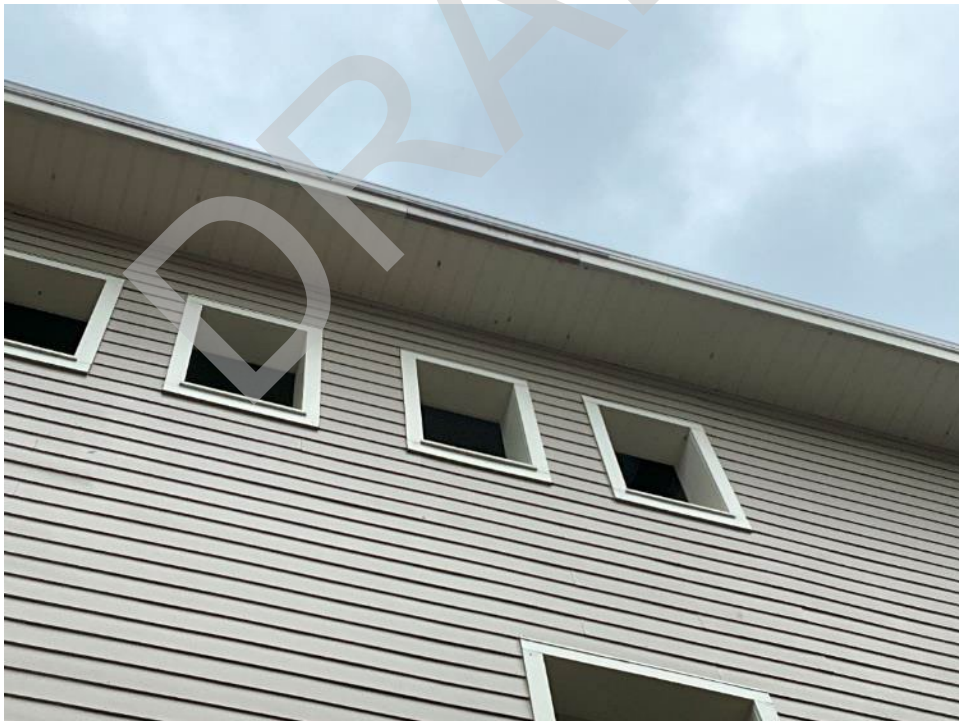
126. View of missing piece of the finish on the fascia along the east elevation.
