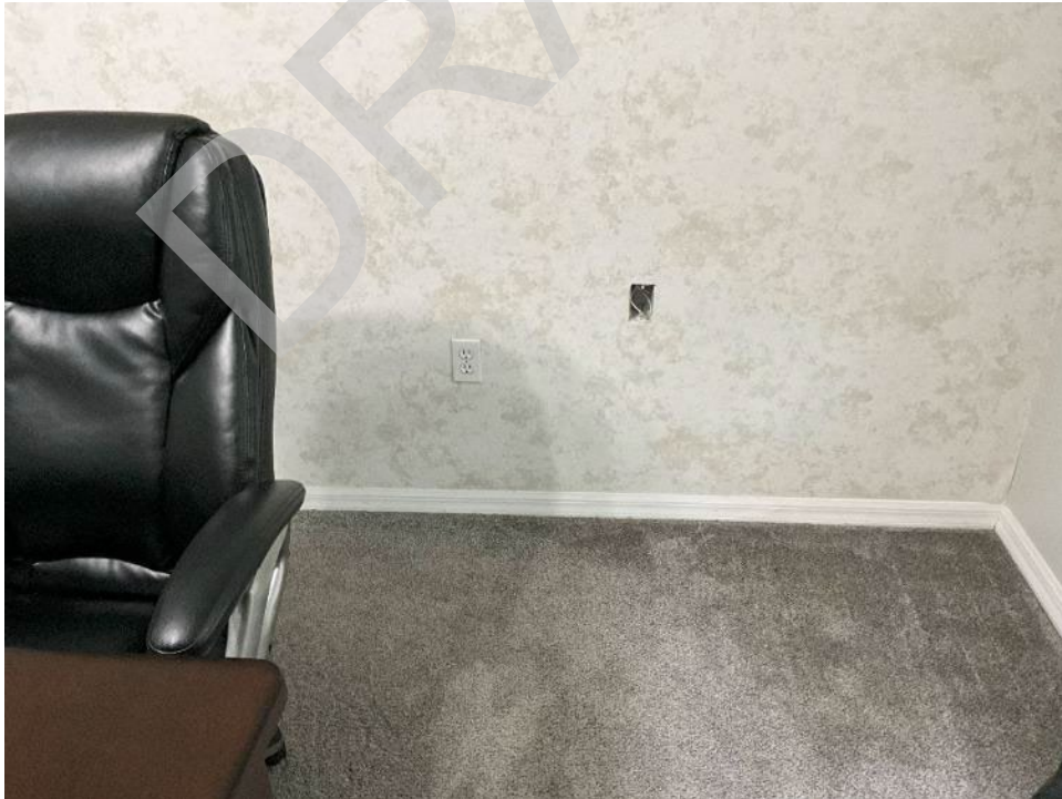
42. View of open electrical receptical in unit C101.
