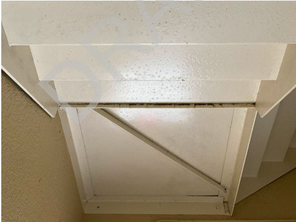
84. View of minor corrosion under the metal stairs.
