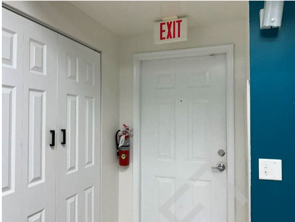
131. View of typical fire equipment around the community.
