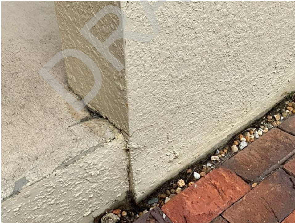
78. View of crack in bottom of the column in front of unit G104.
