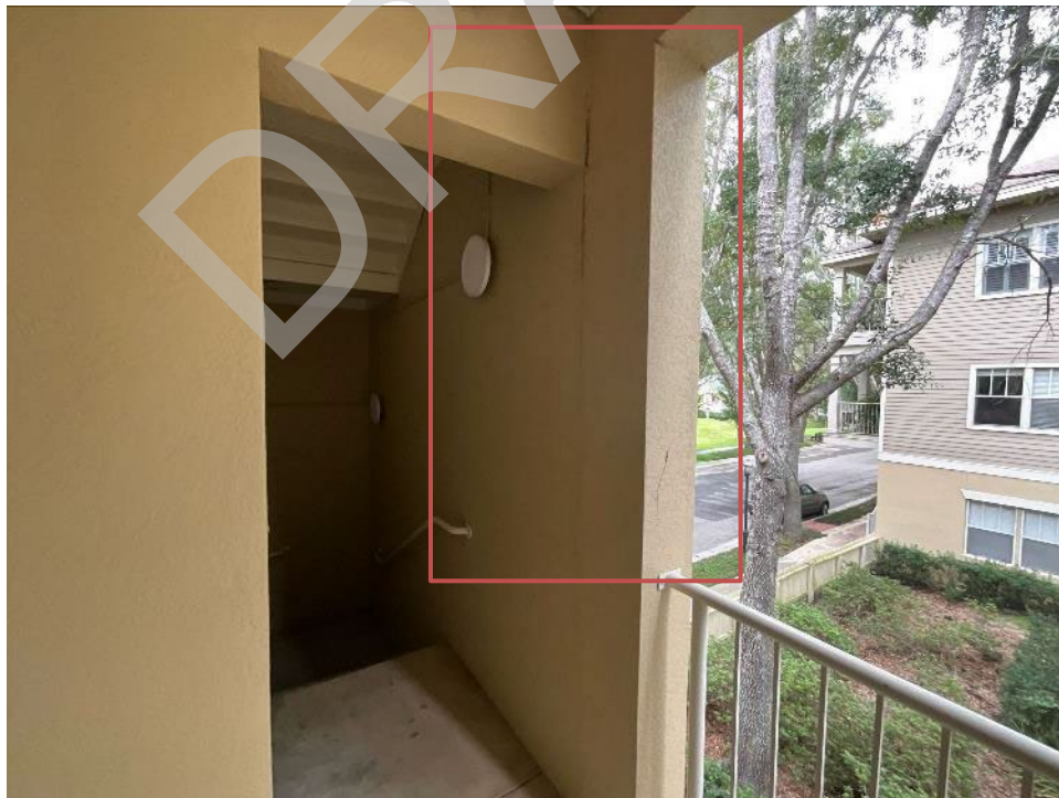
66. View of cracked section along the wall and beam near unit F203. The stucco will need to be removed to expose the interface for Phase II.
