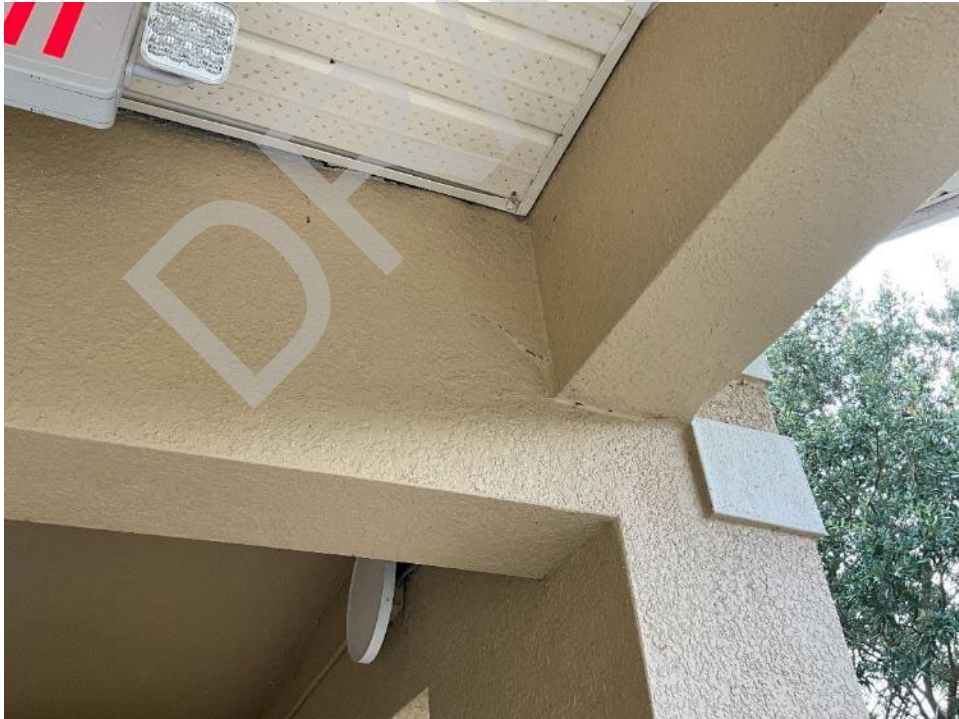
100. View of finish cracking in the beam near the stairwell and unit H301.
