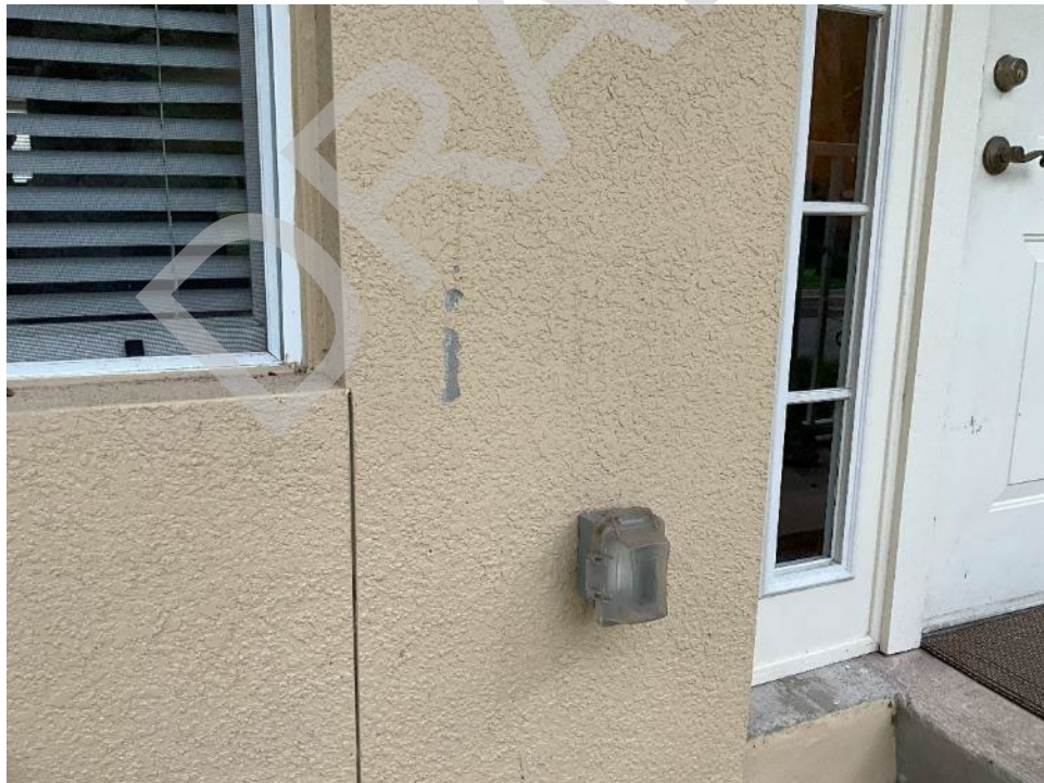
82. View of delamination on the exterior of the building.
