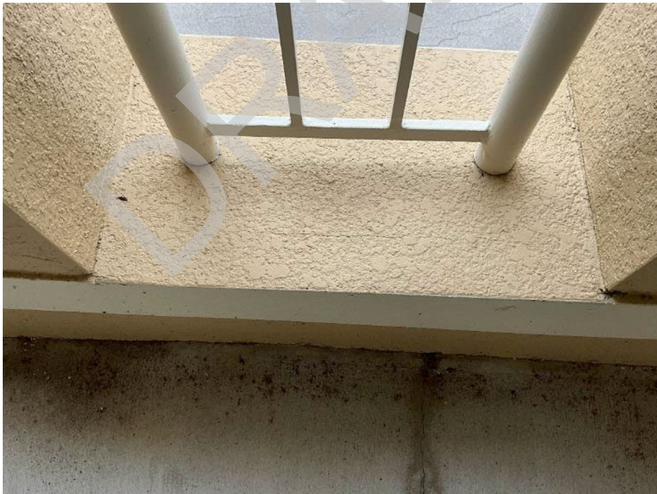
10. View of cracking underneath the railing alcoves at each building.
