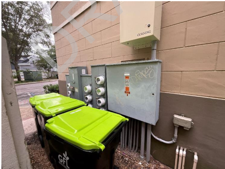
128. View of typical electrical meters.
