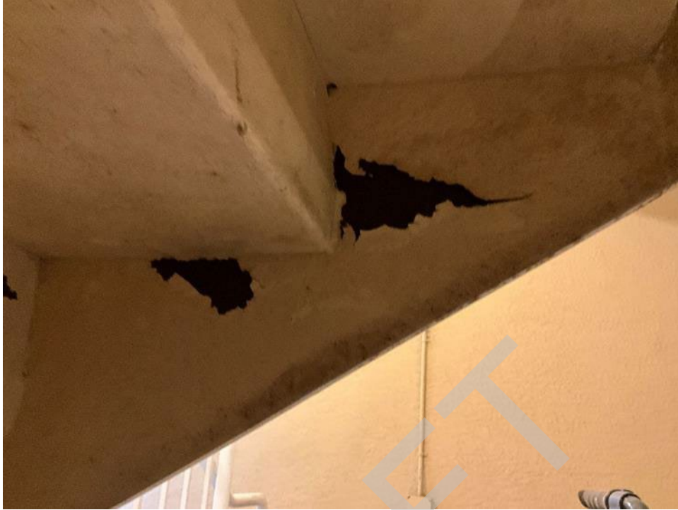
21. View of paint delamination along the stairwells.
