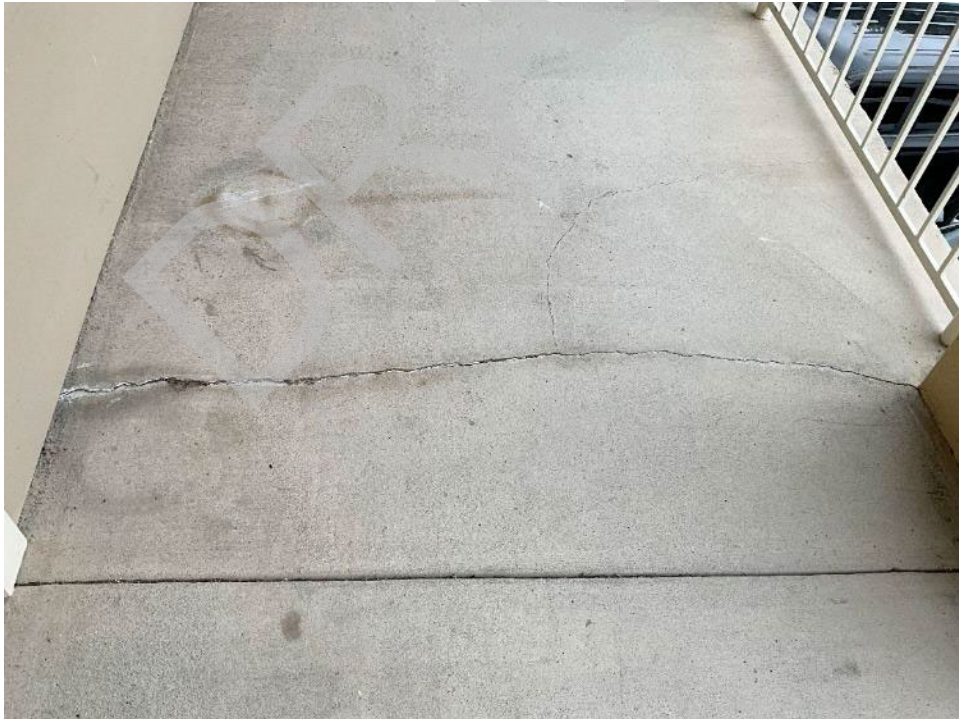
12. View of cracks in the breezeways of the building.
