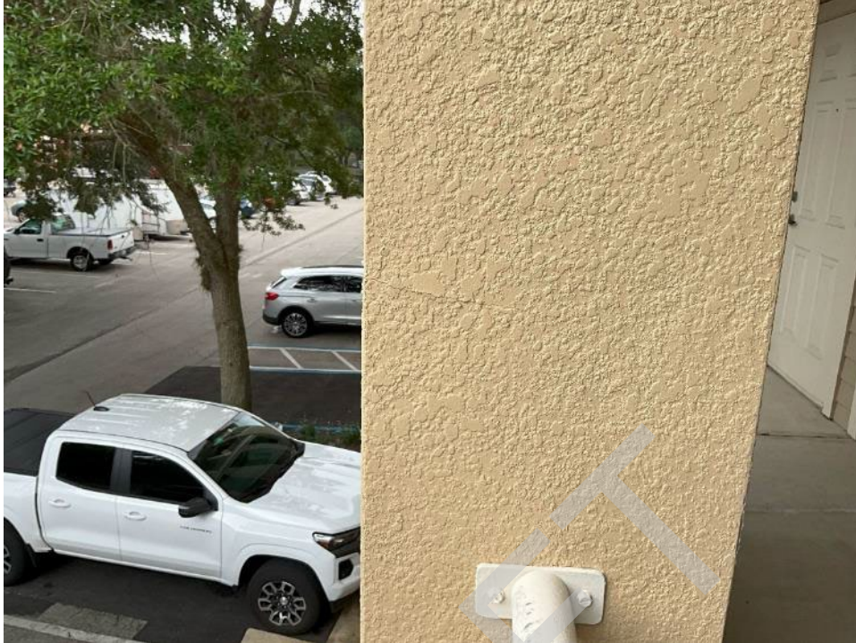
101. View of finish cracking in the column near the stairwell and unit H201.
