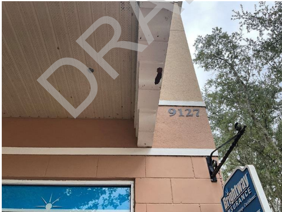
58. View of cracking and holes in the finish of the beams above unit D-103.
