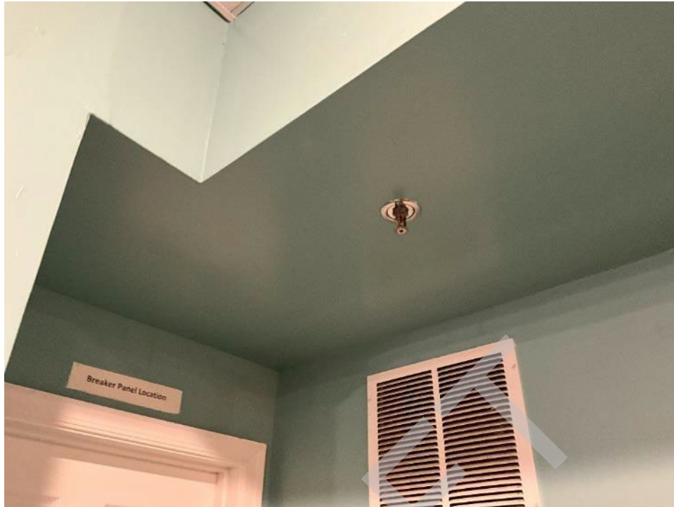
129. View of typical sprinklers through out the buildings.
