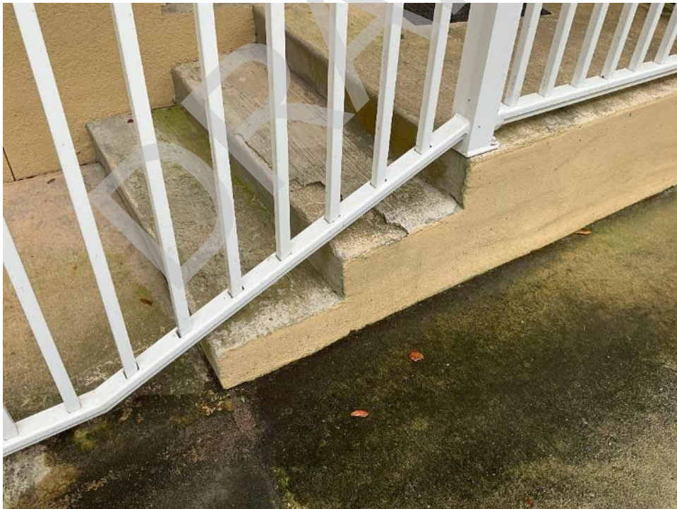
94. View of spalled section of concrete stairs.
