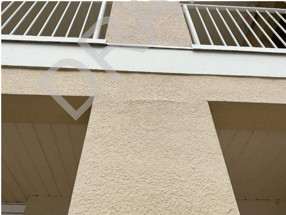
80. View of bulging on the front of a first level column.
