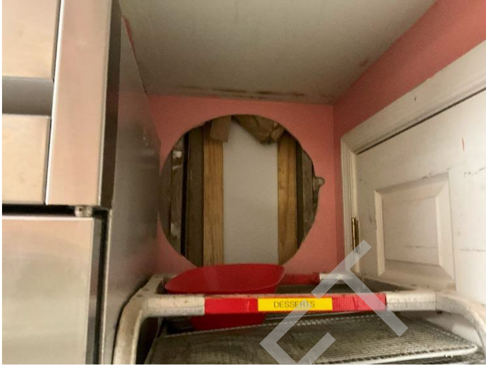
39. View of unrepaired walls in suite B-102.
