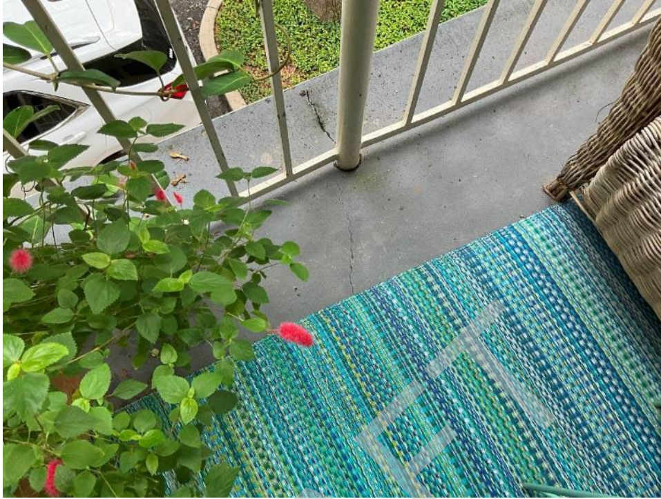
89. View of a crack in the balcony of unit H201.
