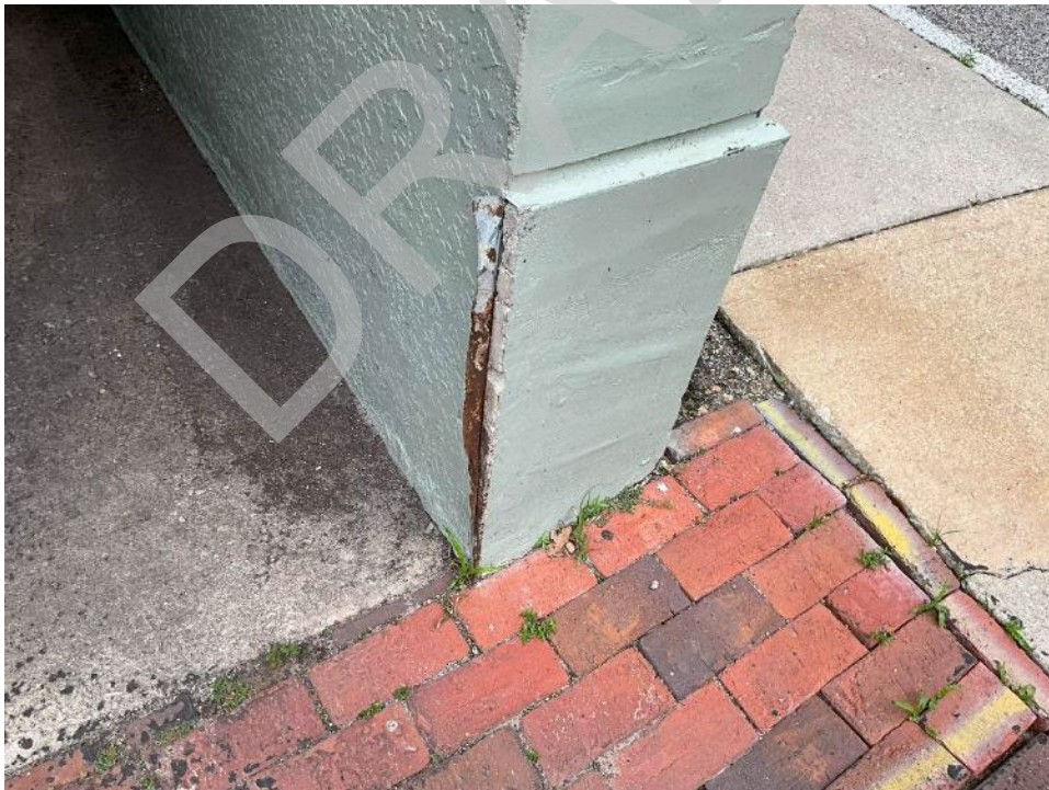
114. View of corroded edge of wall base.
