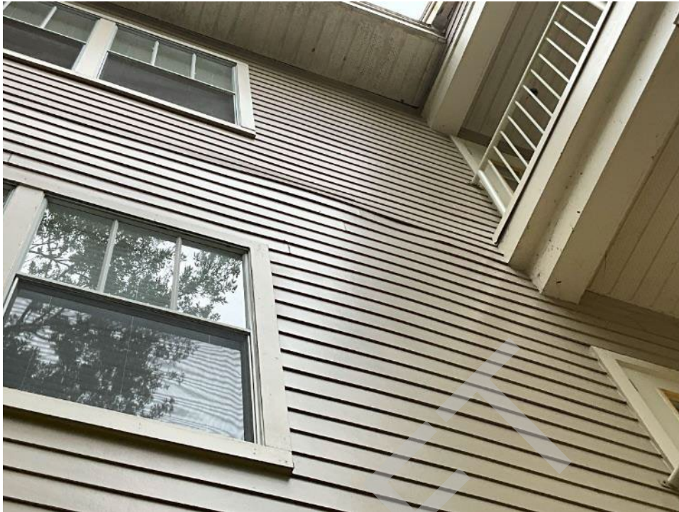
95. View of bulging in siding along the rear elevation.
