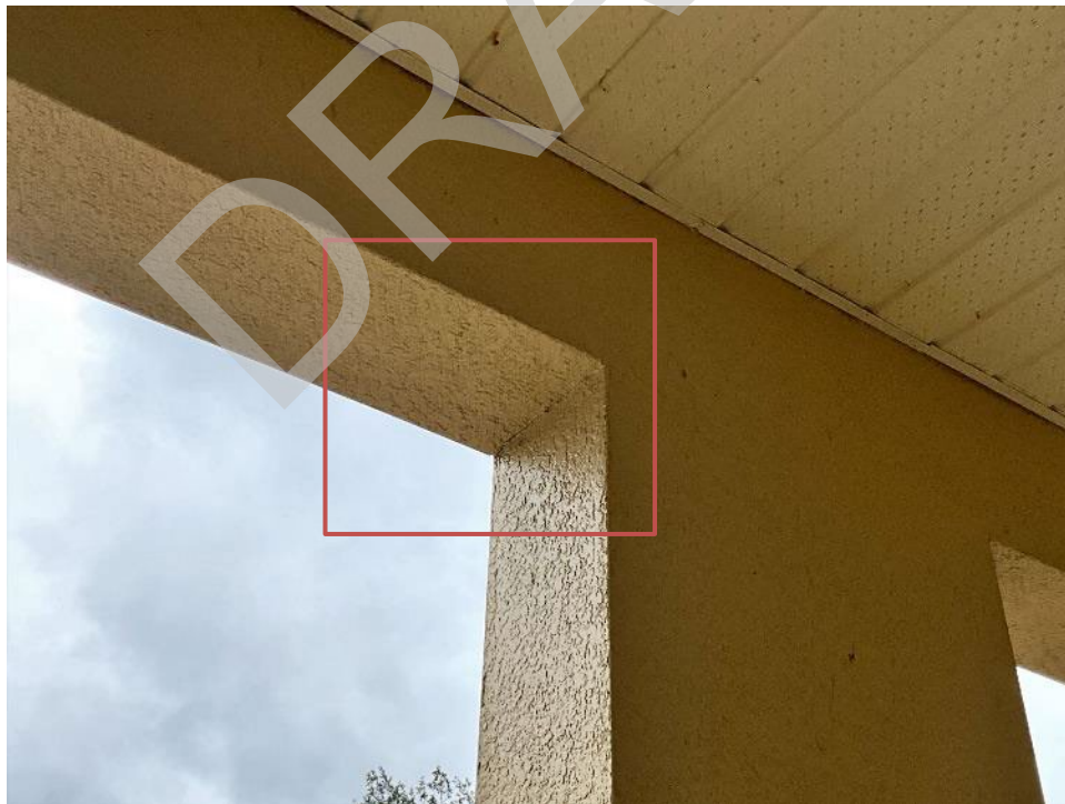
76. View of cracked section along both sides of the beam to column interface near unit G204. The stucco will need to be removed to expose the interface for Phase II.
