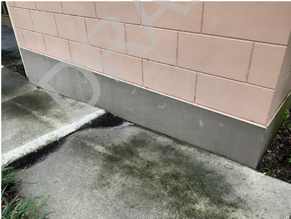
46. View of staining and cracking around the foundation of the building.
