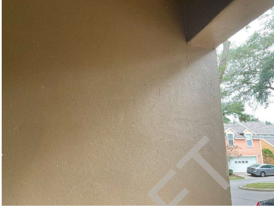
127. View of crack in the finish along the interior breezeway.
