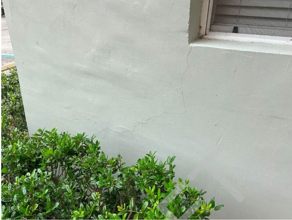
109. View of crack running from the corner of the window to the bottom of the wall.
