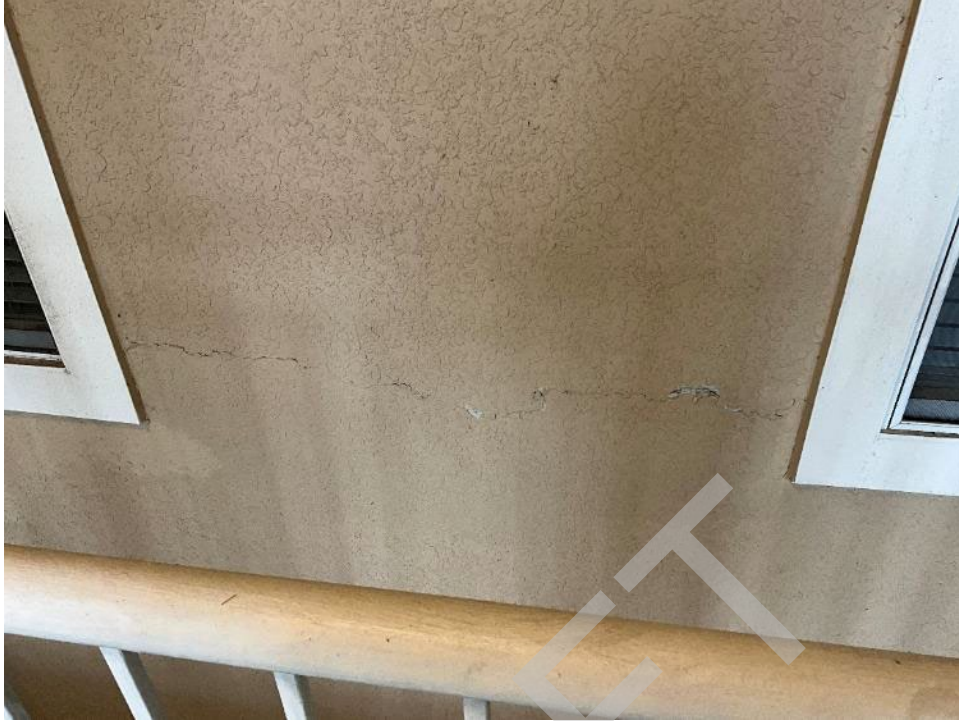
23. View of horizontal cracking between windows on the second level.
