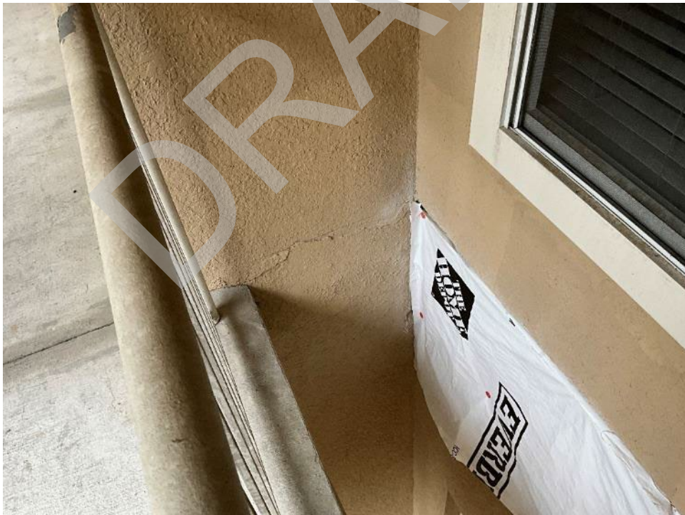
24. View of horizontal cracking between the breezeway slab and the wall.
