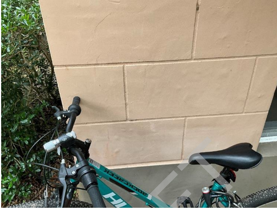
45. View of stair-step cracks in the wall finish.
