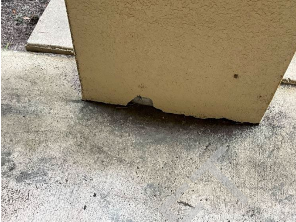
91. View of missing section of stucco at the bottom of a column near unit H104.
