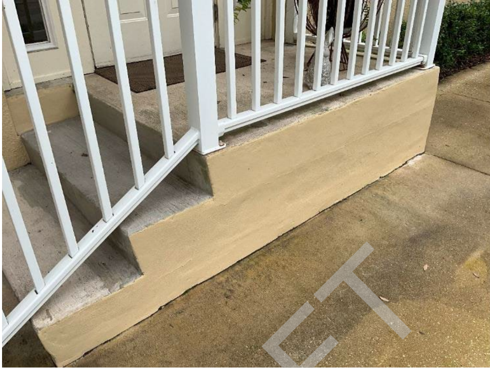
83. View of bulging along the stairs leading to unit G102.
