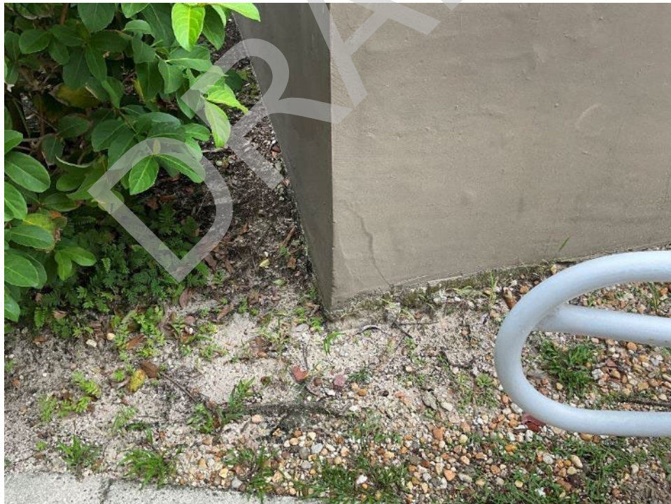
60. View of cracking at a corner of the building.
