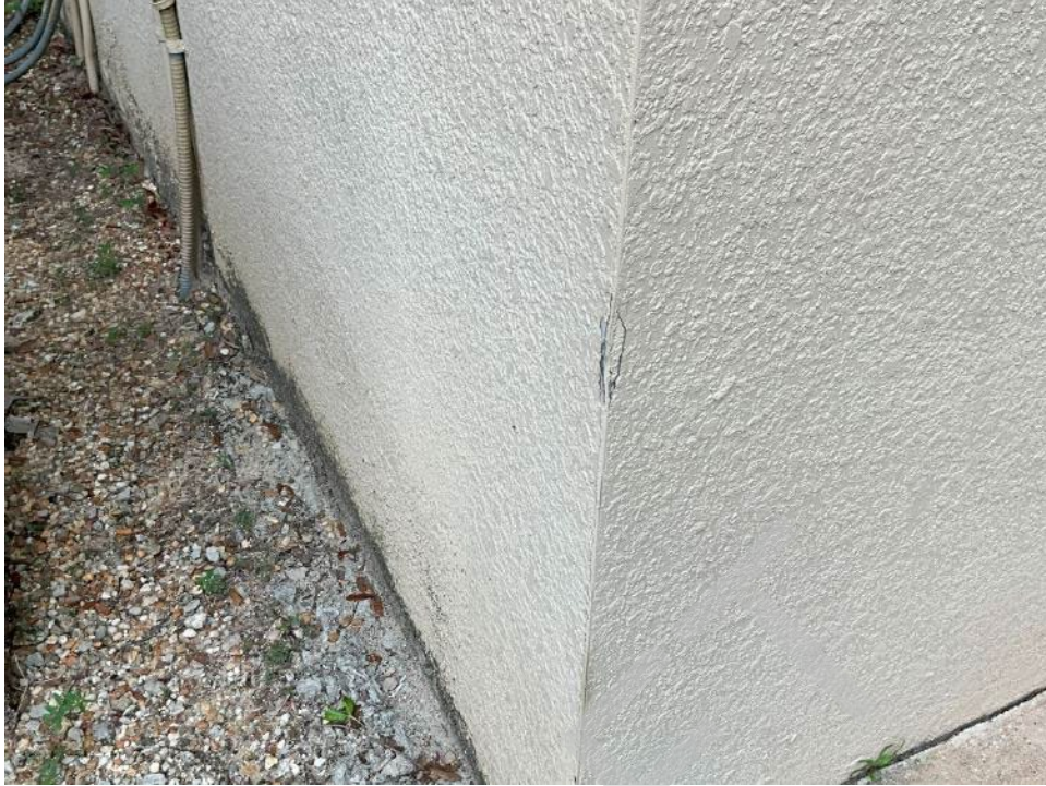
97. View of spalling at the corner of the building.
