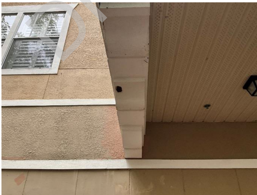
28. View of spalling in decorative beam below balcony above unit B101.
