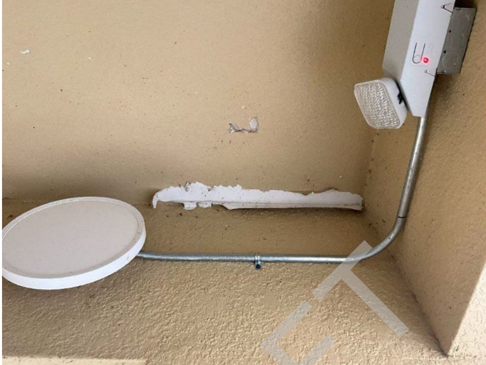
13. View of paint delamination along the ceiling of the stairwells.
