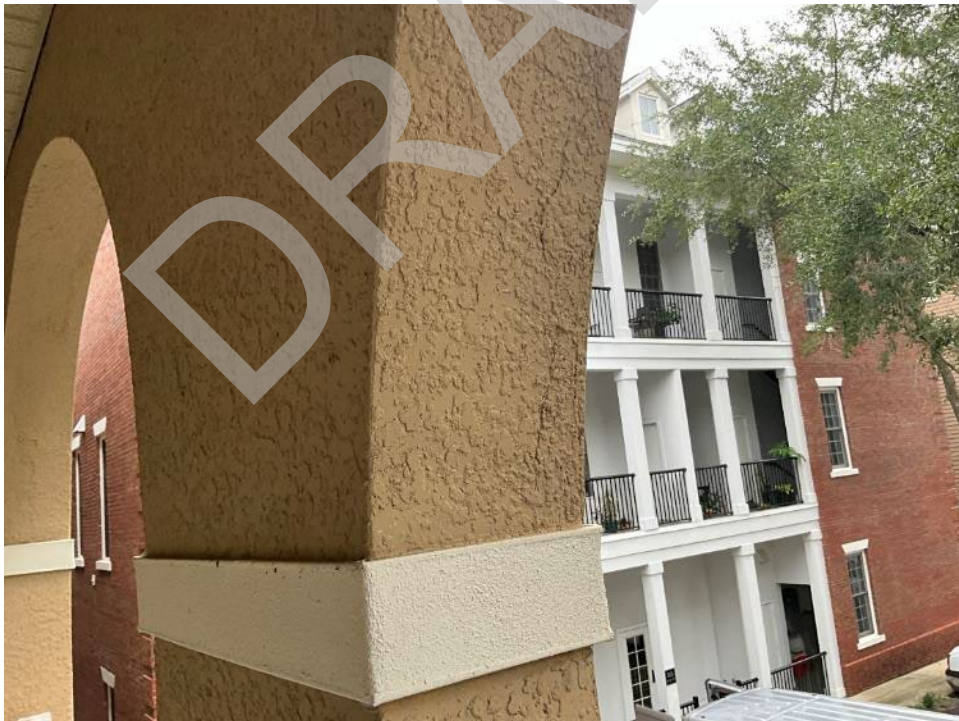
34. View of finish cracking along column near unit B201.
