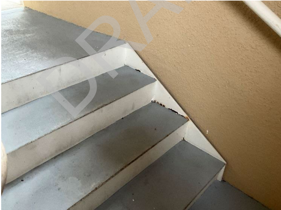
48. View of corrosion along the stairs.
