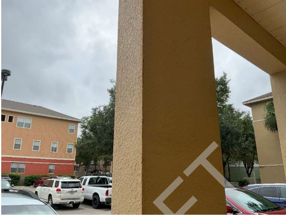
79. View of corrosion in the corner of a column on the first level.
