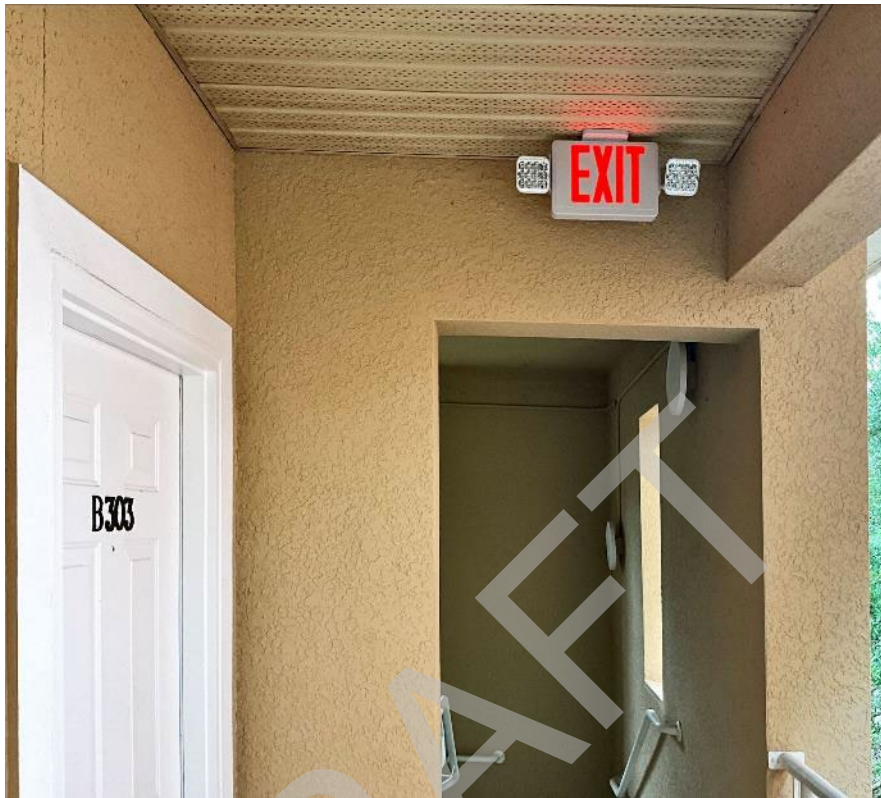
27. View of cracked section of wall next to unit B303. The paint and stucco will need to be removed to expose the wall for Phase II.
