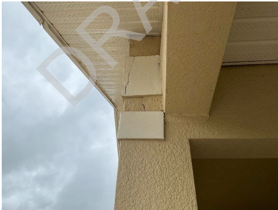
74. View of cracked sections along the beam and wall near unit G304. The stucco will need to be removed to expose this area for Phase II.
