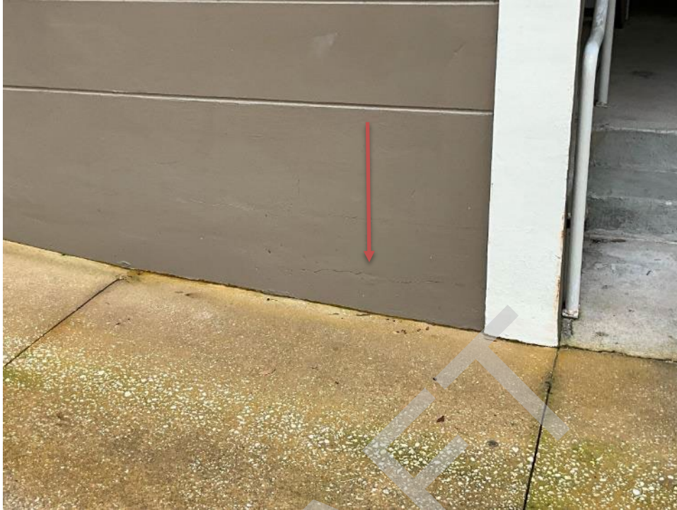
123. View of horizontal crack at the base of the wall next to the opening on the west elevation.
