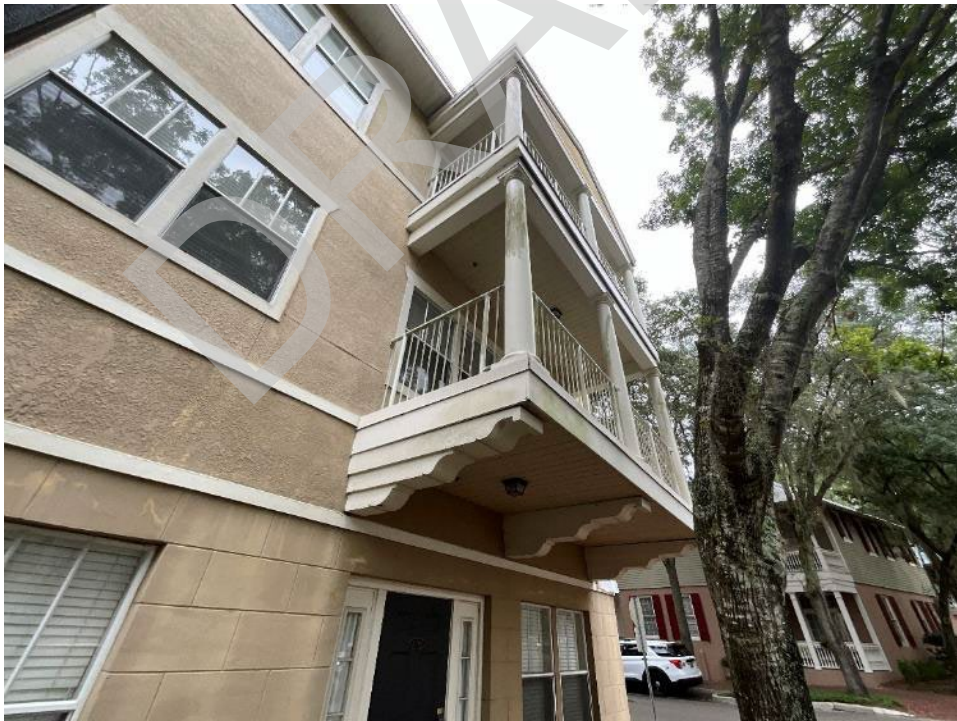
8. View of staining observed along the walls, columns, and beams of the balconies of all buildings.
