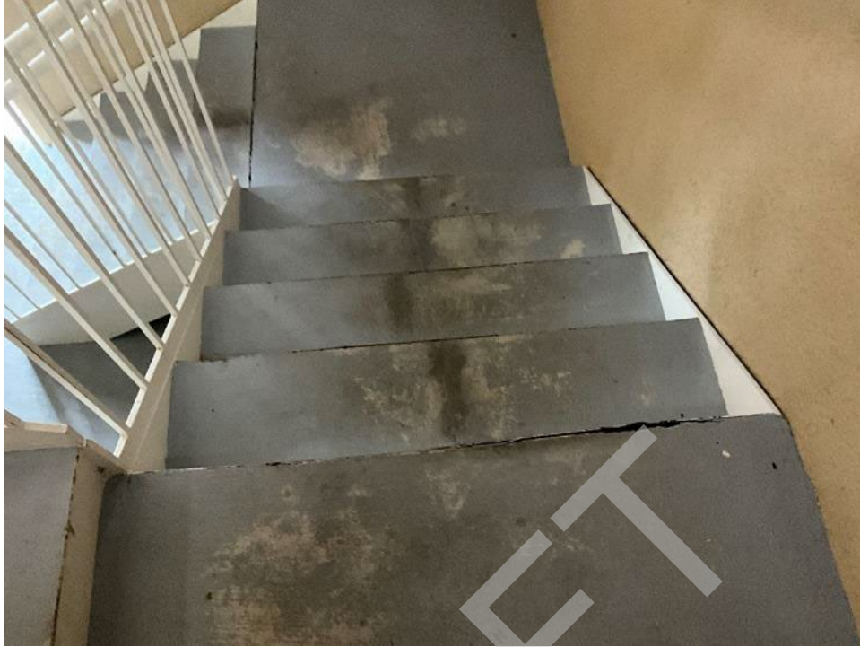
49. View of paint delamination along the stairs.
