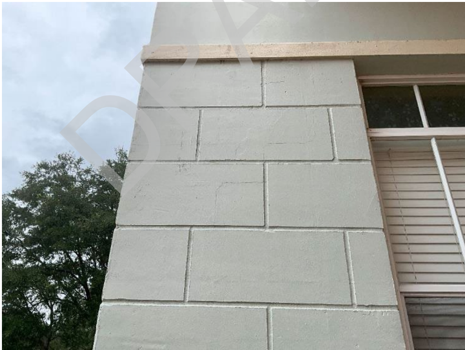
110. View of stair-step crack in the wall near the window.
