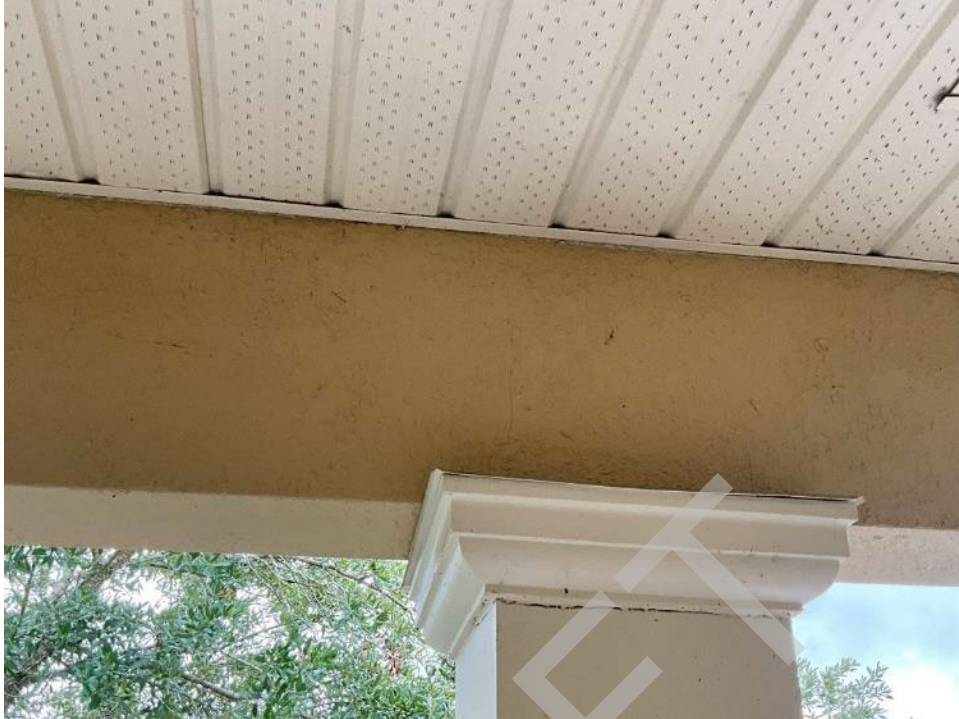
99. View of cracks in the interface of the column top and the column.
