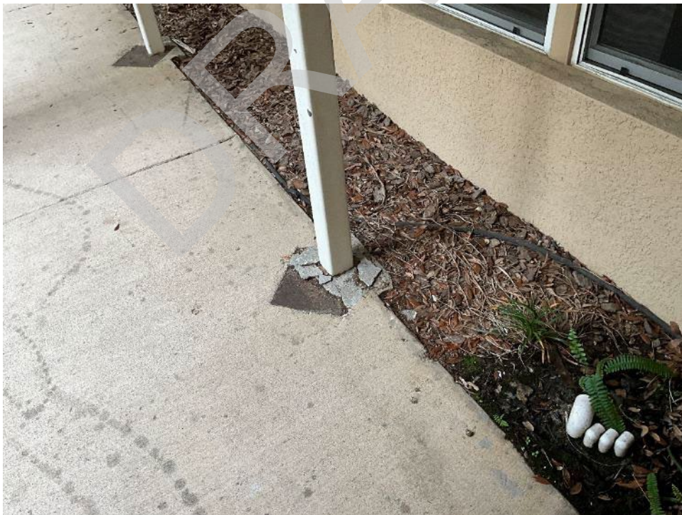
30. View of spalled concrete above steel column base plate at rear elevation.
