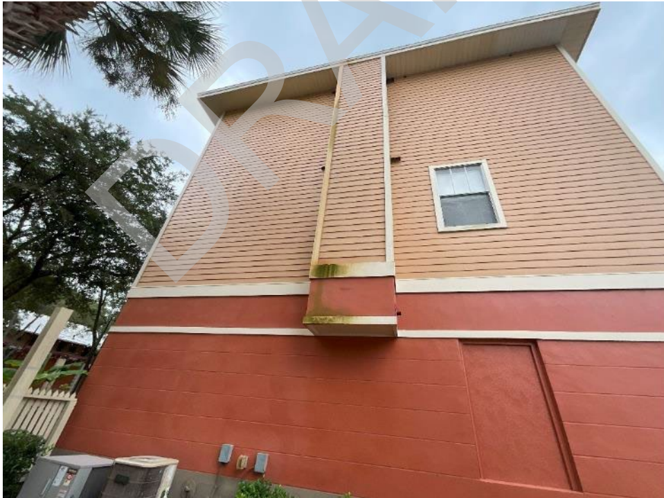
104. View of staining along a ventilation stack.
