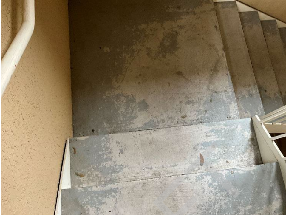
35. View of delamination on the concrete topping along the stairs.
