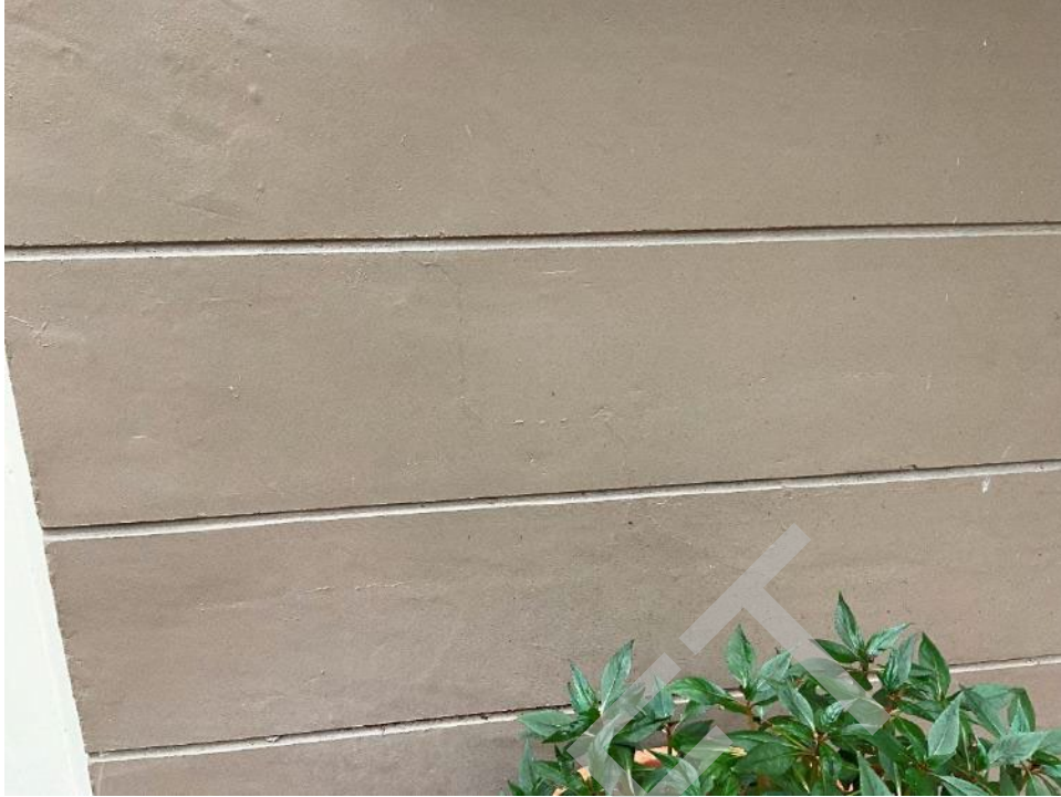
119. View of stair-step crack observed in multiple areas around the building.
