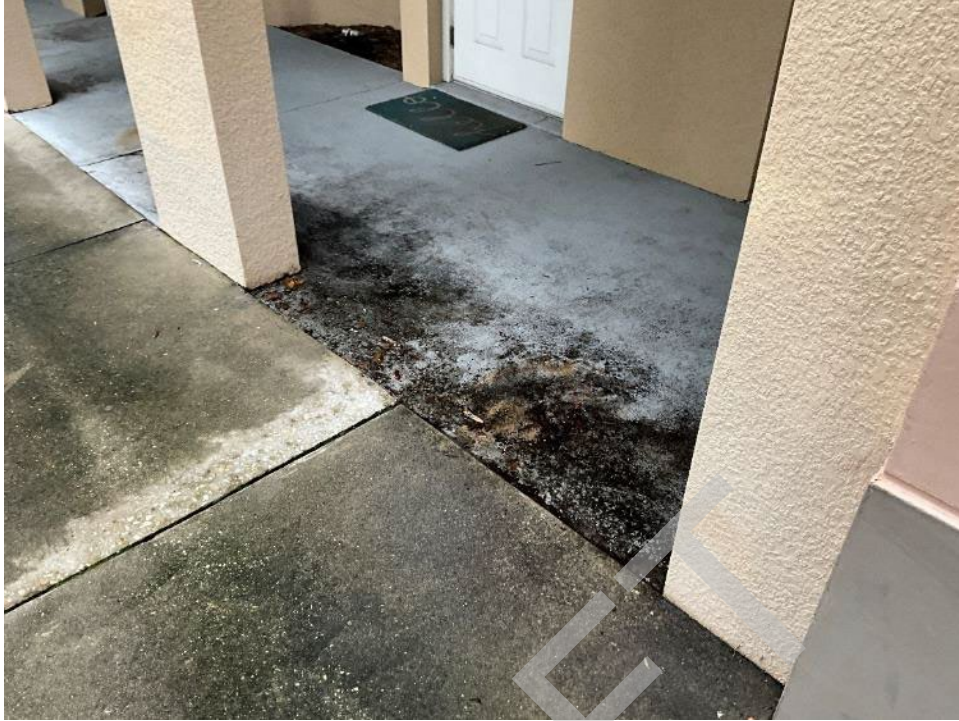
47. View of major staining along the first level slab.
