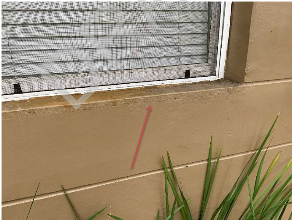
124. View of cracking under a window-sill.
