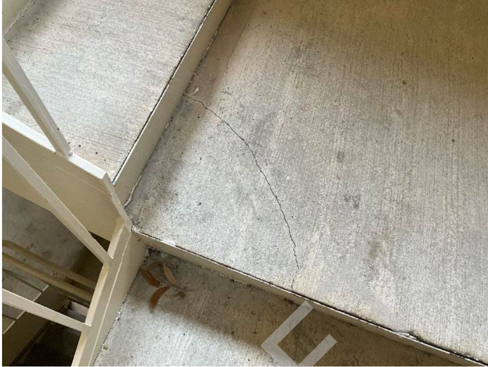
11. View of cracking in the concrete topping in the stairwells.
