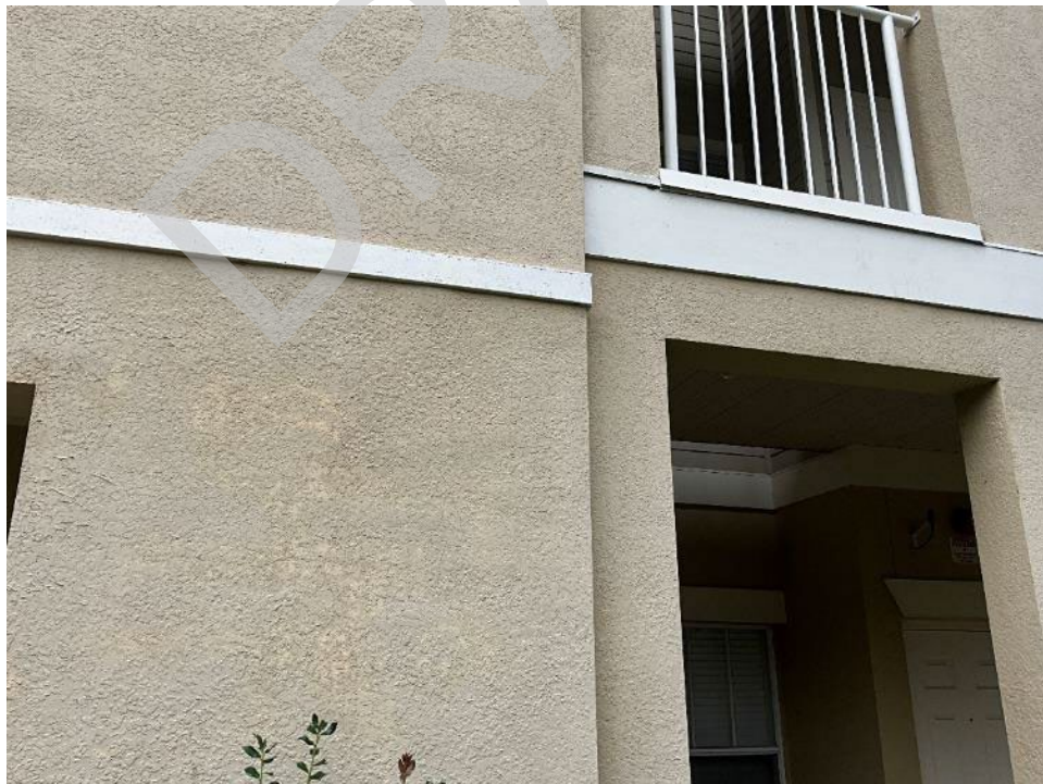
62. View of paint delamination along the walls around the building.
