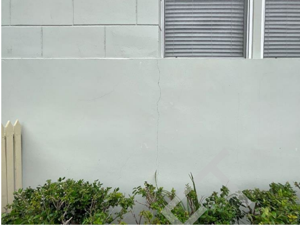
111. View of vertical cracking observed around the base of the wall.
