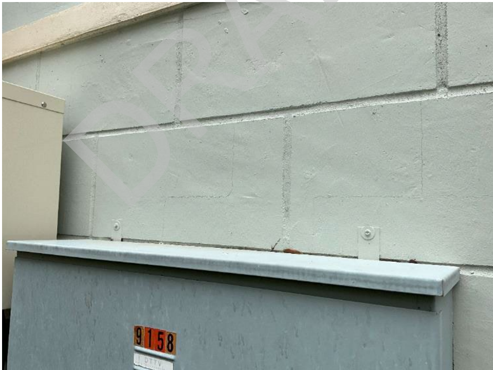
116. View of stair-step cracks along north wall.
