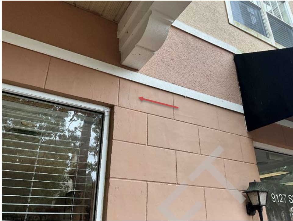
57. View of minor vertical crack in the wall near the window to unit D-102.
