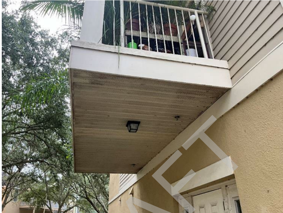
61. View of staining under the balconies.
