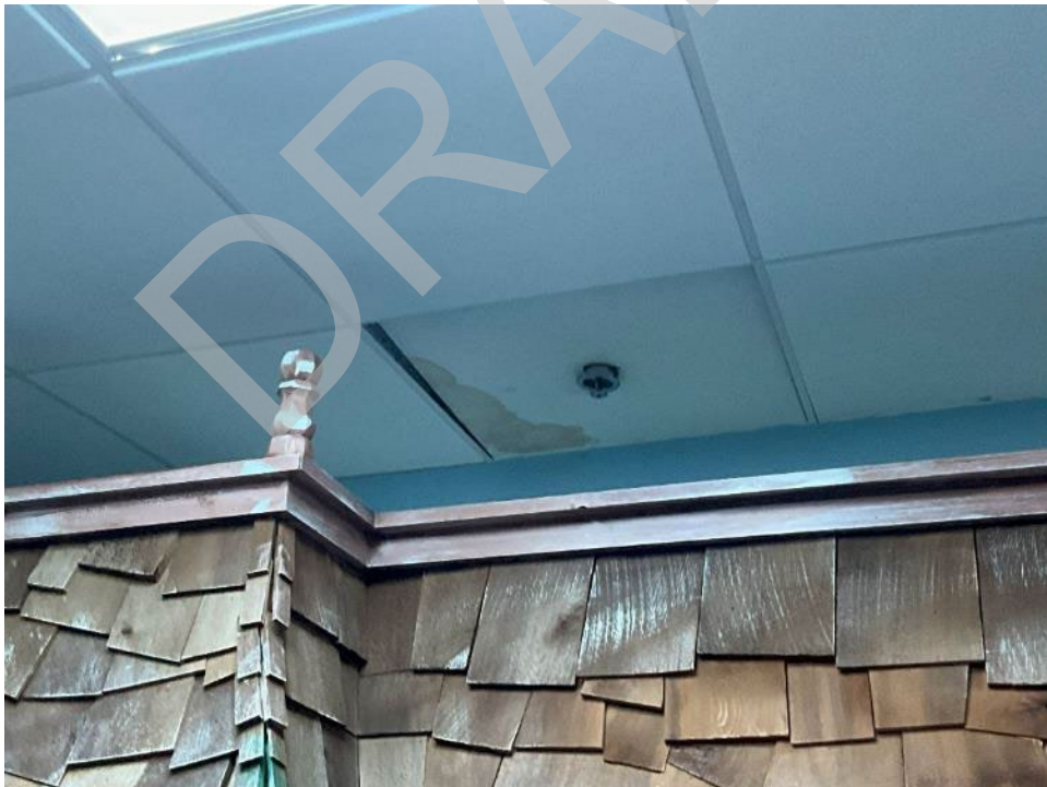
40. View of water intrusion along a ceiling panel in suite B-103.
