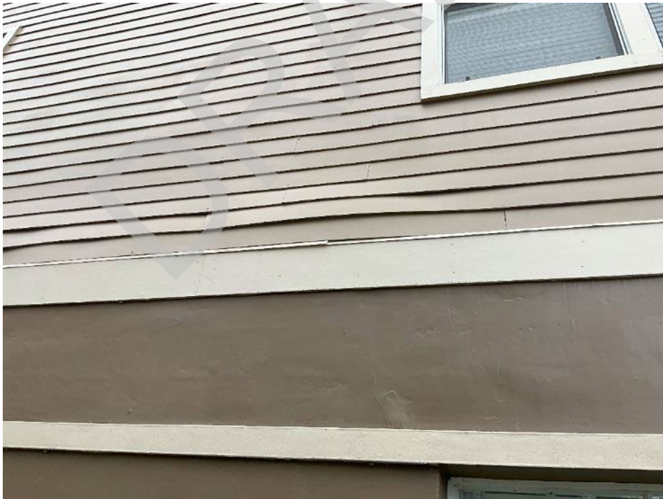
120. View of bulging under the siding around the building.
