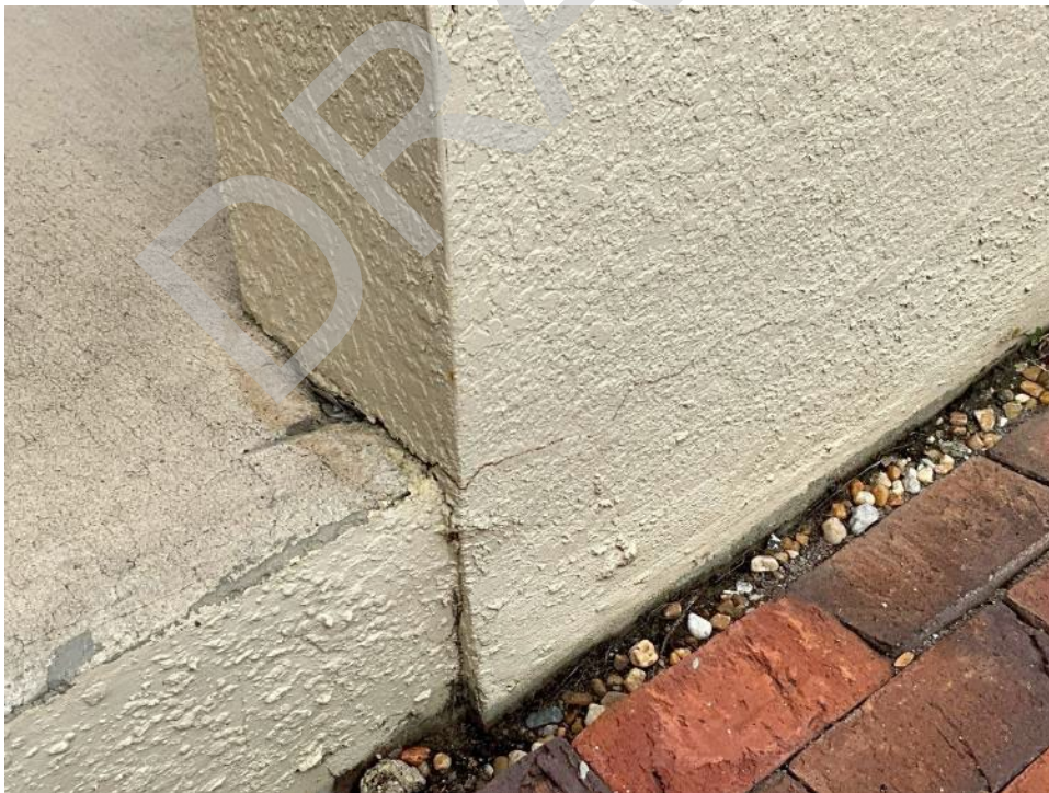
78. View of crack in bottom of the column in front of unit G104.
