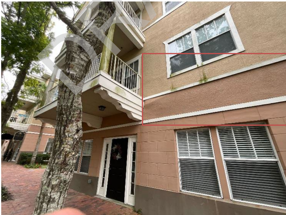
52. View of cracked section of wall next to unit D201 balcony. The paint and stucco will need to be removed to expose the wall for Phase II.
