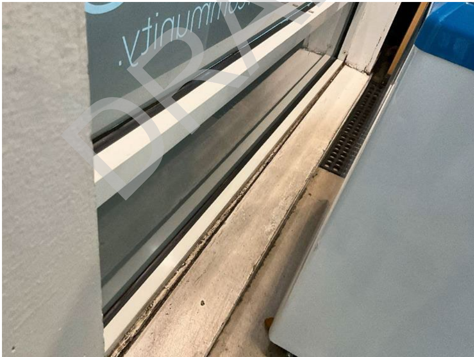
38. View of cracking along the interface between the window and the sill in suite B-102.
