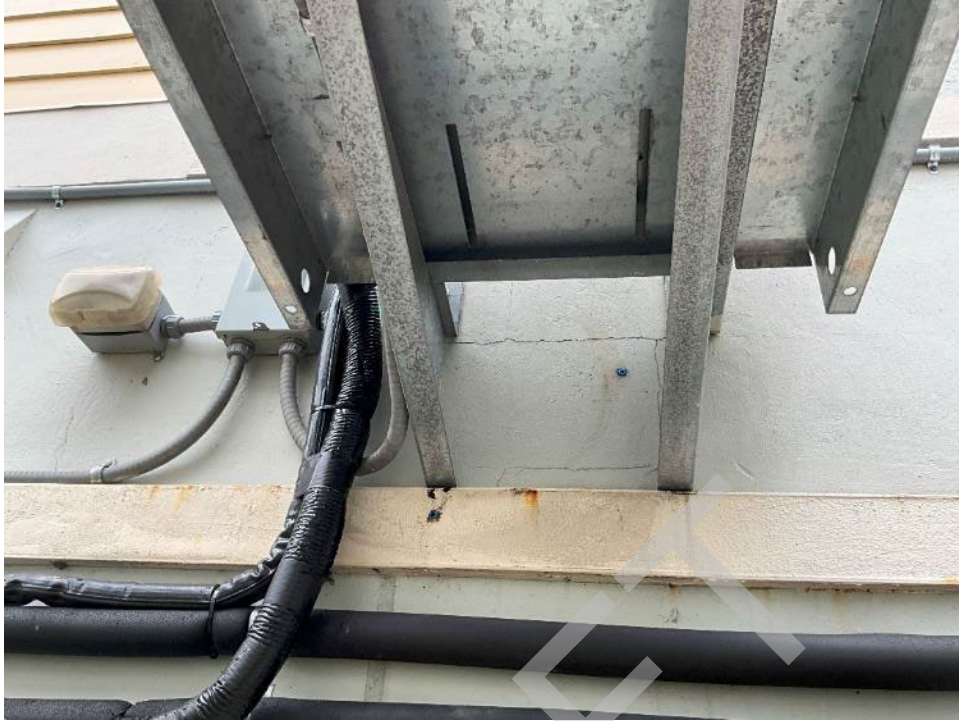
115. View of cracked wall behind AC stand.
