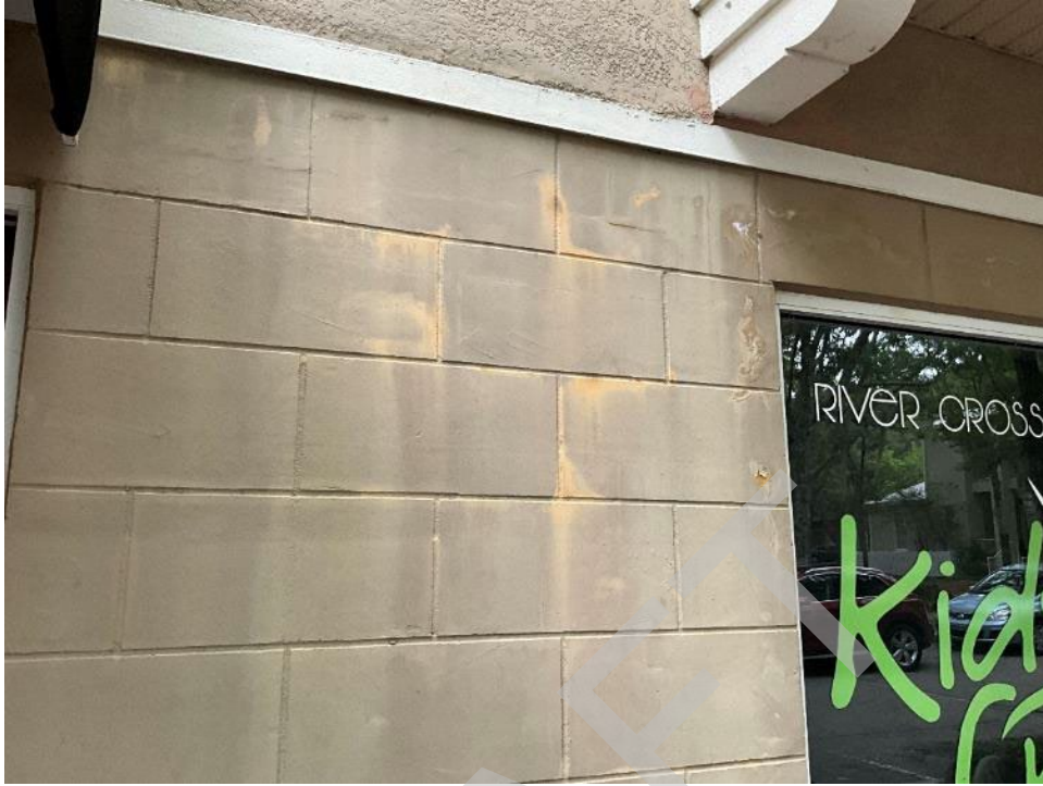
29. View of staining along the walls of the building.
