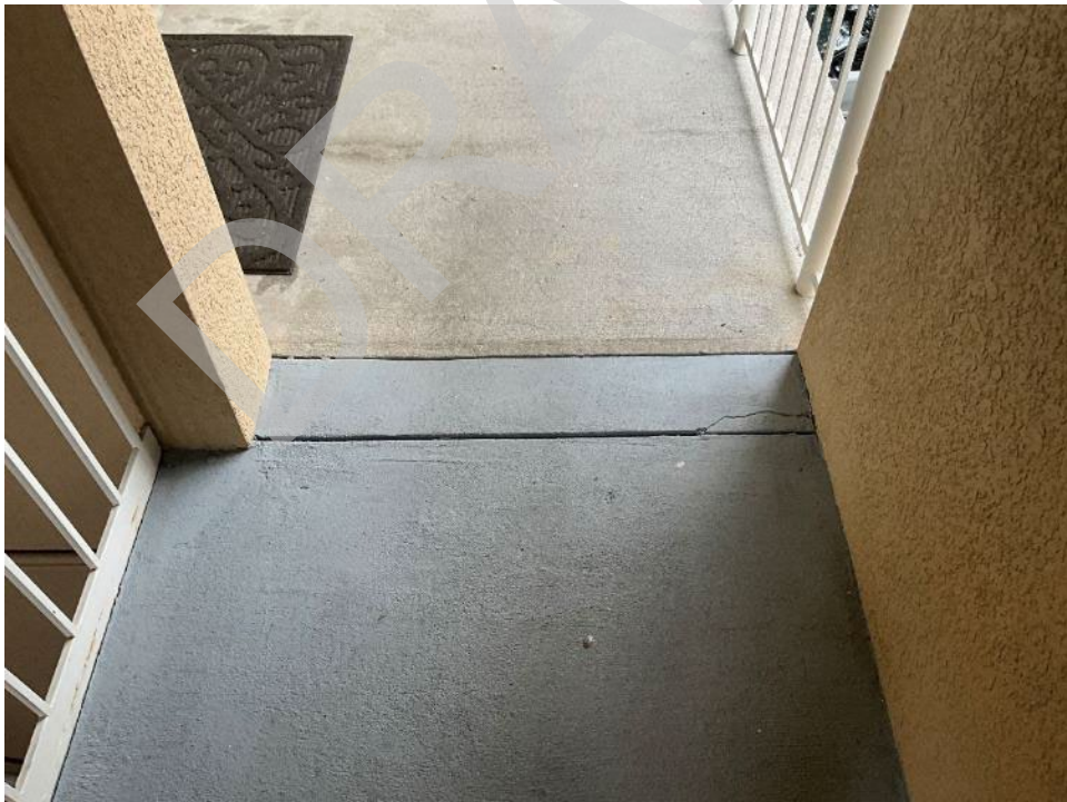
50. View of cracking around the control joint.
