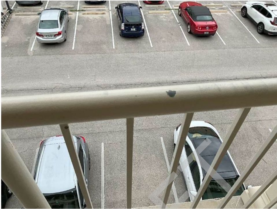
9. View of paint delamination along the breezeway railing at each building.
