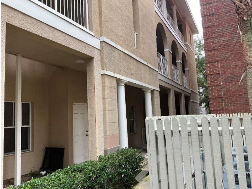
31. View of corrosion along edges of column in rear elevation.
