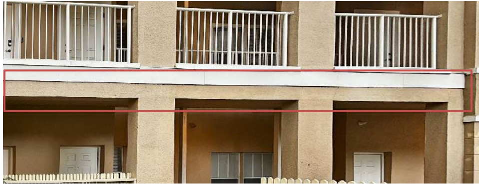
19. View of cracked section of beam below the Building A breezeway. The paint and stucco will need to be removed to expose the beam for Phase II.
