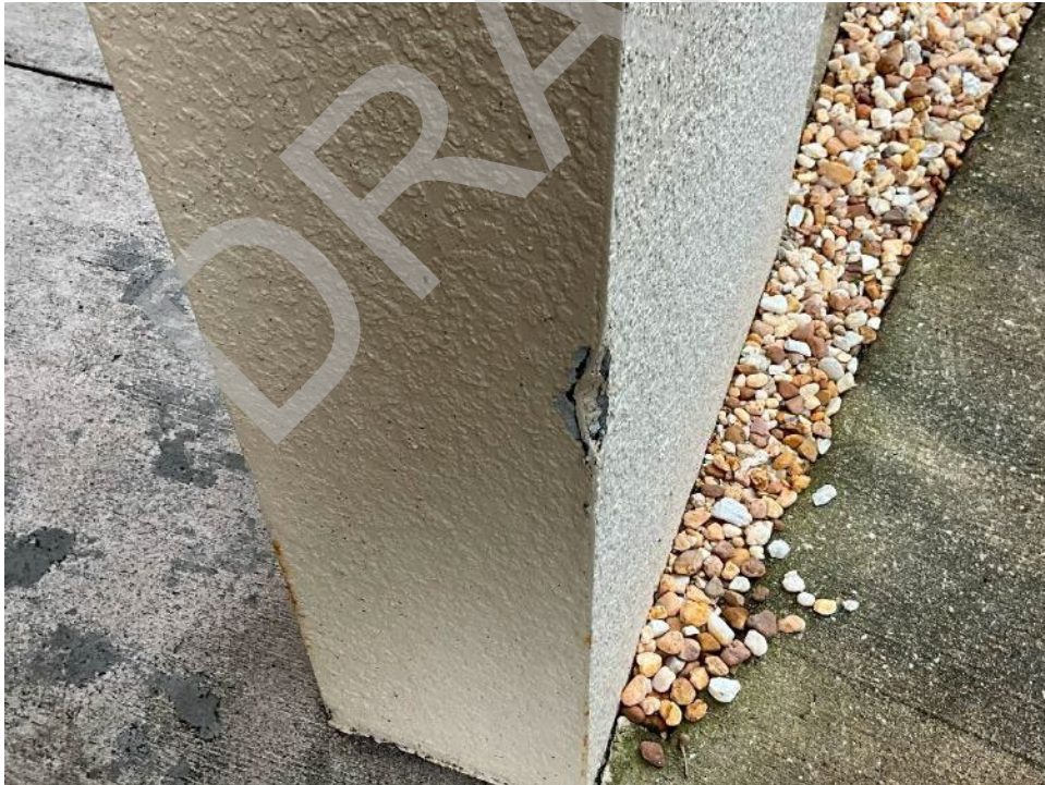
92. View of spalled concrete column near unit H103.
