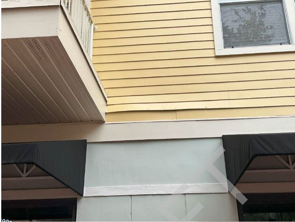
107. View of bulging siding observed around the building.
