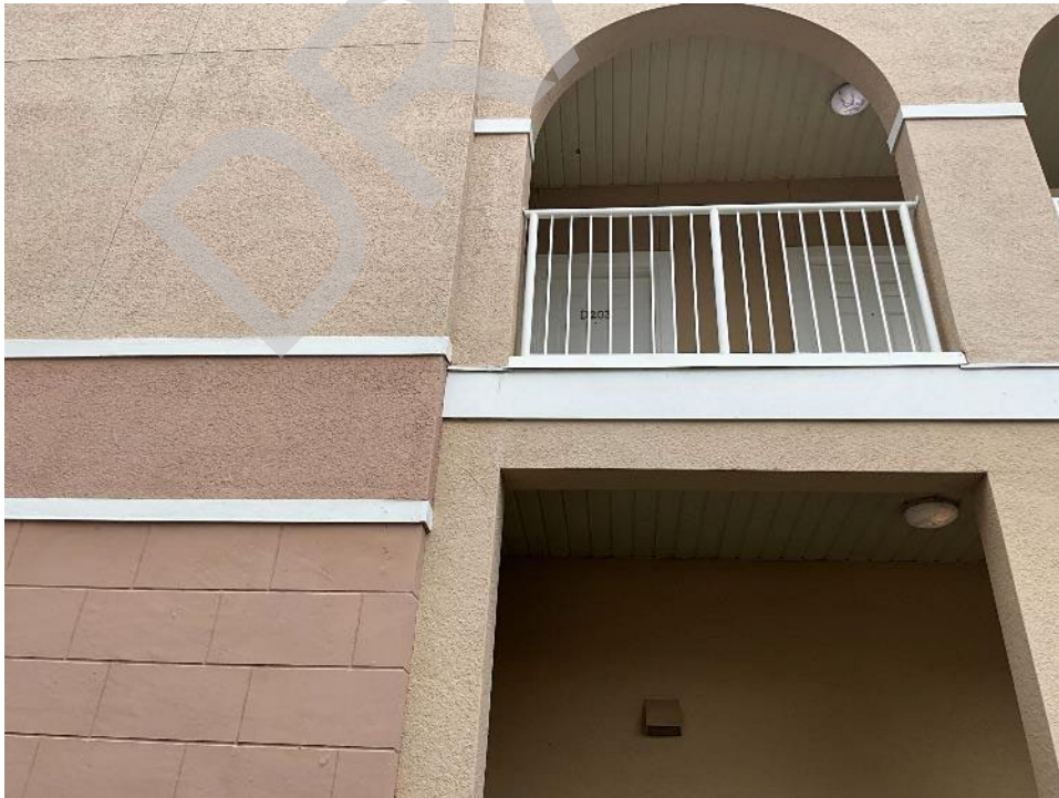
54. View of cracked section along the exterior column near D203. The stucco will need to be removed to expose the column for Phase II.
