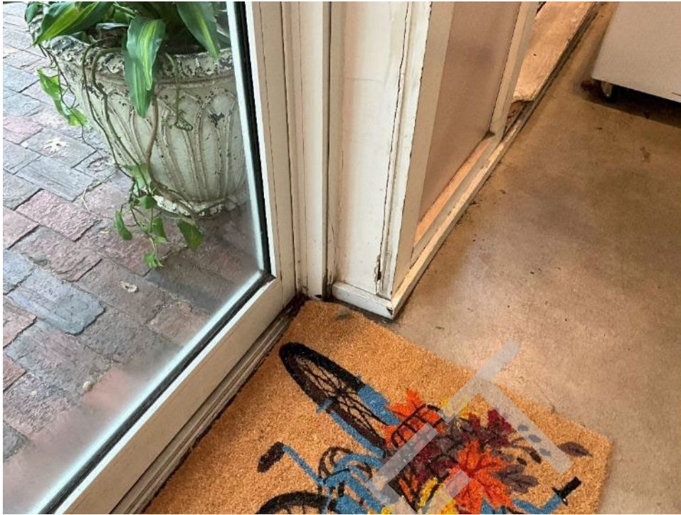
37. View of cracking along the finish around the entry door to suite B-102
