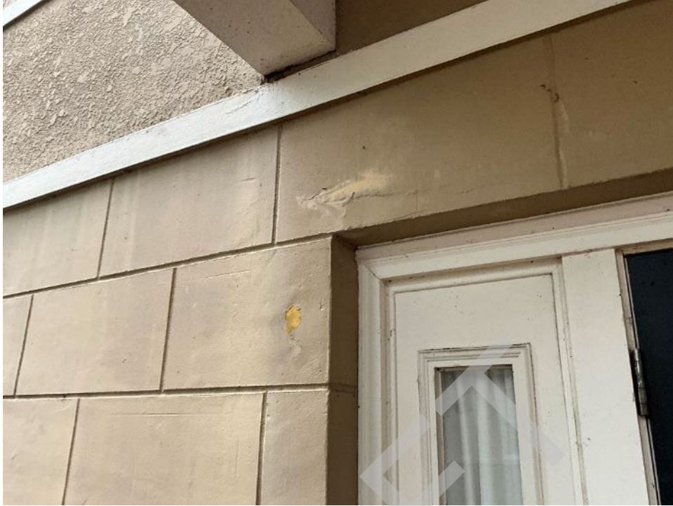
15. View of paint delamination along the walls of Building A.
