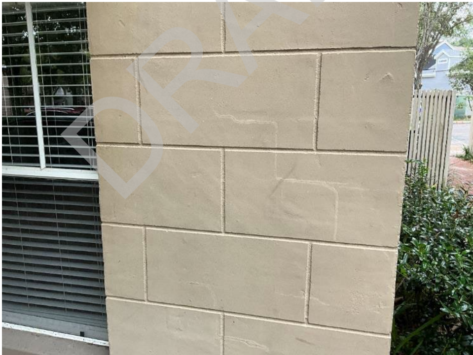
36. View of stair step cracking on the exterior wall.
