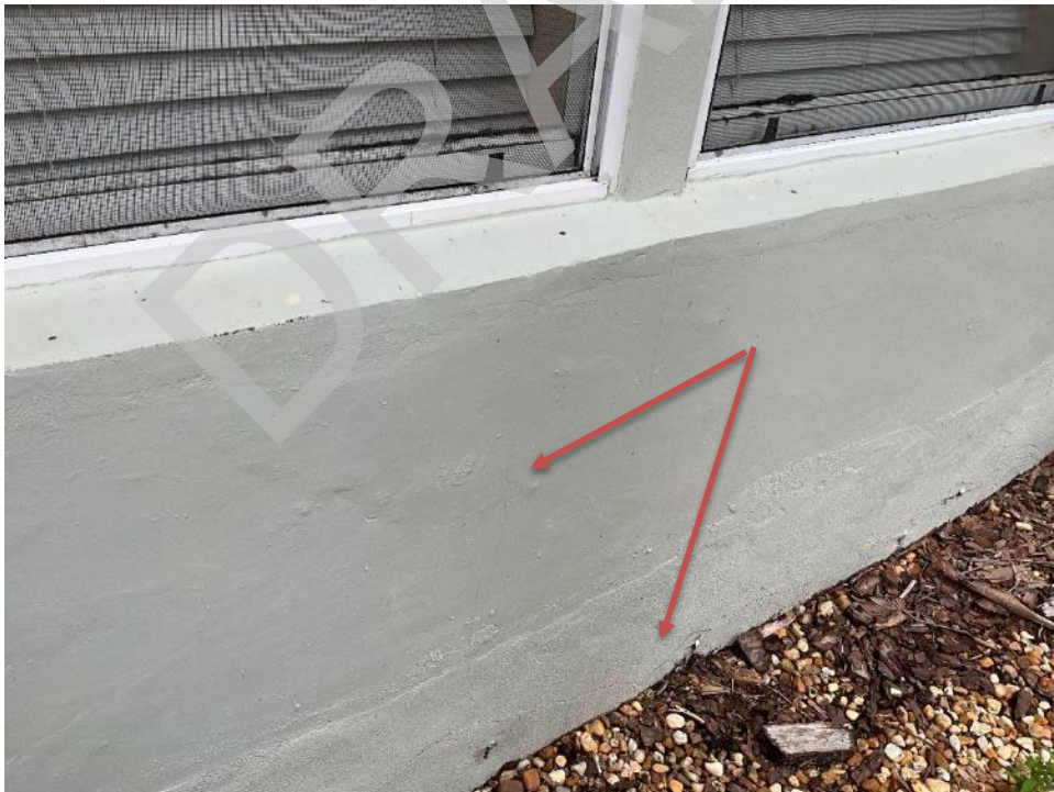
108. View of cracking in the base of the walls.
