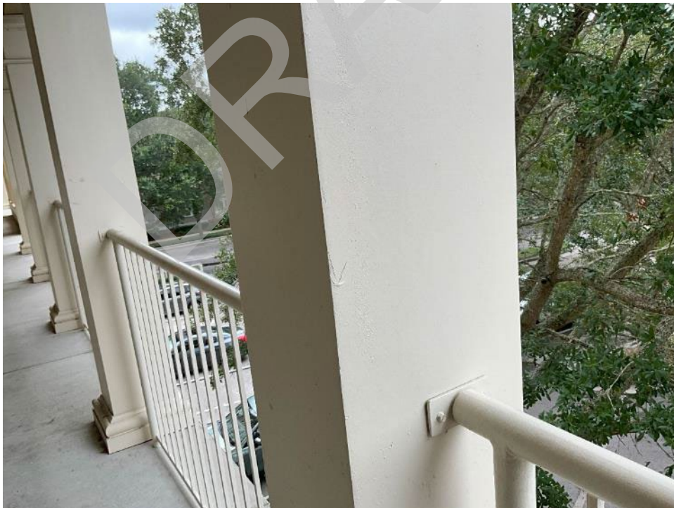
98. View of bubbling in the paint in the column near unit H304.
