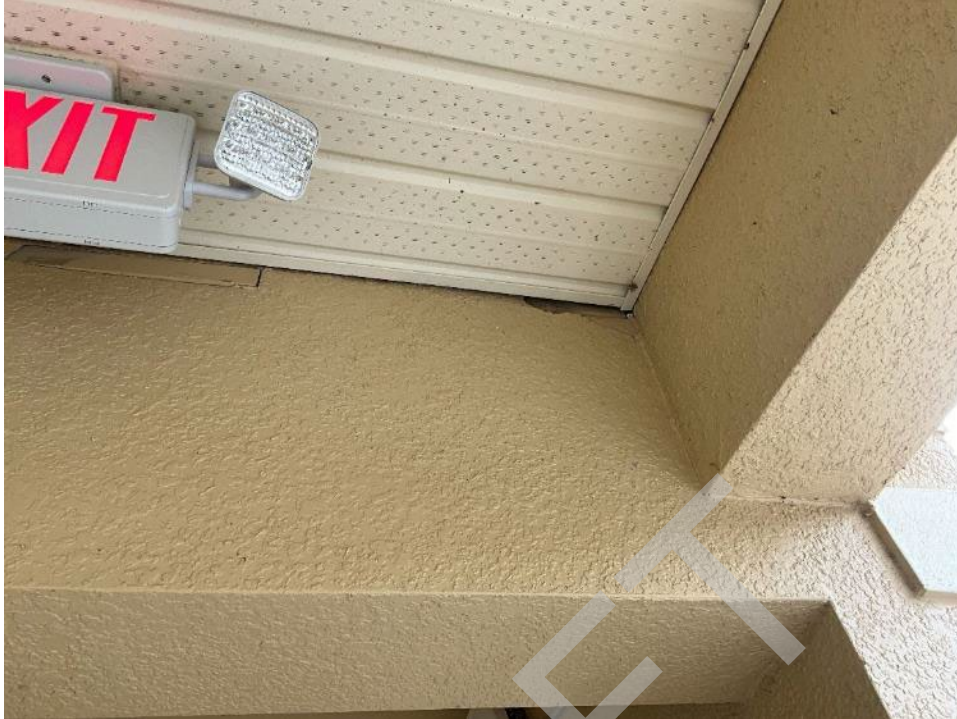
85. View of finish cracking in the beam near the stairwell.
