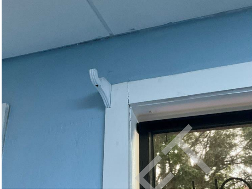
41. View of crack in the finish around a window in suite B-103.
