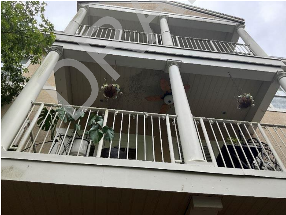
16. View of staining observed on the ceiling of a balcony of Building A.
