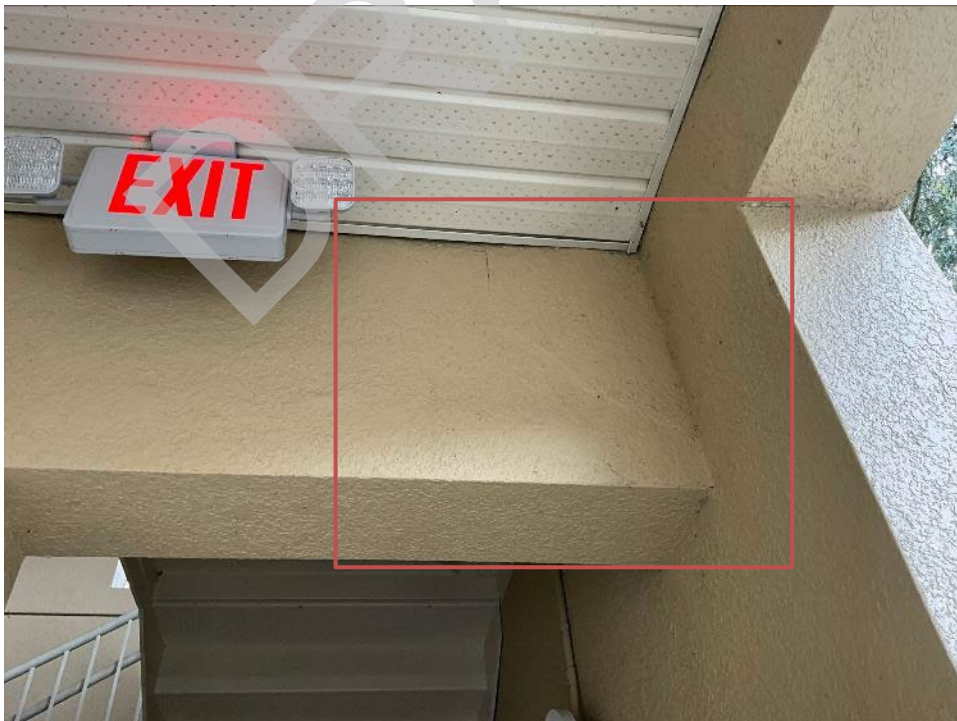
88. View of cracked section along the beam near unit H201. The stucco will need to be removed to expose the beam for Phase II.
