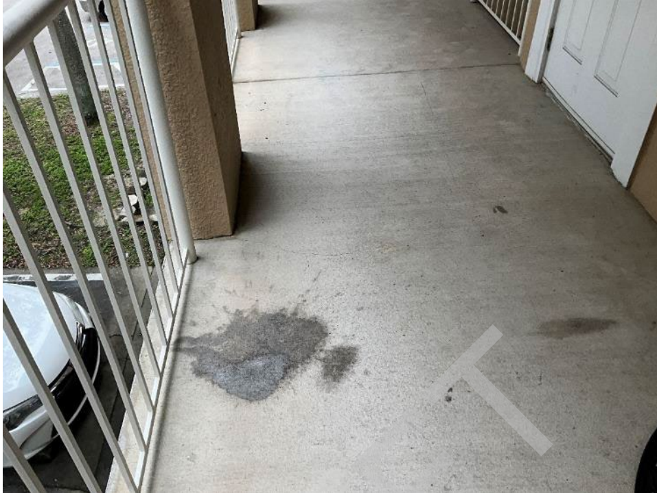
51. View of staining along the breezeway floor in front of unit C201.
