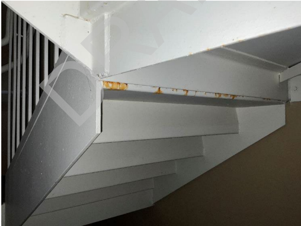
32. View of corrosion under stairs in stairwell.
