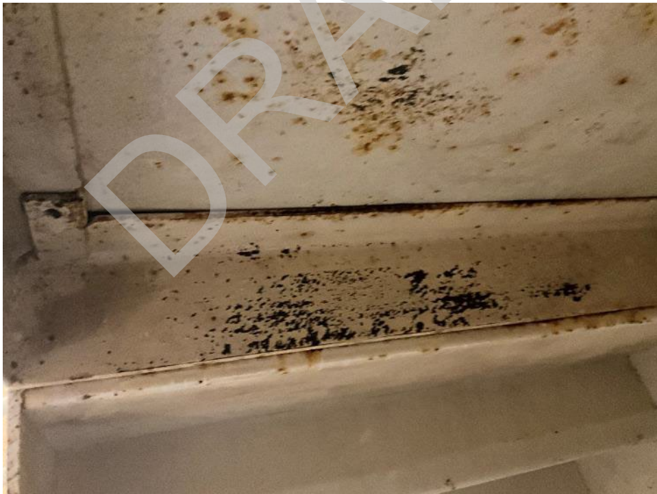
22. View of corrosion below the metal stairs.
