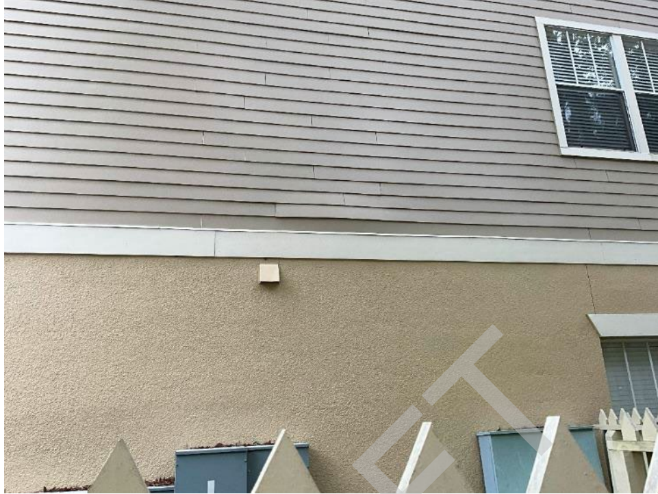
81. View of bulging along the siding of the building.
