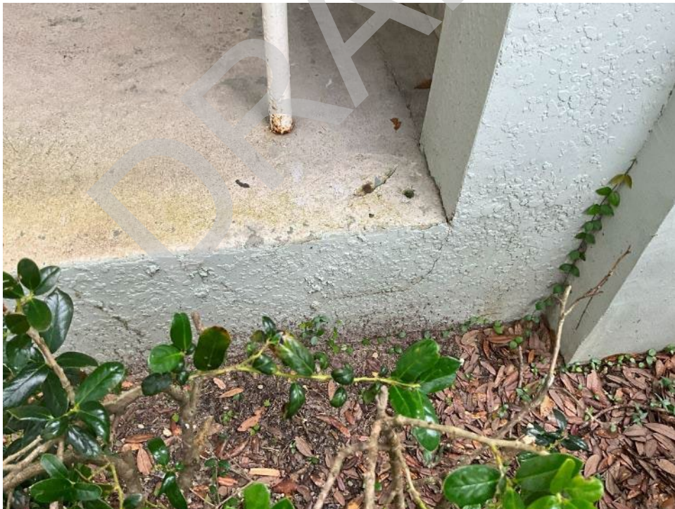
112. View of cracking in the stucco in front of the bottom slab.
