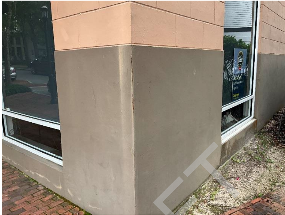
59. View of corrosion at the corners of the building.
