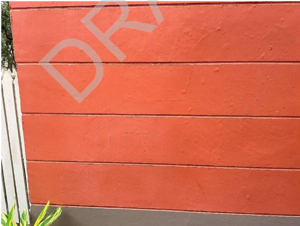
102. View of stair-step cracking observed in multiple walls around the building.
