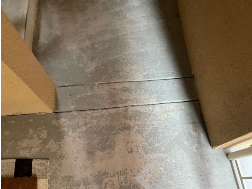
33. View of cracking along control joint and delamination along the breezeway floors.
