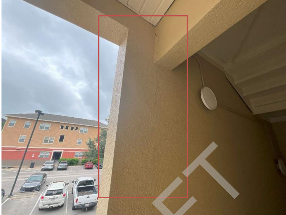
75. View of cracked section along the wall near unit G204. The stucco will need to be removed to expose the wall for Phase II.
