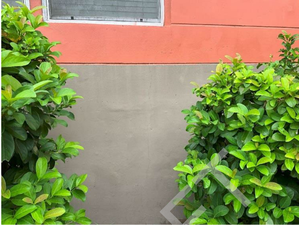
103. View of vertical cracking in base of walls.
