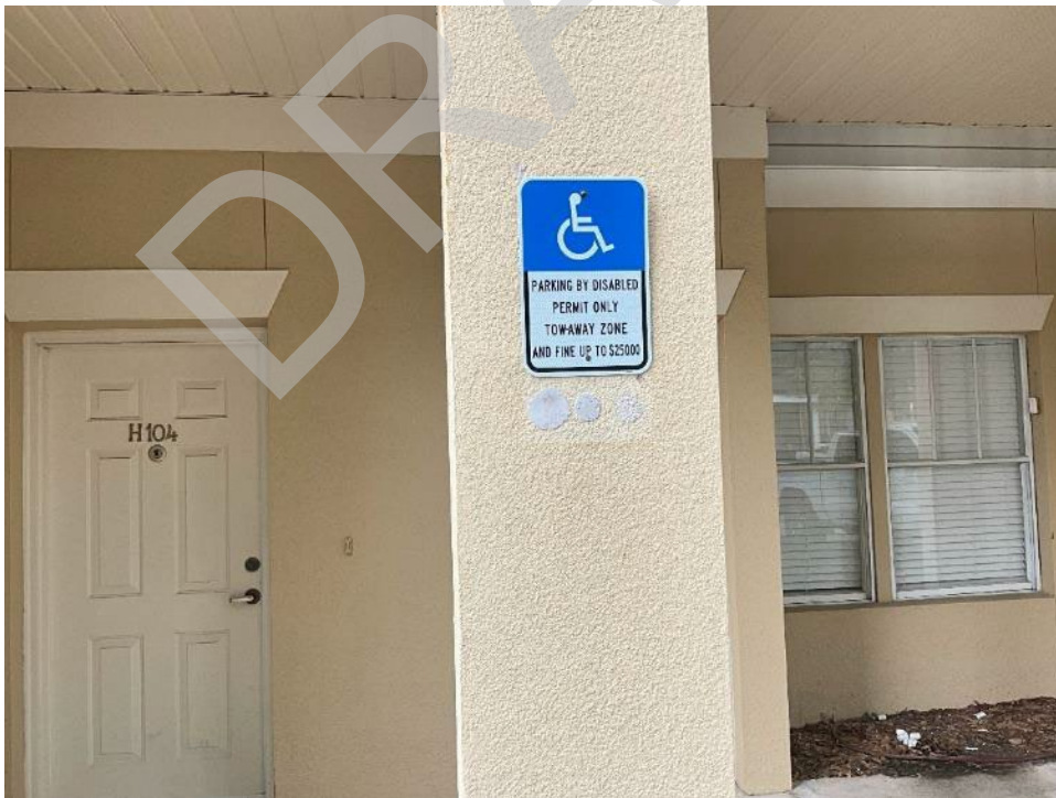
90. View of unrepaired column section unit H104.
