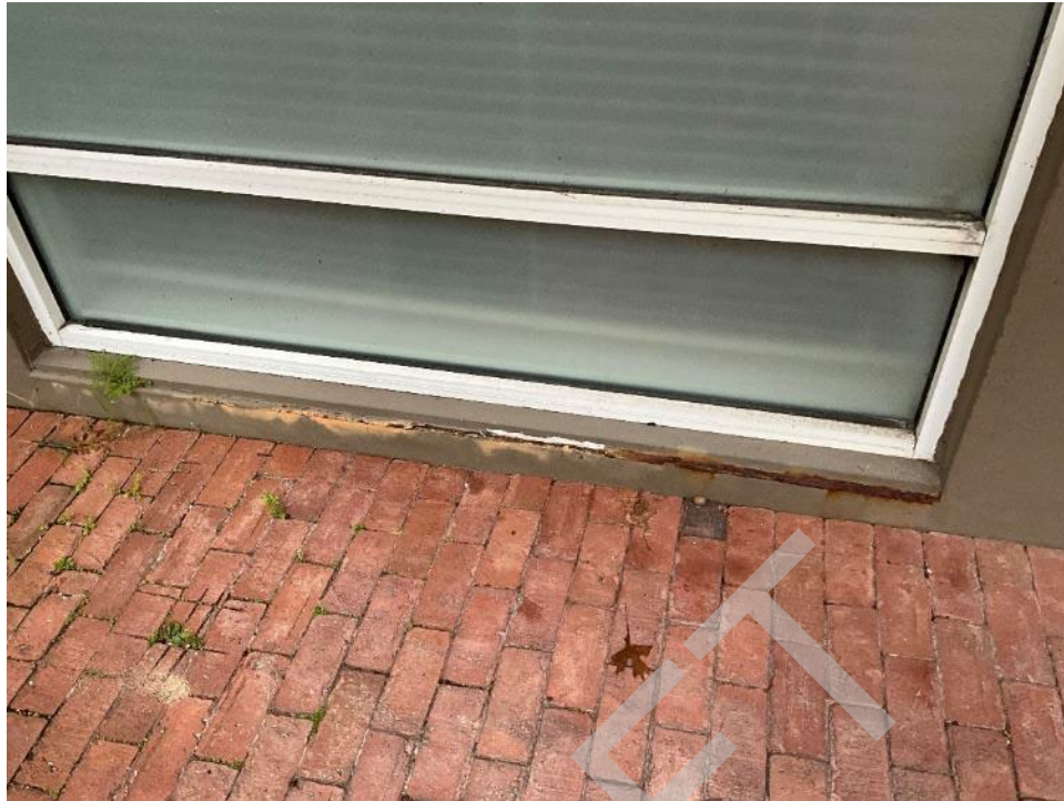
17. View of staining and corrosion along the base of the window of Suite A-103.
