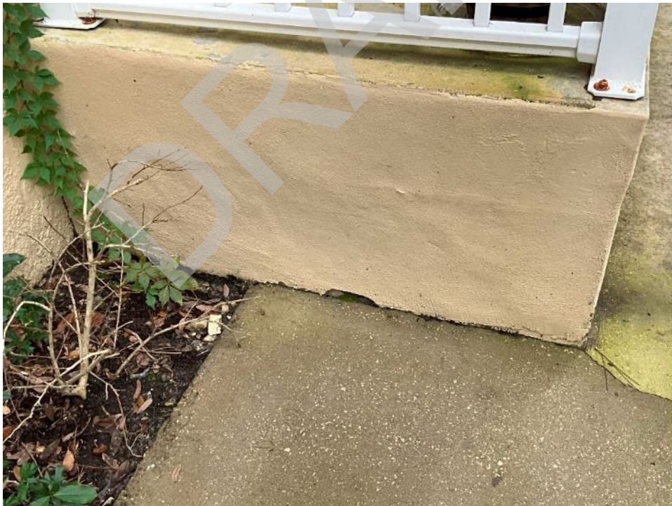
96. View of spalled section and minor bulging along the concrete stairs of unit H104.
