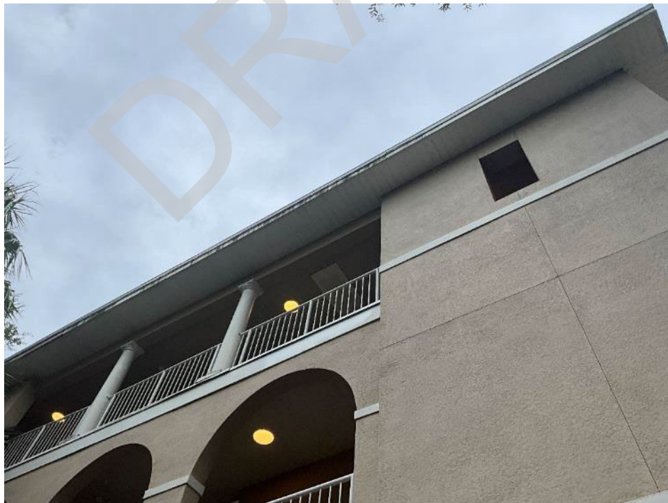
6. View of staining around the fascias of each building.
