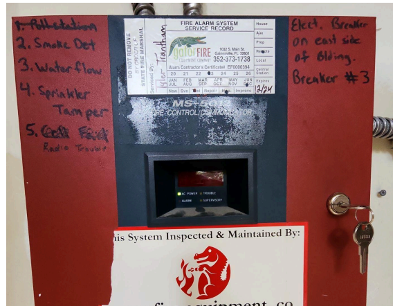
Typical Fire Alarm Control Panel
