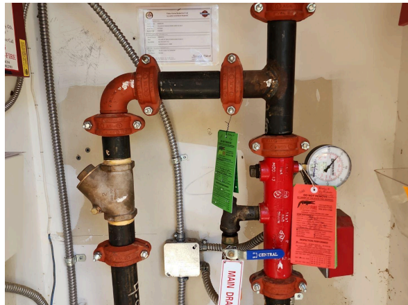
Fire Suppression Equipment
