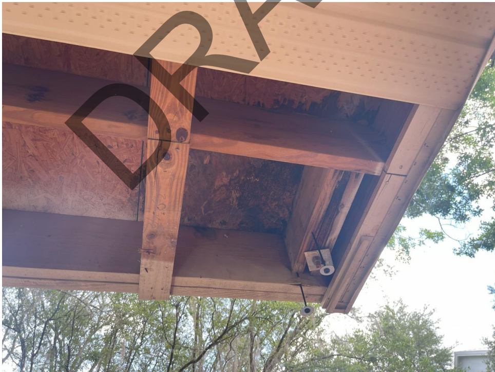
Photograph 2: View of deteriorated oriented strand board (OSB) sheathing below the balcony at Unit A-201.
