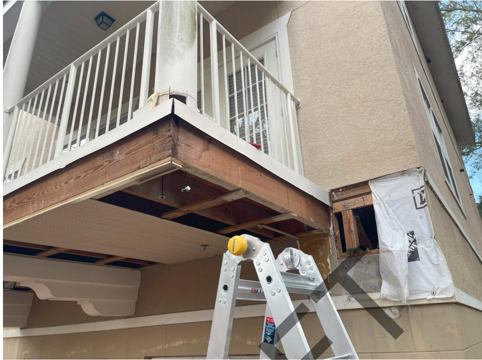
Photograph 5: View of the exposed wood framing at the balcony of Unit A-201 and the exposed wood floor trusses between the first and second floors.
