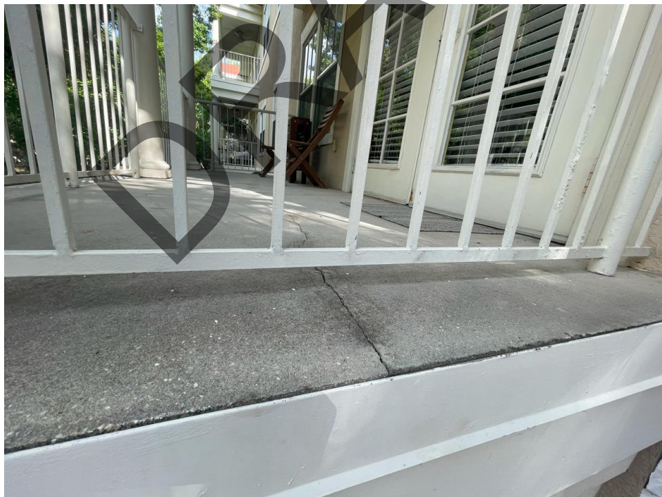
Photograph 4: View of cracking observed in the concrete balcony slab at Unit A-201.
