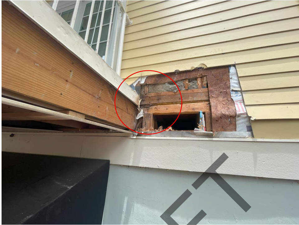
Photograph 11: View of stained wall framing observed to the east of the balcony at Unit J-202.
