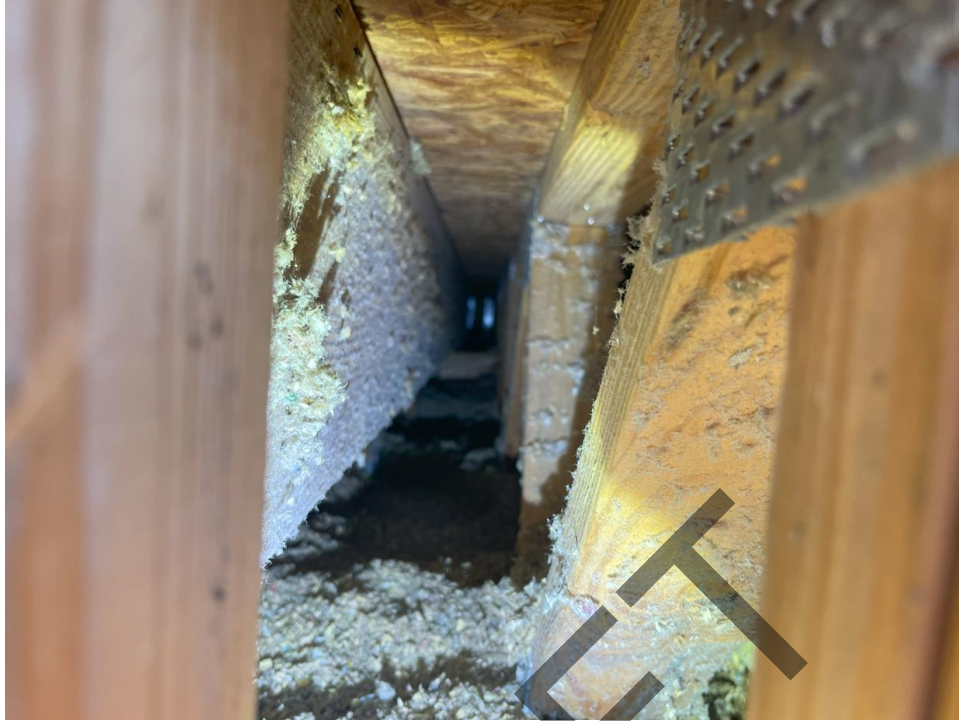
Photograph 7: View of an approximately 3- to 4-inch gap between the balcony joist and the floor truss between the first and second floors at Unit A-201.
