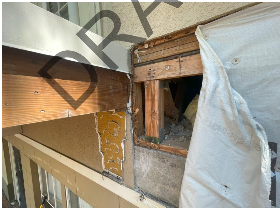
Photograph 6: View of the exposed wood framing at the balcony of Unit A-201 and the exposed wood floor trusses between the first and second floors.
