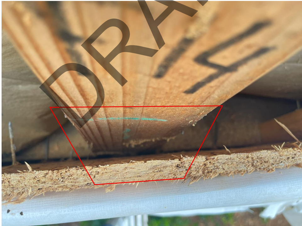
Photograph 12: View of missing fasteners between the OSB sheathing and wood framing along the west elevation of Building K.
