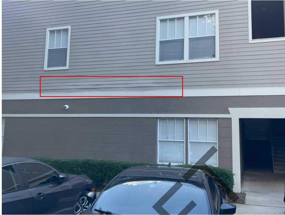
Photograph 9: View of bulging siding observed along the west elevation of Building K.
