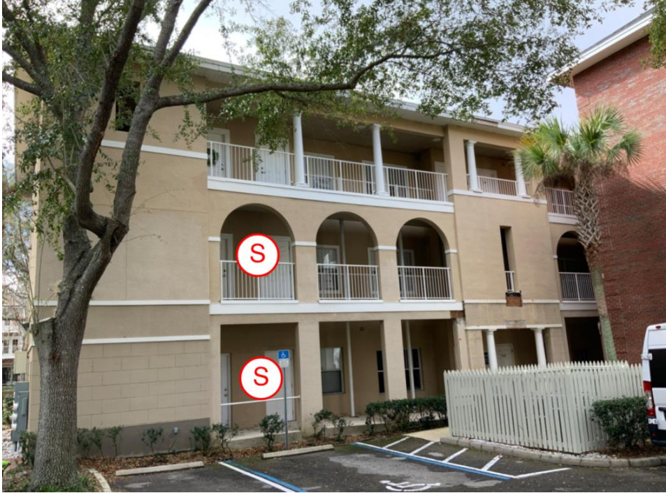
Shoring 3: View of shoring locations along the north elevation of building B.
