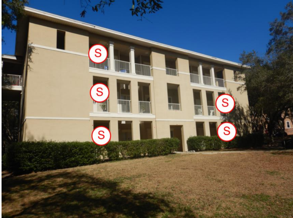
Shoring 7: View of shoring locations along the south elevation of building E.
