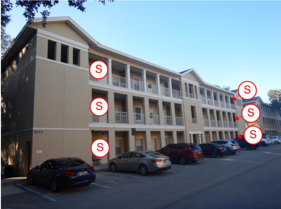
Shoring 9: View of shoring locations along the east elevation of building G.
