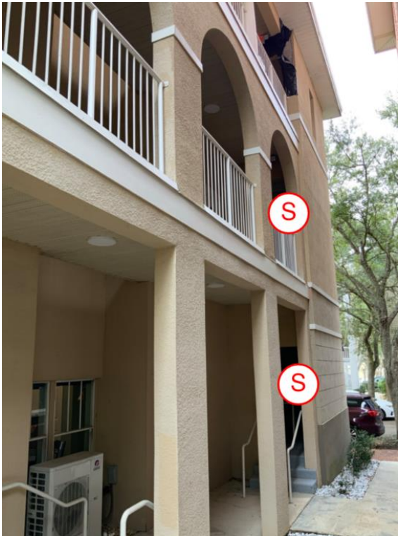
Shoring 4: View of shoring locations along the north elevation of building B.
