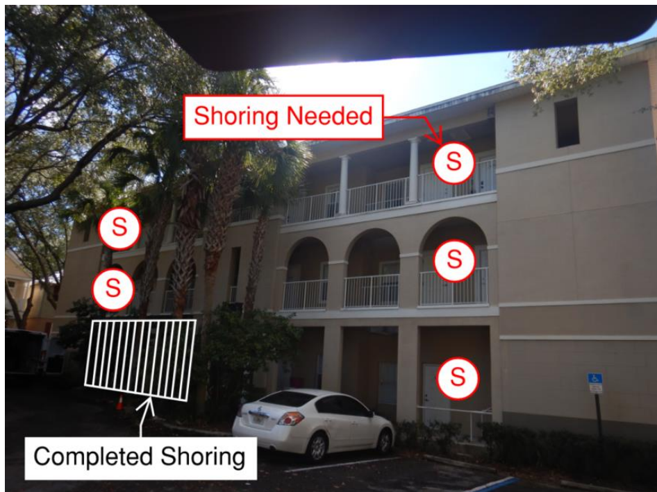
Shoring 2: View of shoring locations along the north elevation of building A.
