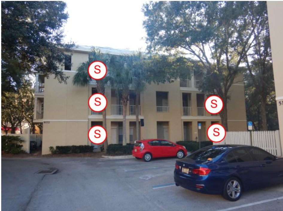
Shoring 8: View of shoring locations along the north elevation of building F.
