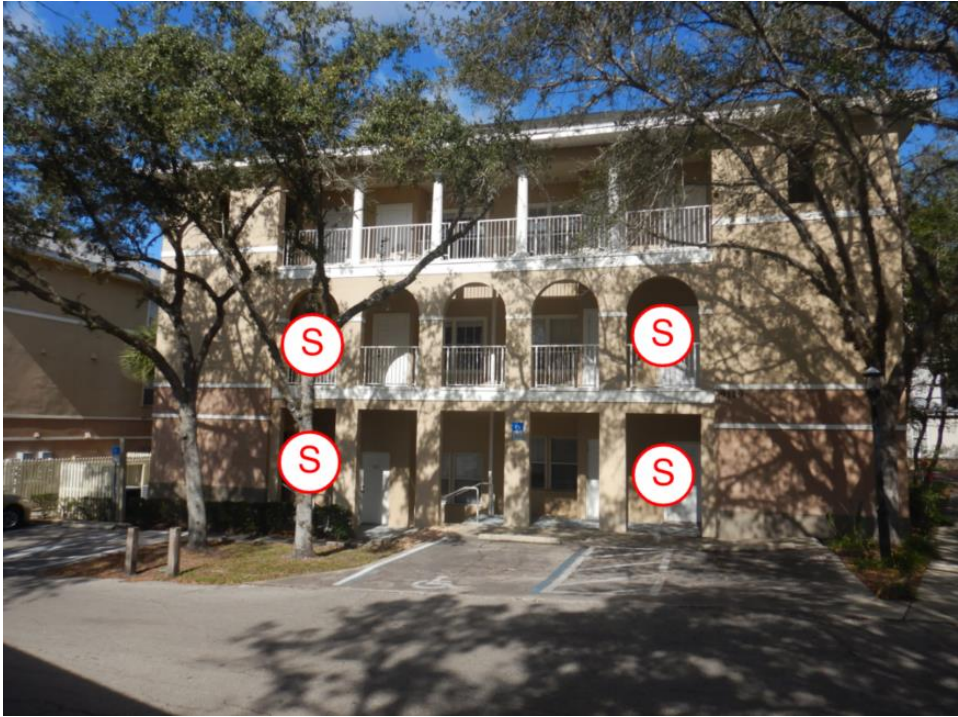
Shoring 5: View of shoring locations along the south elevation of building C.
