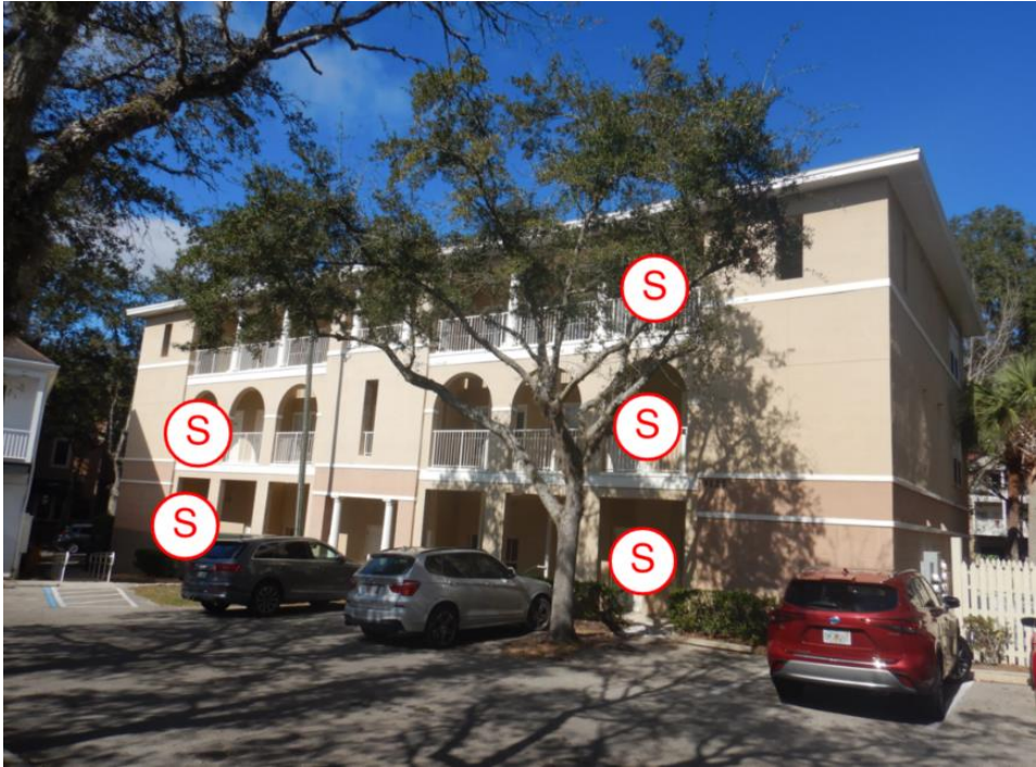
Shoring 6: View of shoring locations along the south elevation of building D.
