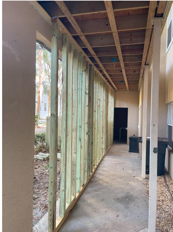
Shoring 1: View of a portion of completed shoring along the north elevation of Building A.
