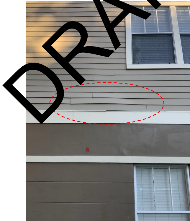
Photograph 8: View of bulging siding along the west elevation of Building K.
