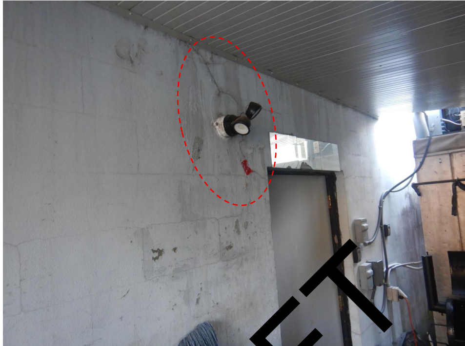
Photograph 7: View of cracked exterior wall finish along the south wall of Building I.
