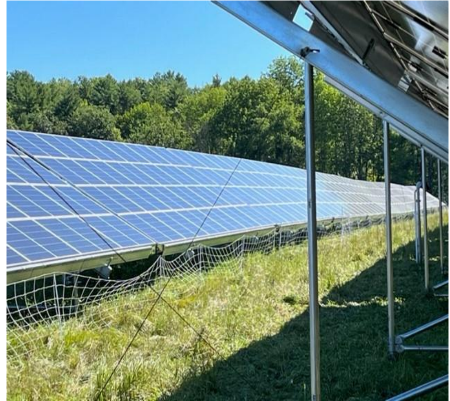
Fixed-tilt panels, low leading edge, DG site, ME
