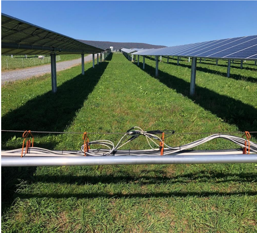
Single axis tracker panels, drive shafts, utility scale site, PA
