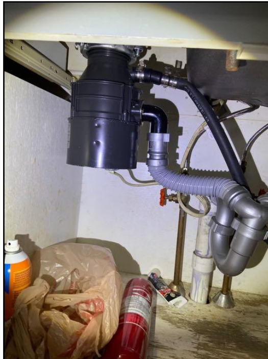
Sink backing up
