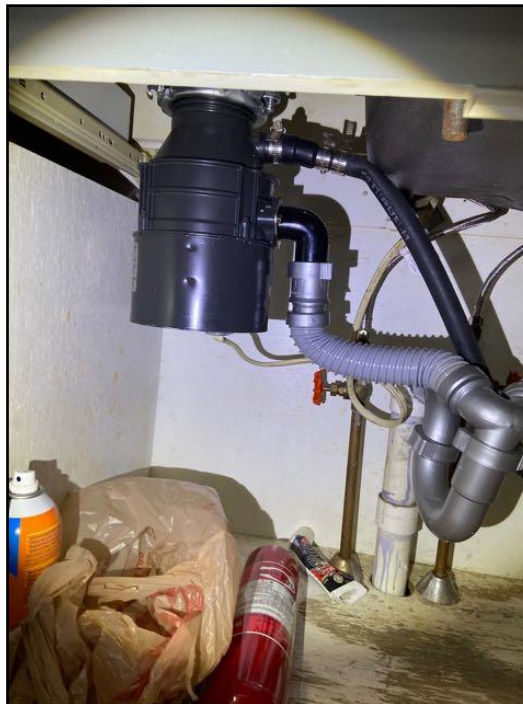
Sink backing up
