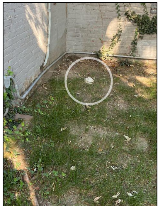
Sewer clean out
