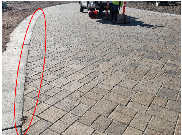
Chipped next to the concrete ribbon
