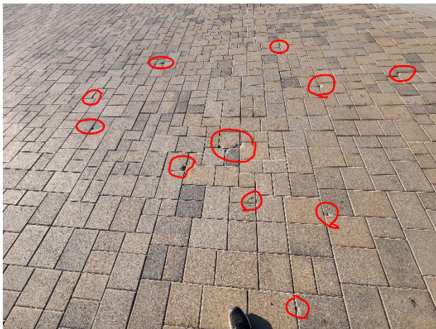
Chipped pavers are circled
