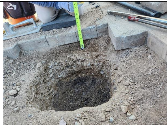
TP-3 The subgrade is different from all the other test locations. It is darker in color, has plasticity and more fines.
