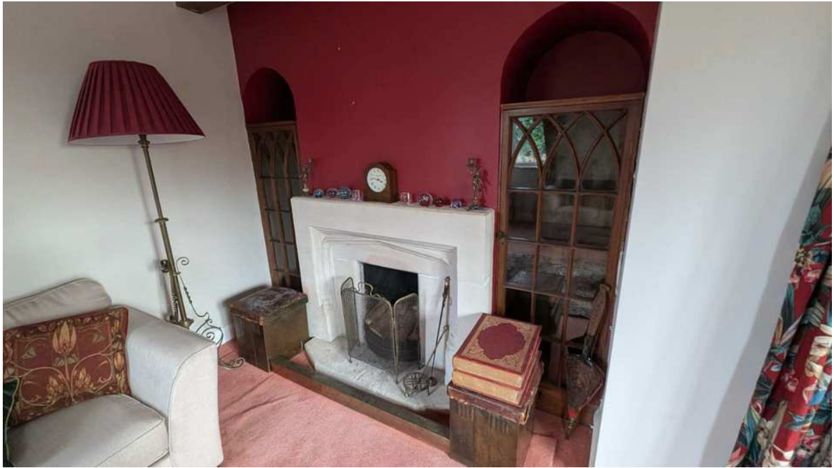
Damp smell to room - damp behind storage units.
