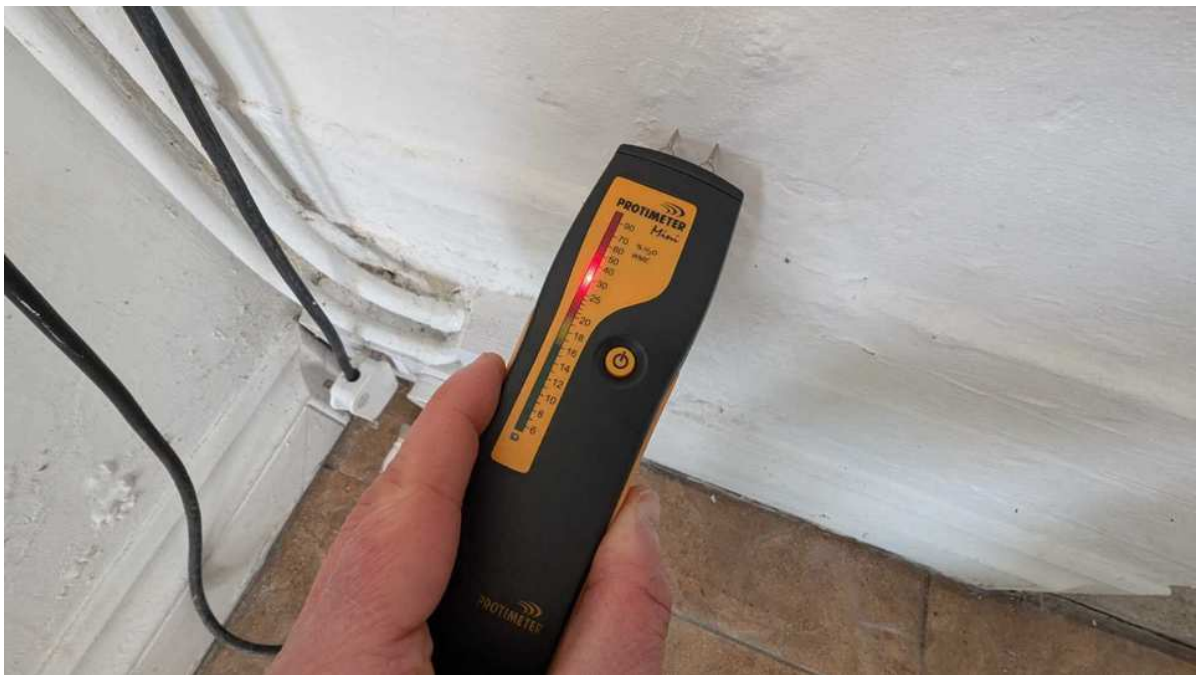
High moisture reading.
