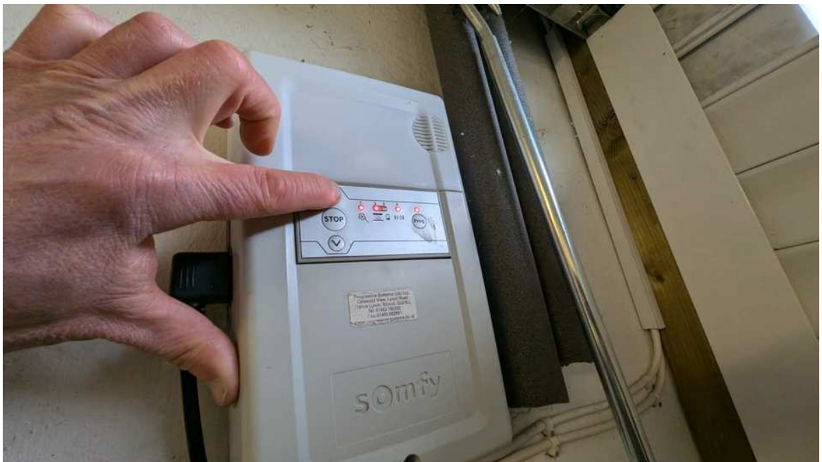
Inoperable at time of inspection.
