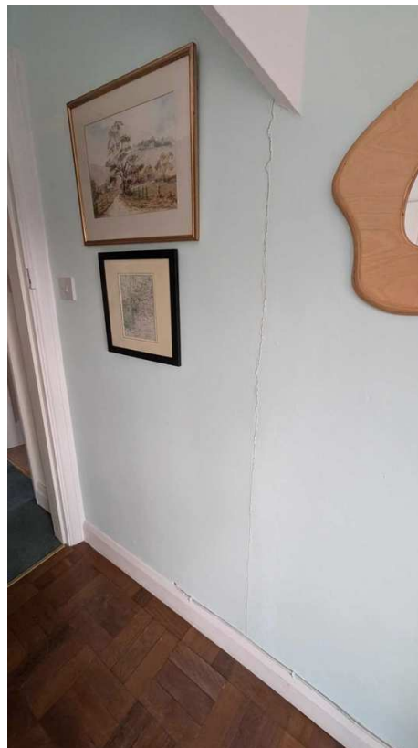
Cracking between solid wall and stud wall.
