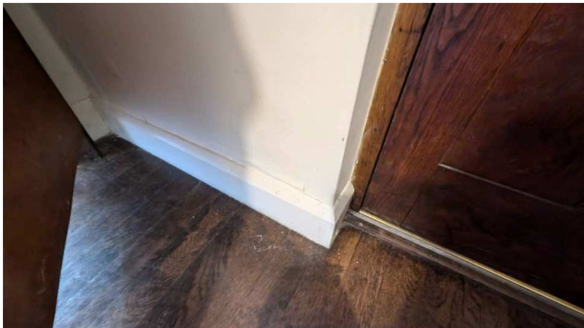
Hallway damp by front door.
