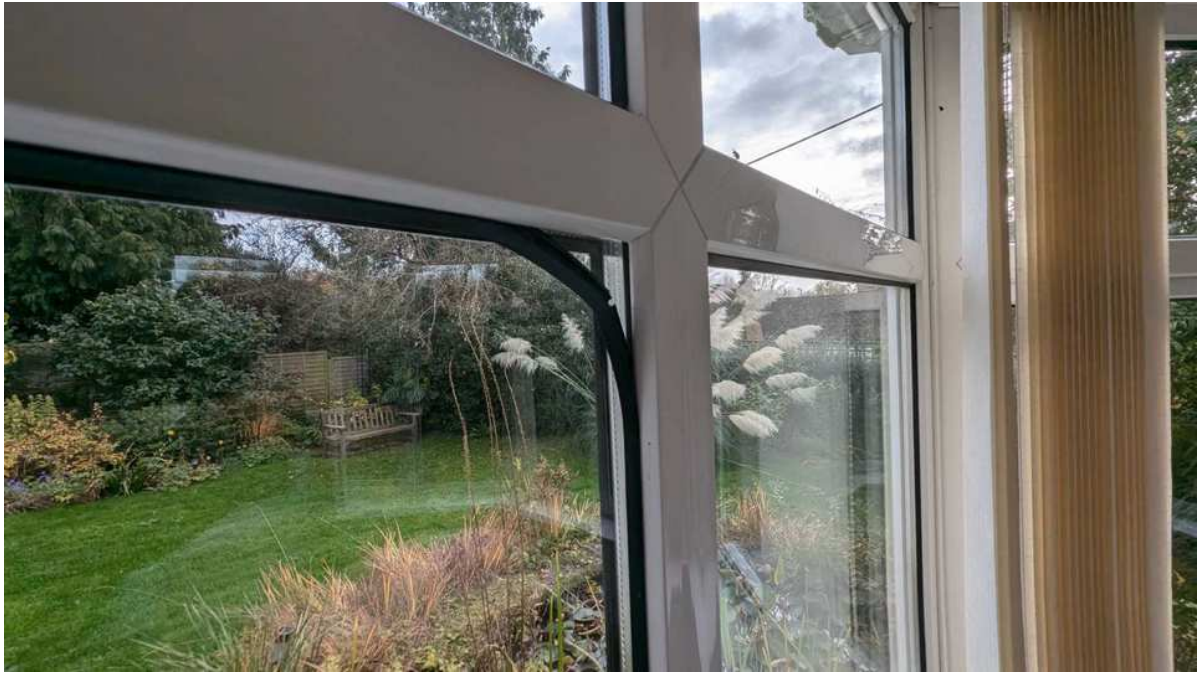
Conservatory Windows: Shrunk seals.
