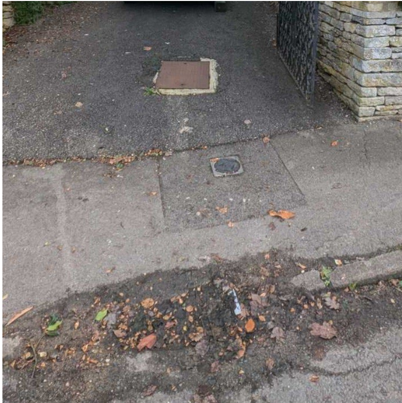
Water meter, front drive.
