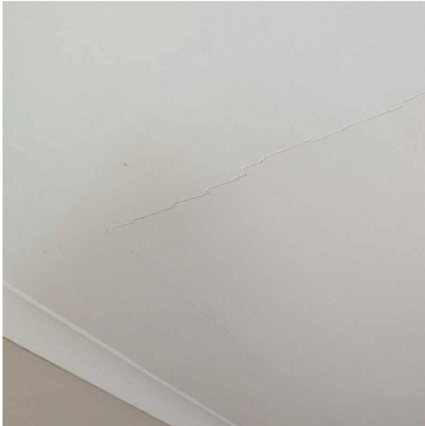
Hairline cracking to ceiling.
