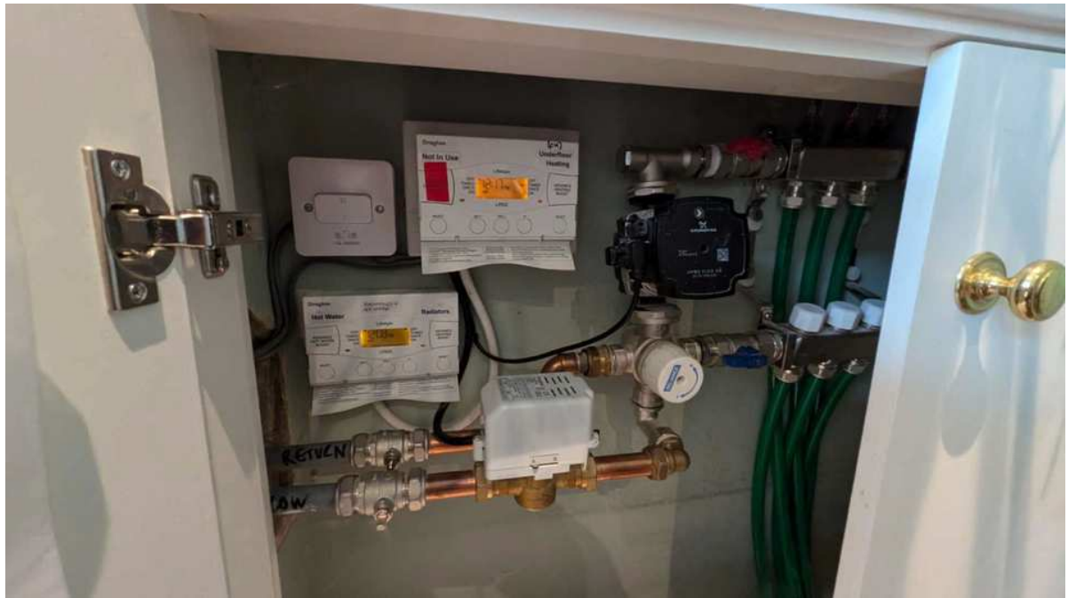
Underfloor heating controls and manifold.
