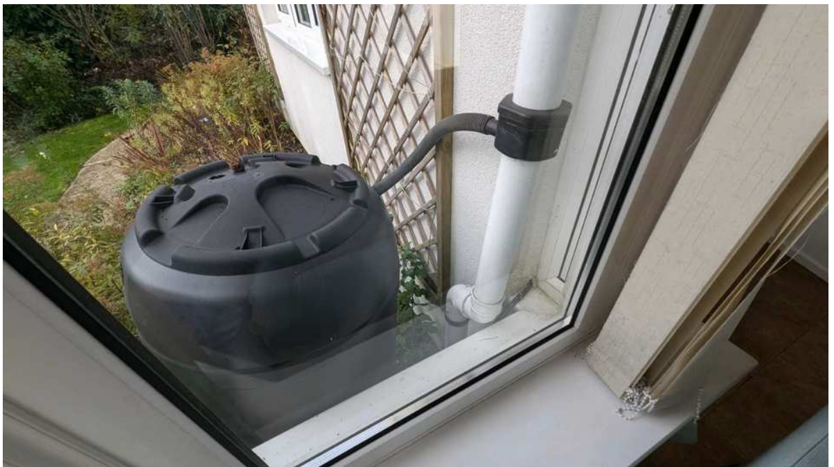
Proximity of leaky rainwater harvester.
