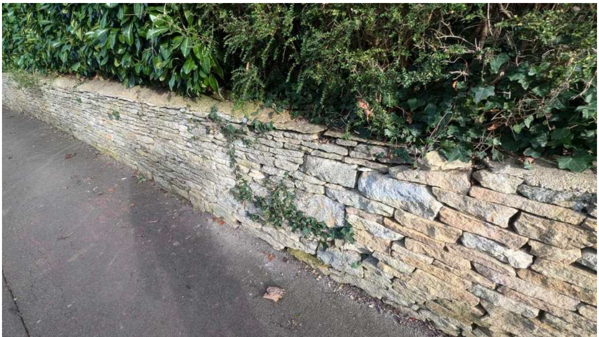
Area in need of repair.
