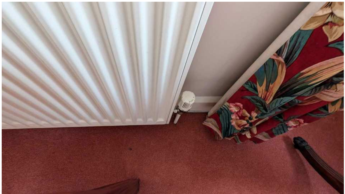
Full thermostatic control to radiators.
