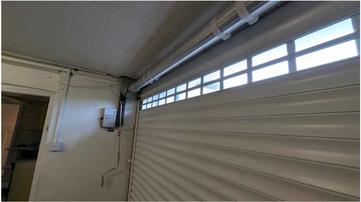
Garage roller shutter door.
