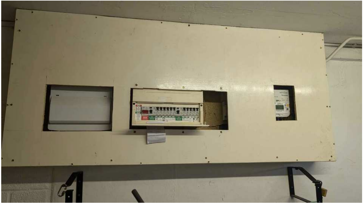
Distribution board and meter.
