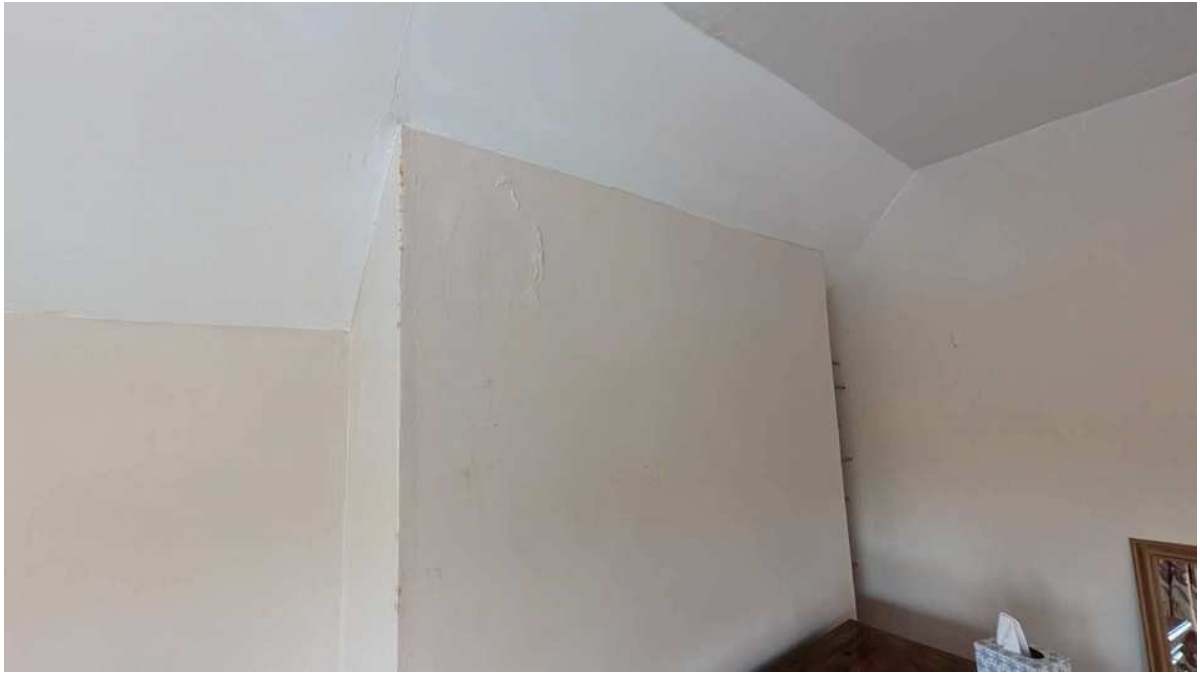
Damp to the chimney breast bedroom 2.
