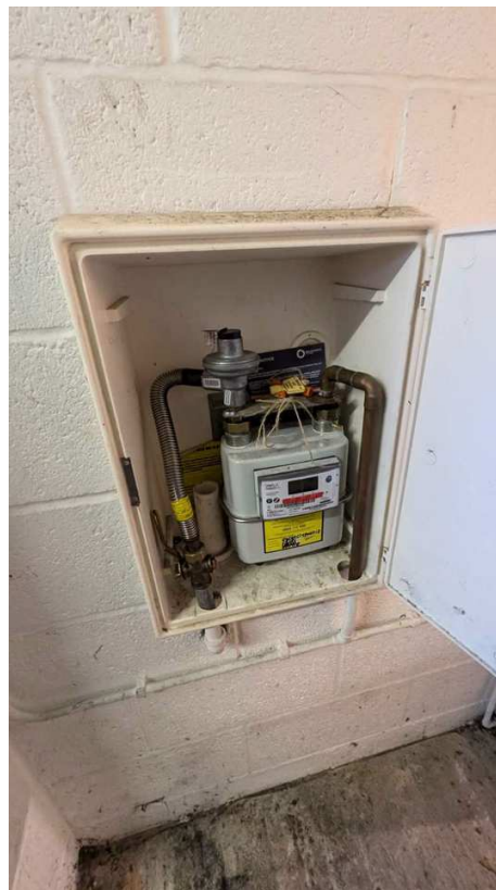
Meter box, corridor to garden.
