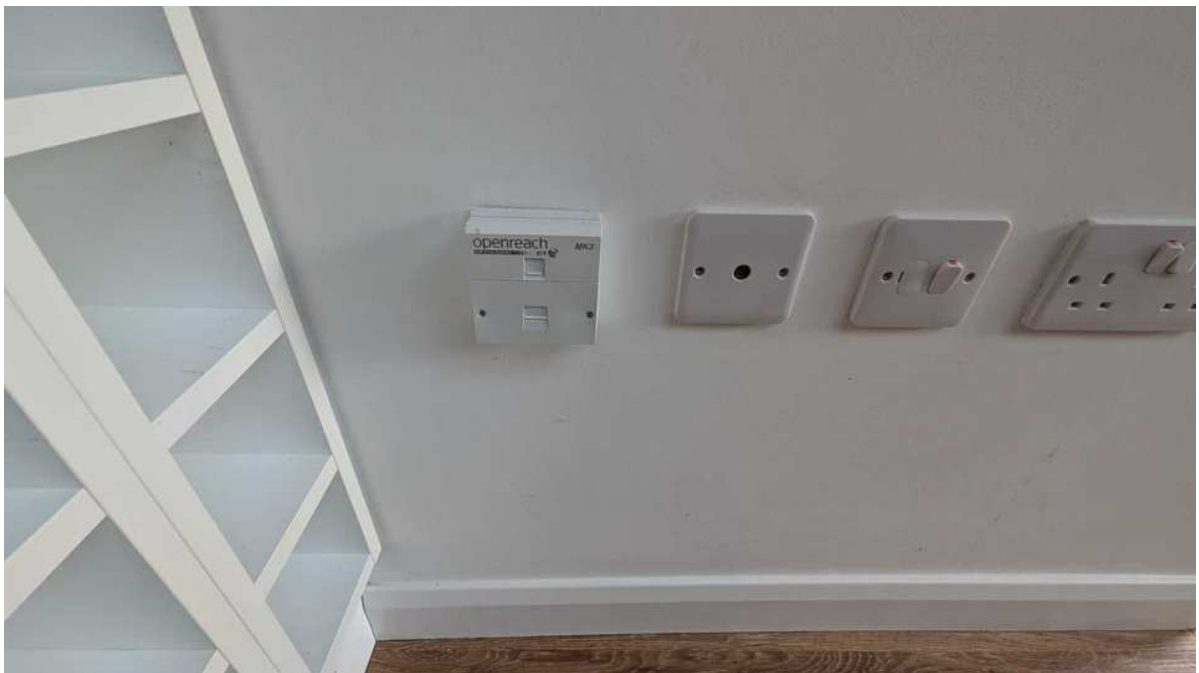
TV outputs and BT ethernet connections.
