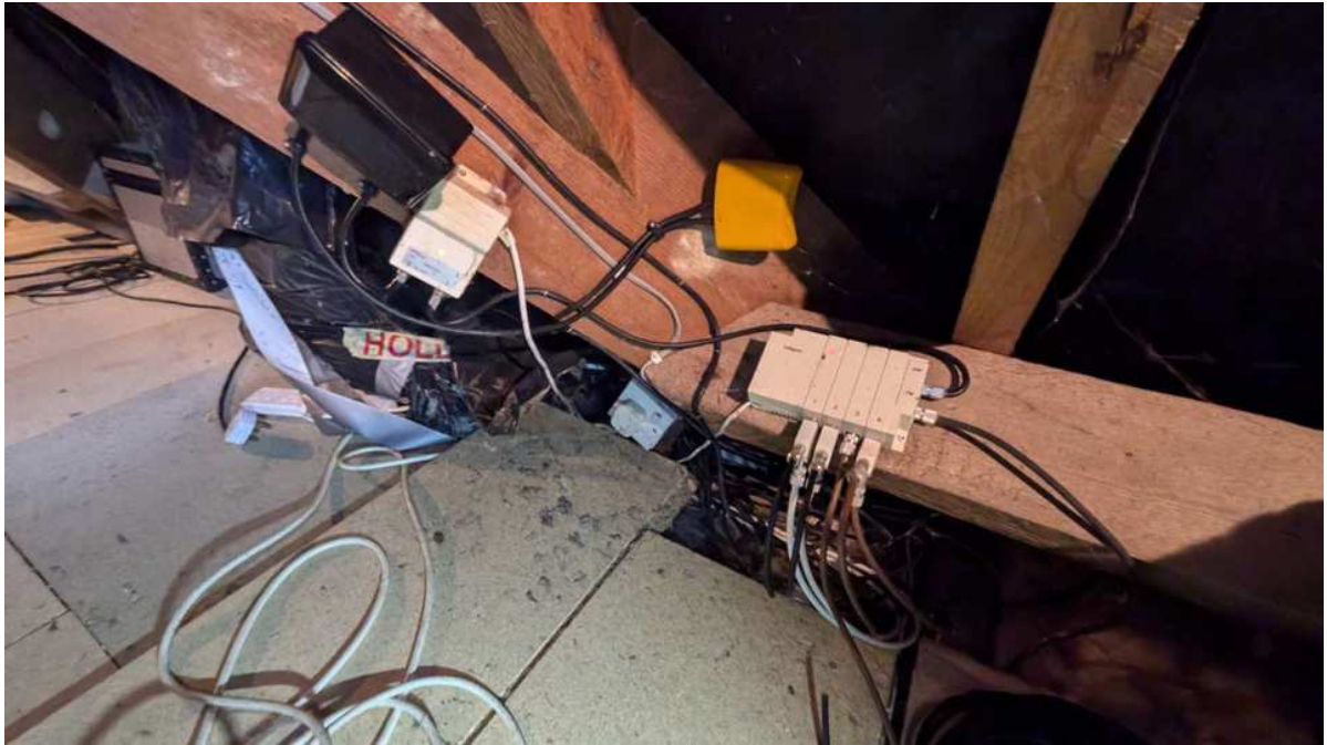
Coax setup to most rooms in the house
