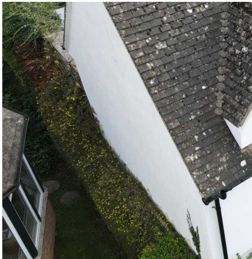
No access to wall left hand side.
