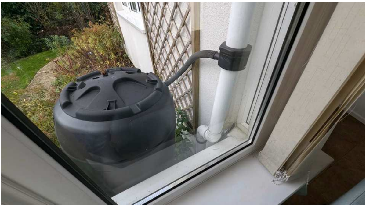
Downpipes leading to rainwater harvesting.
