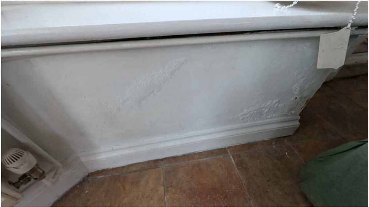
Damp internal perimeter walls.
