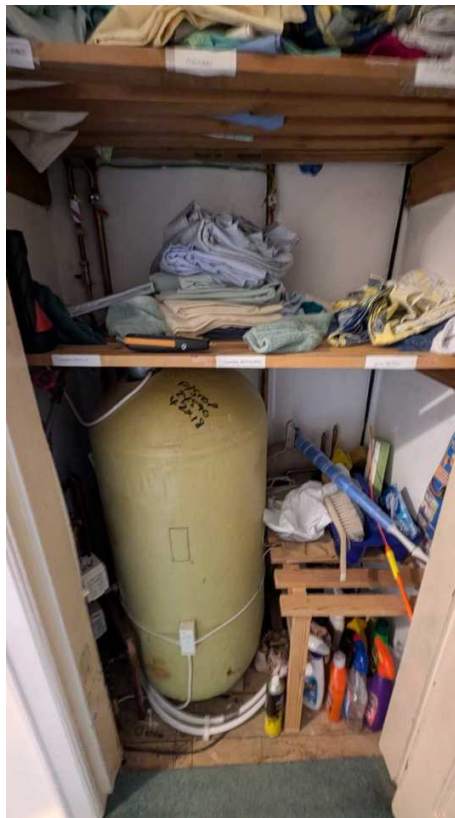
Immersion - upstairs storage room.
