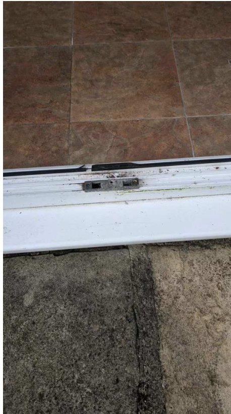
Conservatory doors catch to base.
