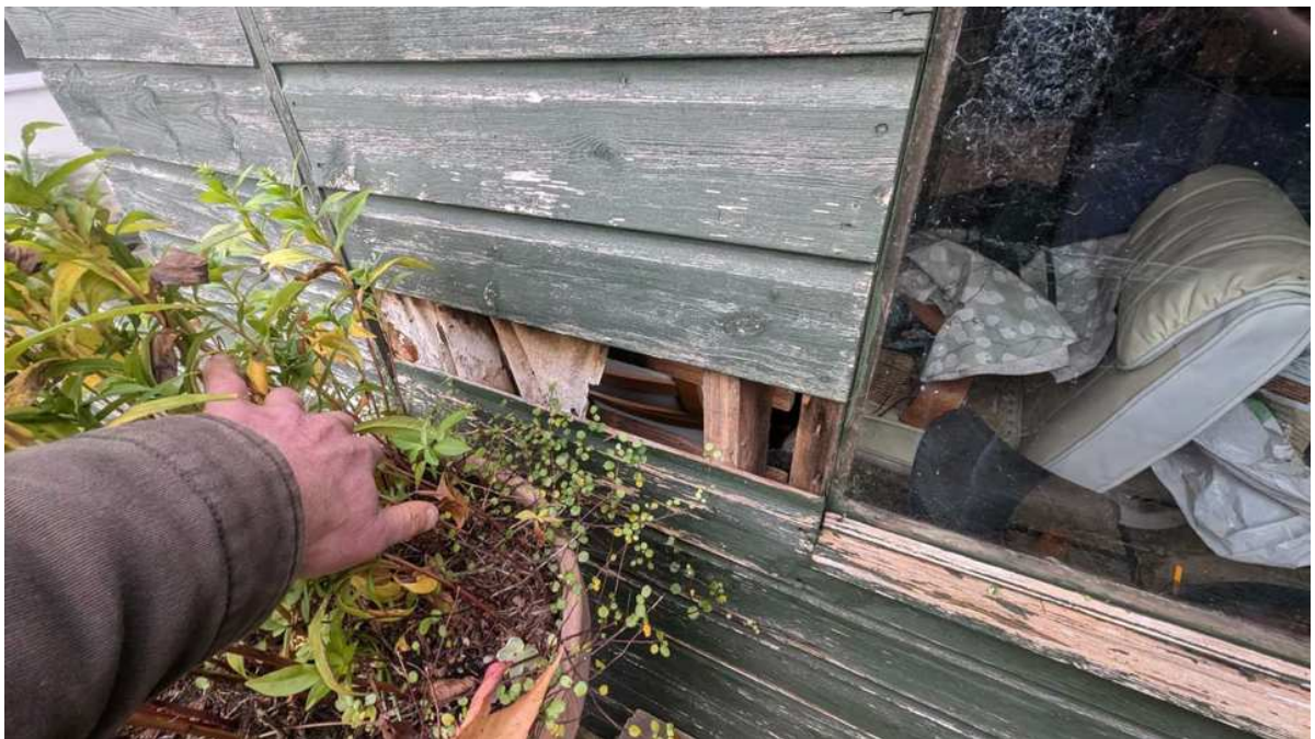
Missing wood panels.
