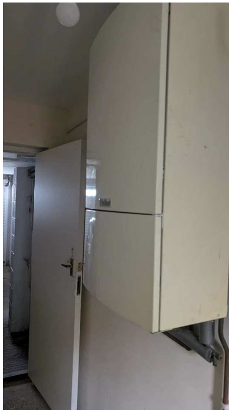
Boiler in garage corridor.
