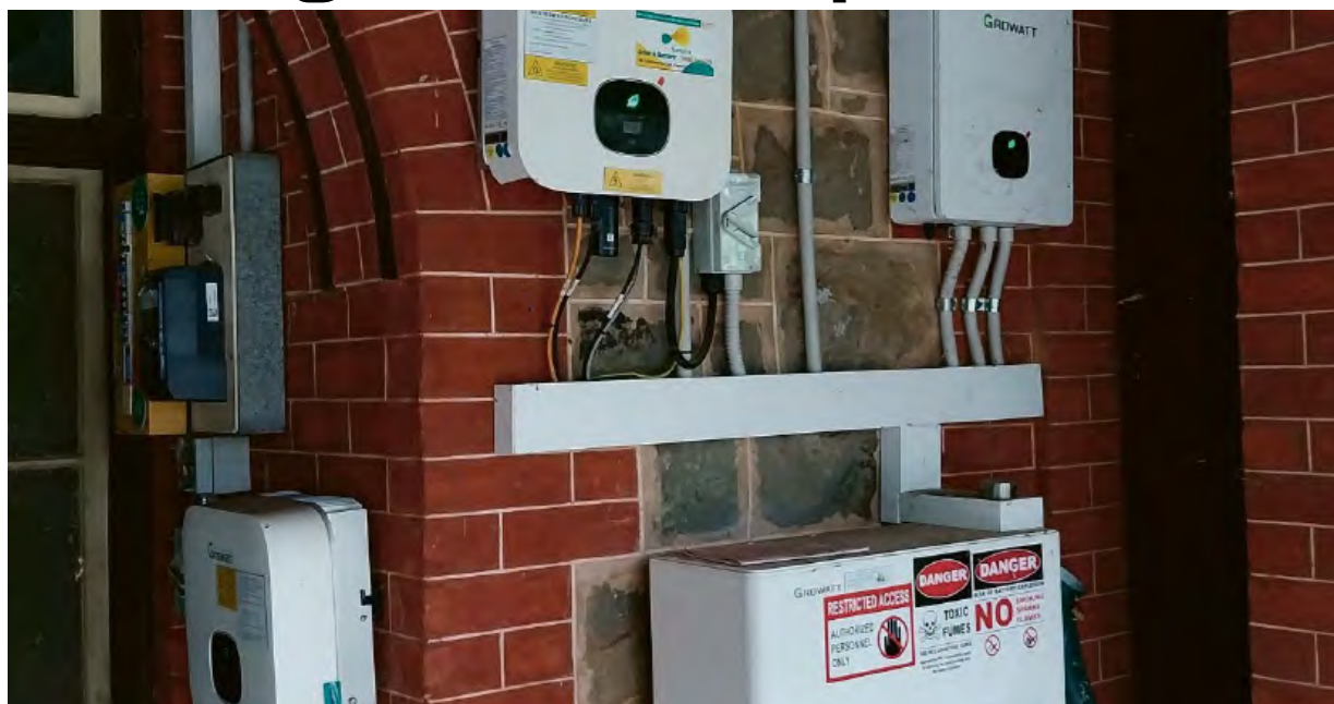
Photo: My home 15kWh solar battery system
