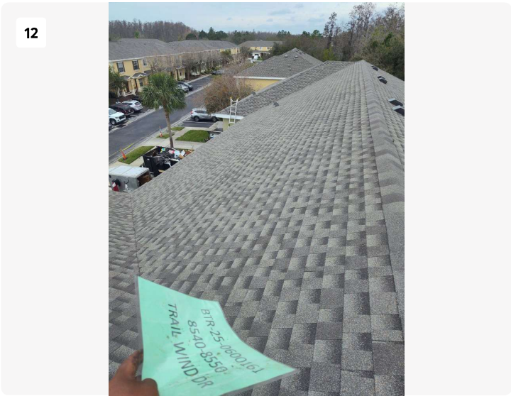
Project: Hammocks 2- Trail Wind 8540-8550 / 2412-6438469-01 Date: Feb 19, 2025, 1:16 PM Creator: Guillermo Cabanas
