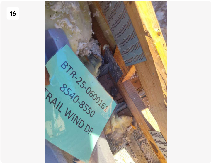
Project: Hammocks 2- Trail Wind 8540-8550 / 2412-6438469-01 Date: Feb 17, 2025, 1:32 PM Creator: Guillermo Cabanas
