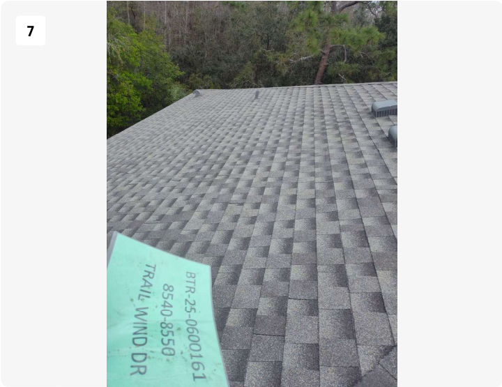
Project: Hammocks 2- Trail Wind 8540-8550 / 2412-6438469-01 Date: Feb 19, 2025, 1:15 PM Creator: Guillermo Cabanas
