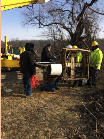
Platform attached to pole
