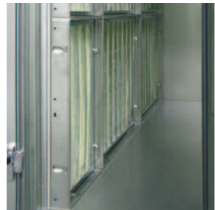
filter frame firmly installed
