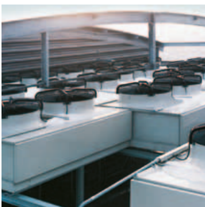
cooling air conveyance by sickle fans
