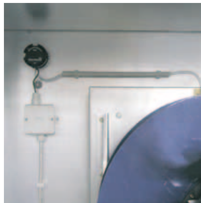
volume flow measuring at the fan
