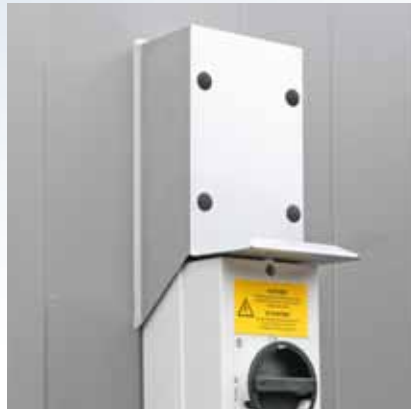
weatherproof cover of repair switch
