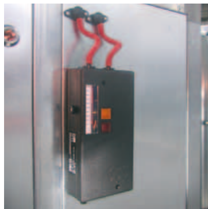
differential pressure manometer (filter supervision)
