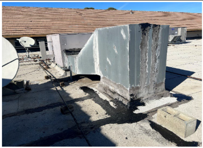
Once the mastic becomes weathered and deteriorated these areas become prone to leaks
