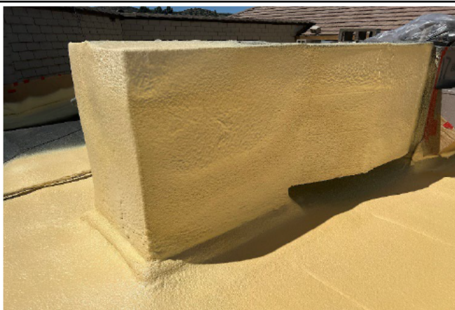
HVAC Ductwork is seamlessly integrated into the roof system removing the most vulnerable areas that are prone to leak
