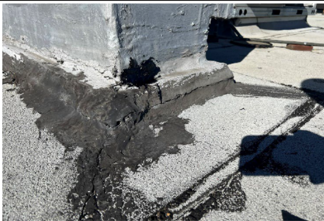
Fractures and splits start accruing in several areas
