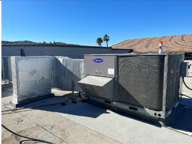
These mechanical metal ductwork connection are sealed with a 3 course mastic seal
