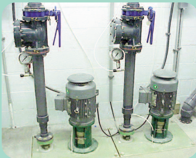
Fybroc Series 5500 Vertical pump installation
