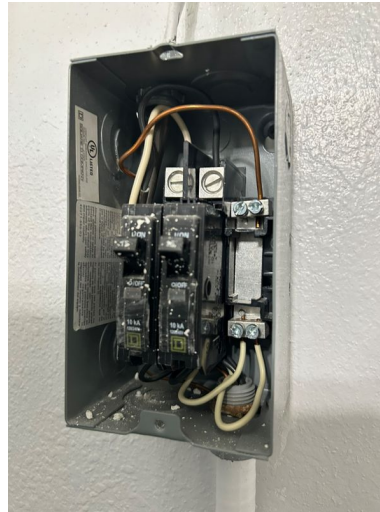
Sub Panel in Laundry Room
