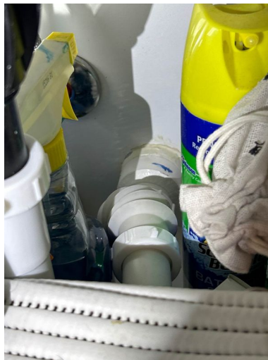
Master Bathroom - both sinks
