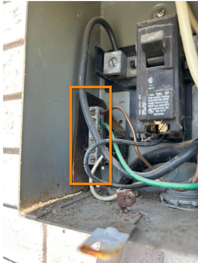
Septic Sub Panel
