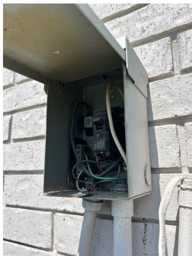
Septic Sub Panel
