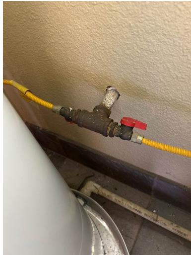
Water Heater Closet
