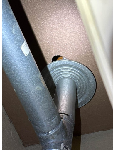
Water Heater Closet
