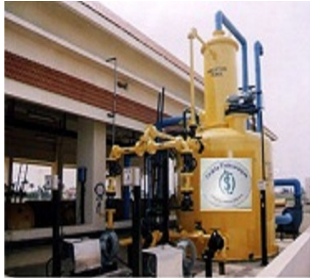
CHLORINE LEAK ABSORPTION SYSTEM
