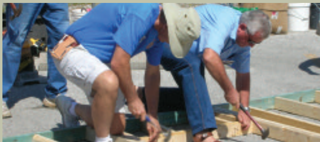
HABITAT, BATSON-COOK, AND ROTARY VOLUNTEERS ERECT THE FIRST "BUILDING HOPE" HOME IN JUST SIX HOURS.
