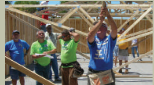
ROTARY AND HABITAT FOR HUMANITY VOLUNTEERS CONSTRUCT THE FIRST HOUSE AT THE "BUILDING HOPE" KICK-OFF.
