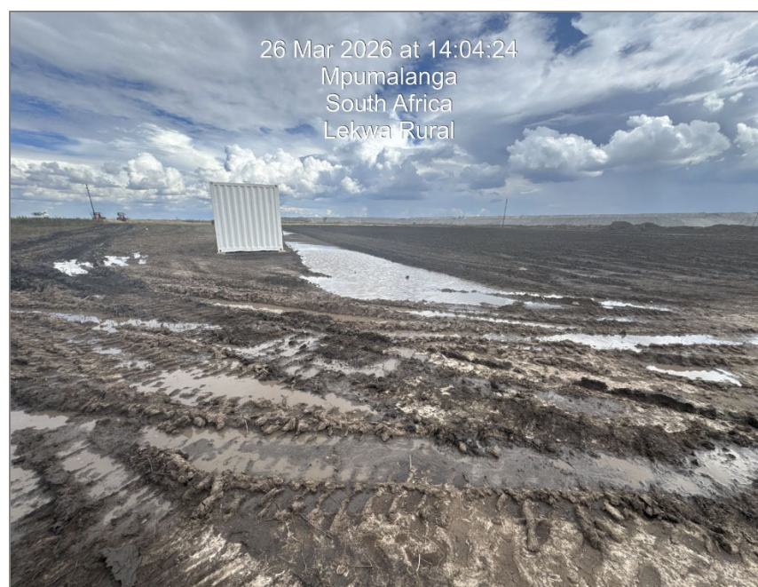
Figure 2: Water ponding at the TSF area
