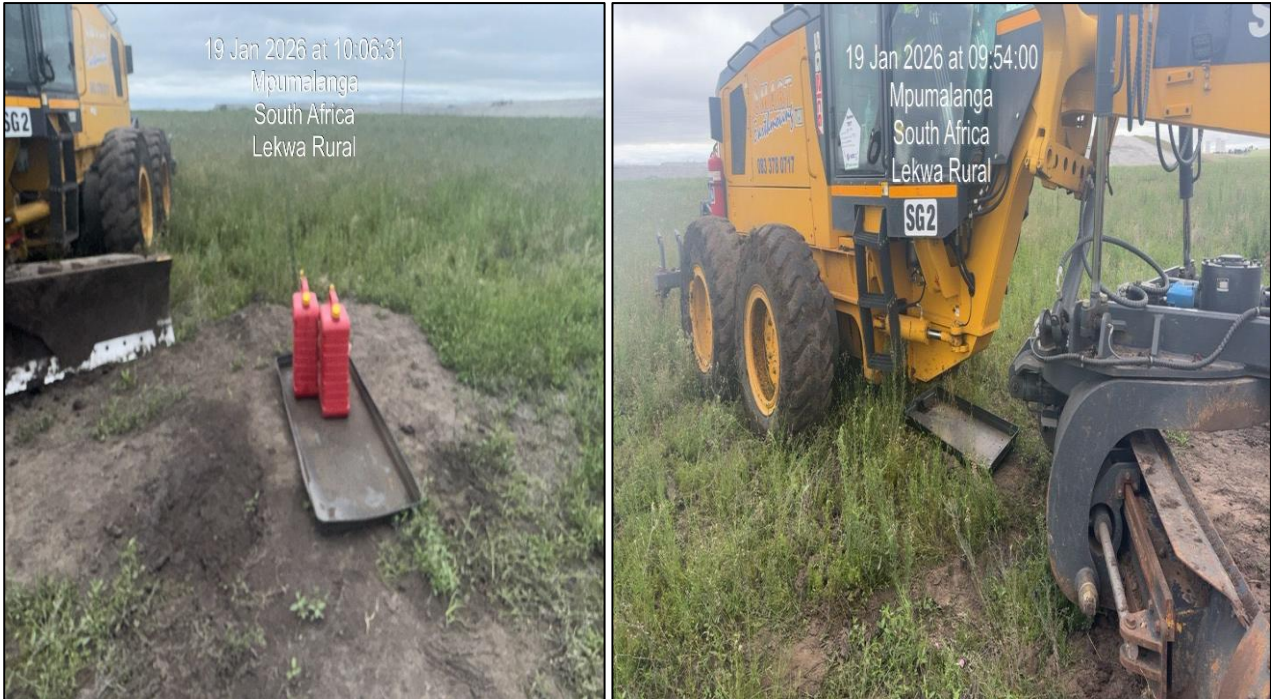
Figure 3: Drip trays in use.
