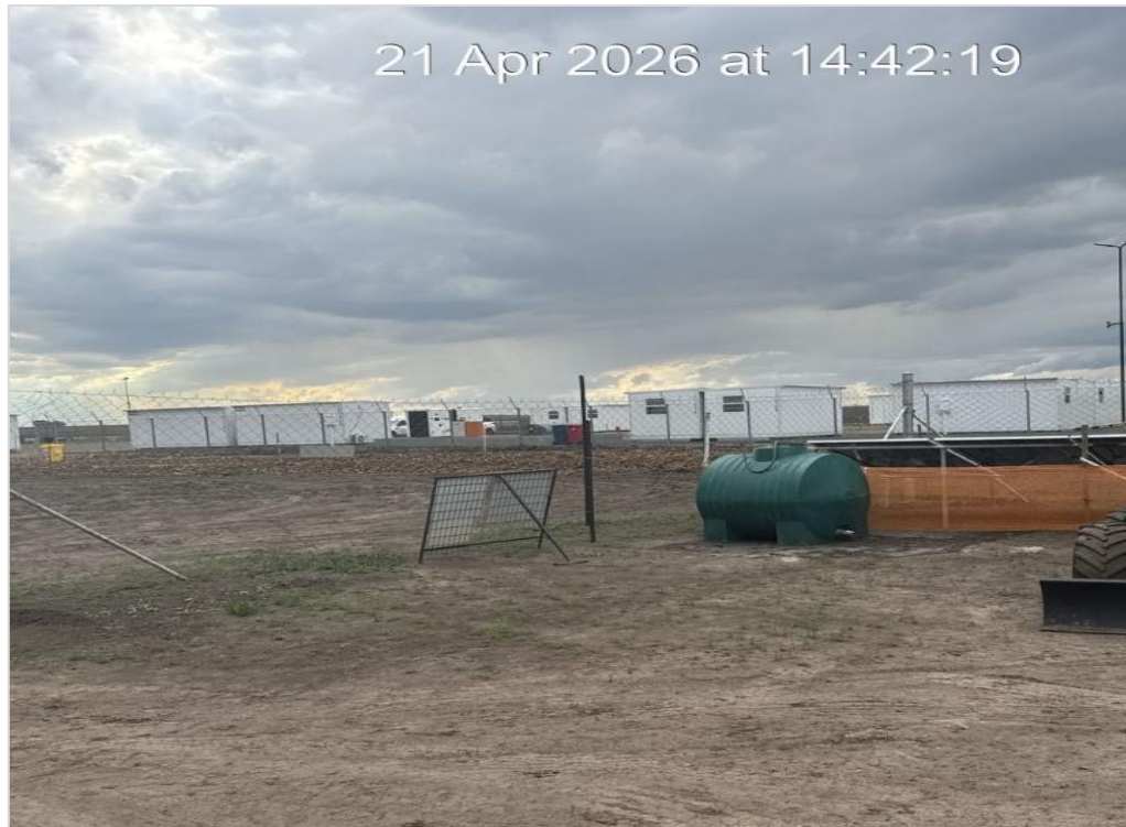
Figure 1: Cement water poured on the ground.
