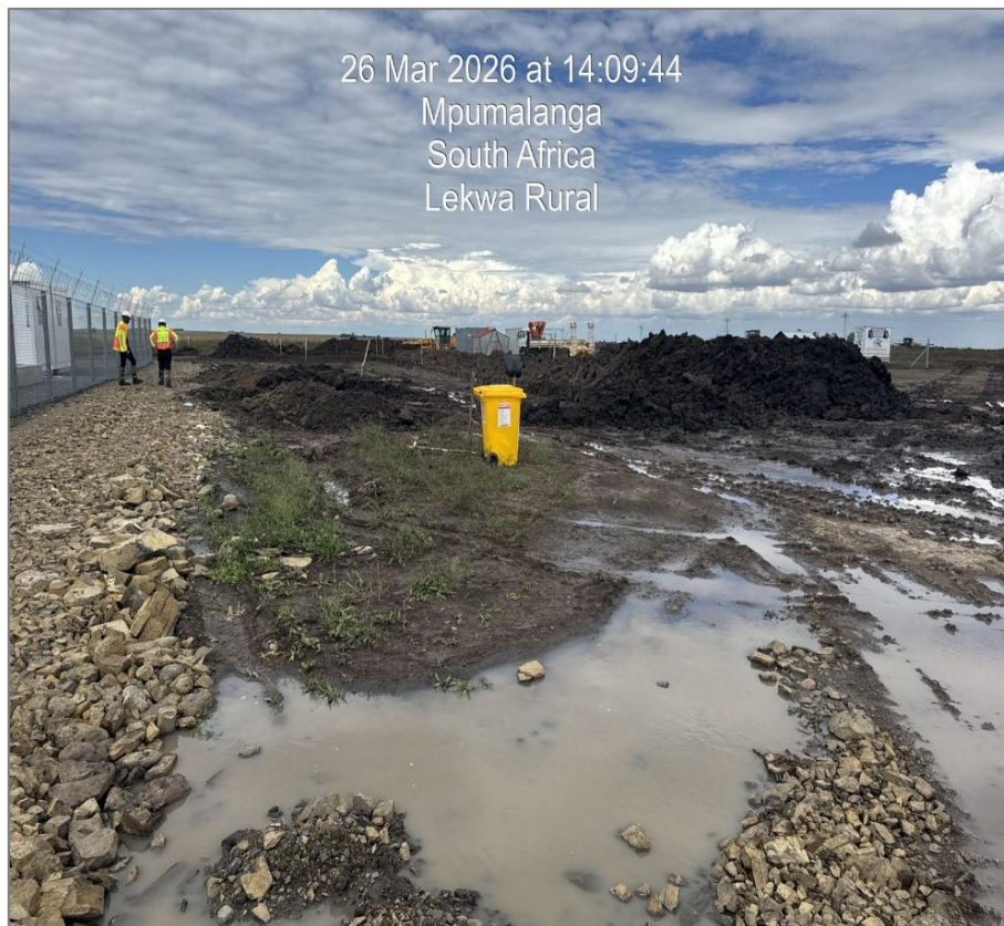
Figure 4: Fencing at the TSF.
