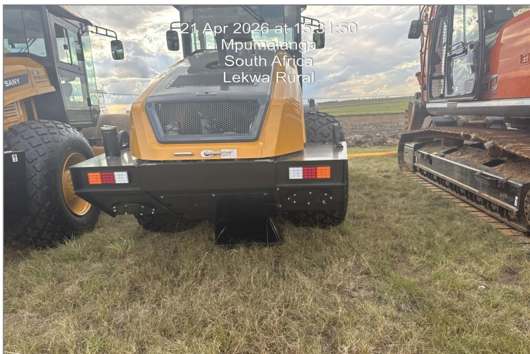
Figure 1: Machines standing with drip trays at the substation.
