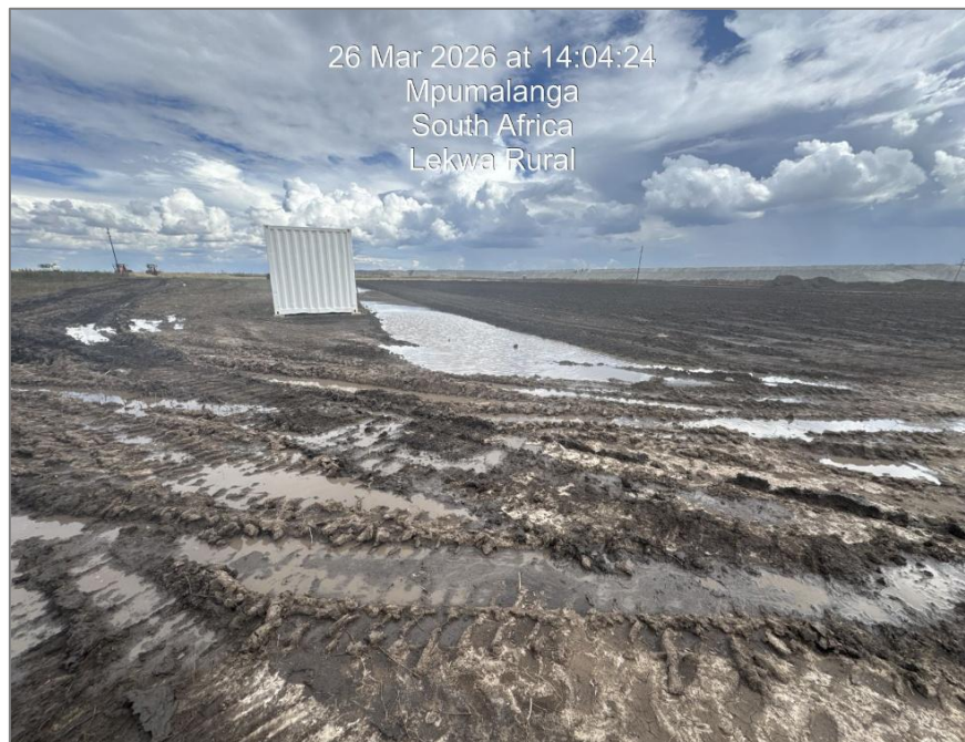
Figure 2: Water ponding at the TSF area
