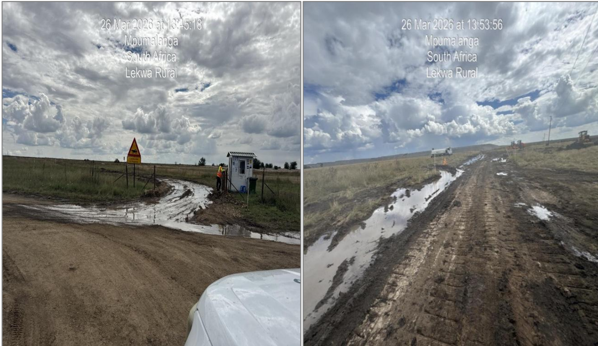
Figure 1: Condition of the access road
