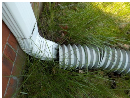
Needs a better extension, water falling at the foundation.
