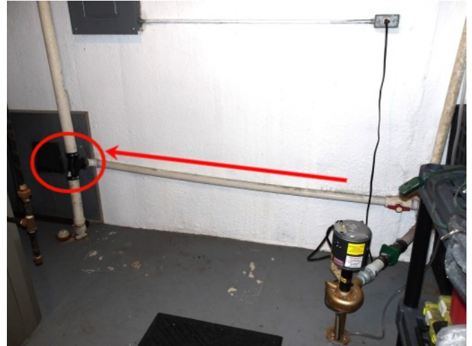
Pump overflow spliced into kitchen drain pipe.
