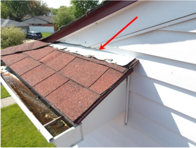
Original gable end flashing damaged from prying nails out from old roof covering.
