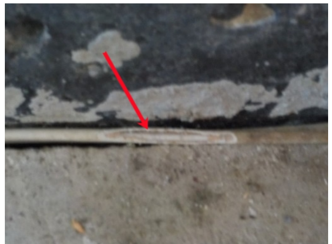
Wire sheathing is worn through
