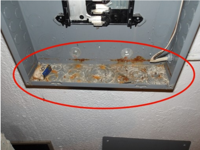
Rust at the bottom of the panel housing.
