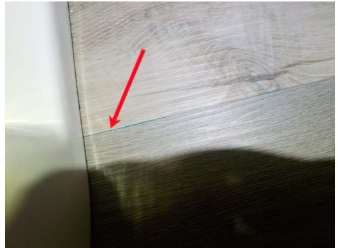
Blue color in floor, potential leak area.
