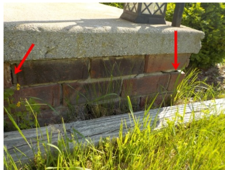
Areas of missing or gapped mortar
