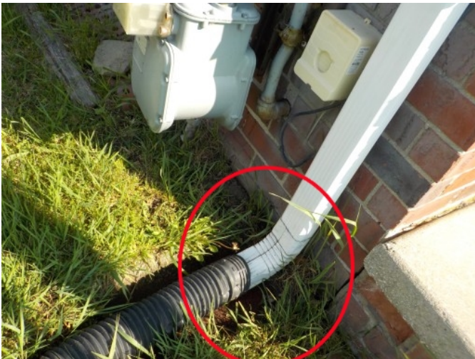
Low area against the foundation.
