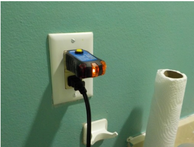
Loose outlet, old GFCI outlet.
