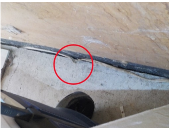
Wire is creased/bent
