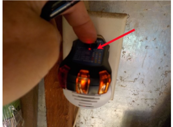
No GFCI protection
