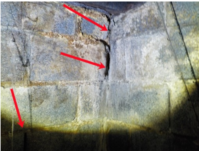
Mortar gaps in firebox
