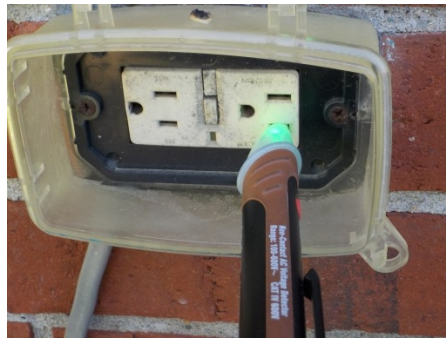
Requires replacement, showing no power.
