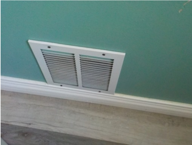
Heat vent has a cold air return cover, no airflow adjustment
