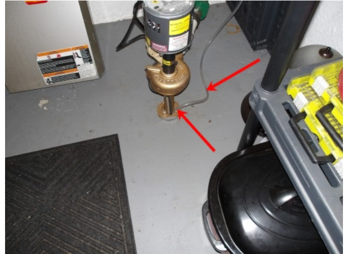
Condensate drain tube terminates into the sump crock.
