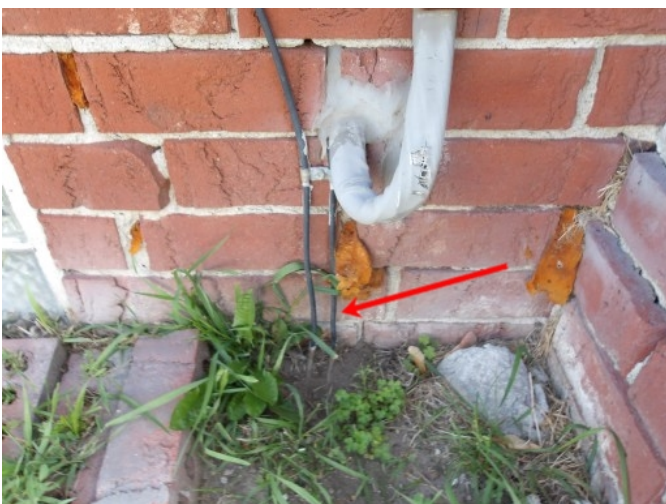
Earth rod ground wire
