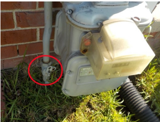
Gas shut-off valve.
