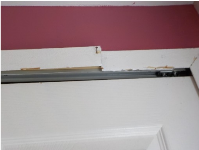
Damage to bedroom door molding.
