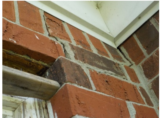
Exterior, brick shows movement.
