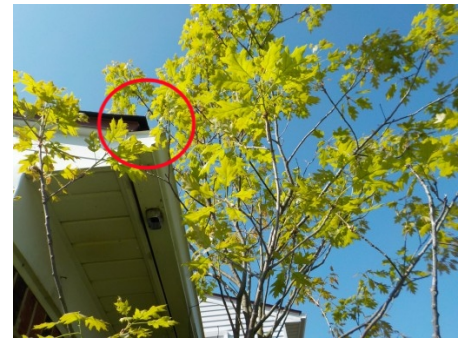
Gutter runs short of the roof length.
