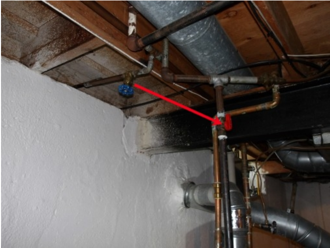
Water heater gas supply shutoff valve
