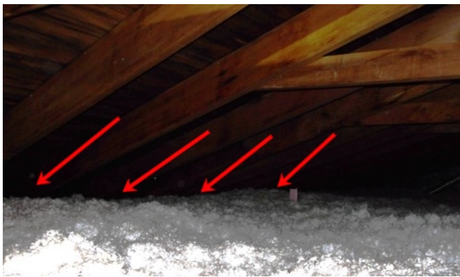
Difficult to see in image, but insulation is filled to soffit areas.
