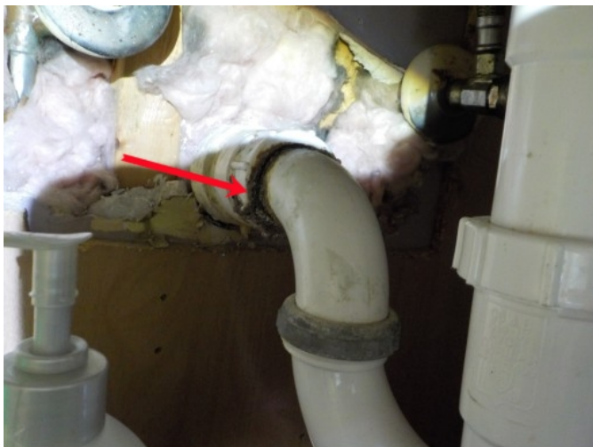
Mineral deposits/build-up at connection may suggest a slow leak.
