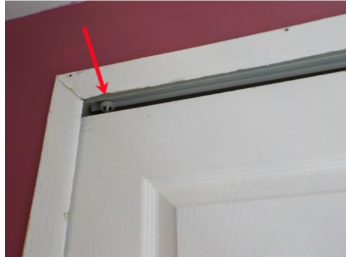
Track wheel needs to be adjusted, rides along molding.
