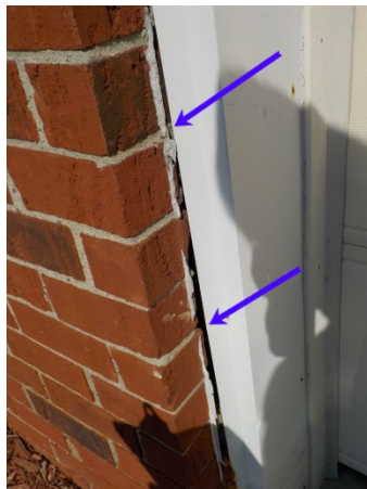
Wall at garage trim has pulled away
