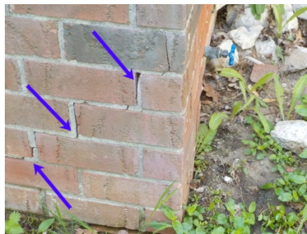
Step crack at North corner
