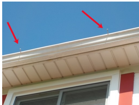
Nails need to be pounded in on upper gutter.
