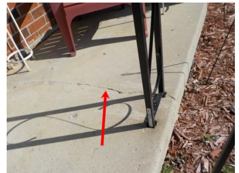
Cap has cracked
