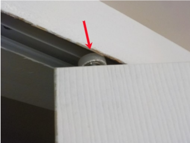
Hallway closet - wheel needs adjustment to stay in track.
