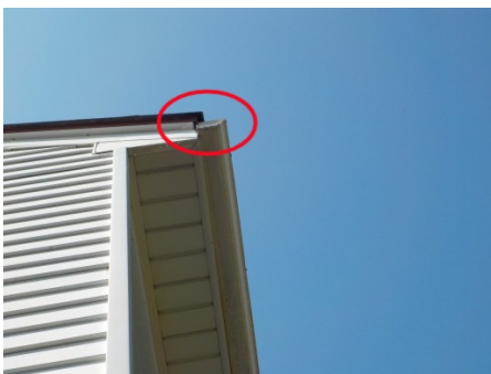
Gutter should run past corner.
