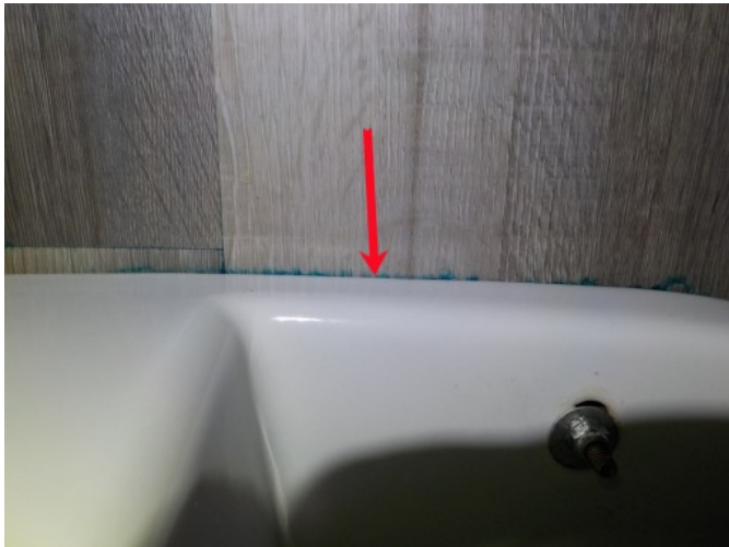
Blue color likely a sign of toilet leak at the base.
