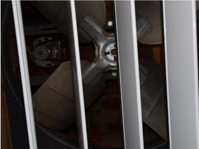
Whole house attic fan as seen from the hallway.
