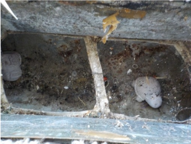
Family room register needs cleaning.
