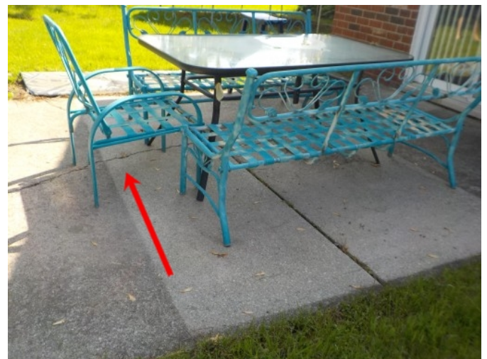
Cracked slab but no major movement or heaving of concrete present.
