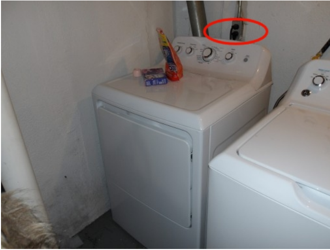
Washer / dryer outlet is required to be GFCI protected.
