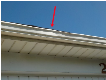
Damaged gutter above garage.
