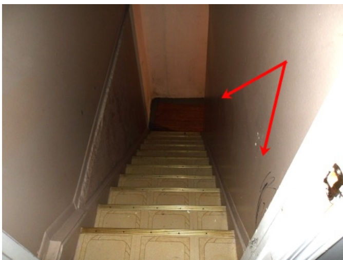
Requires hand rail
