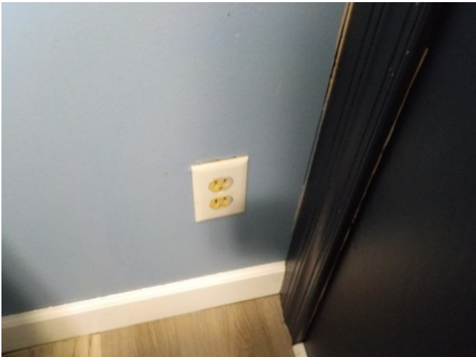
Loose outlet - should be GFCI protected as well.
