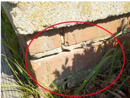
Loose or missing mortar.
