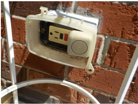
Requires a protective weather cover (porch)
