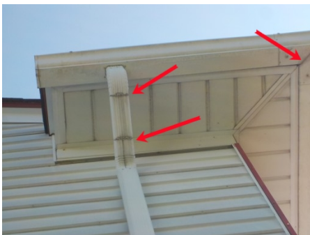
Stains can suggest potential areas of leaks, monitor during rain.
