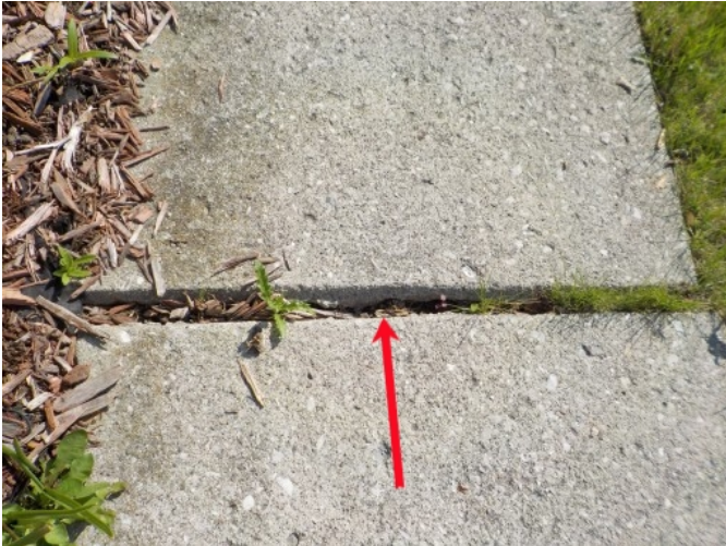
Wide expansion gaps present on walk to porch.
