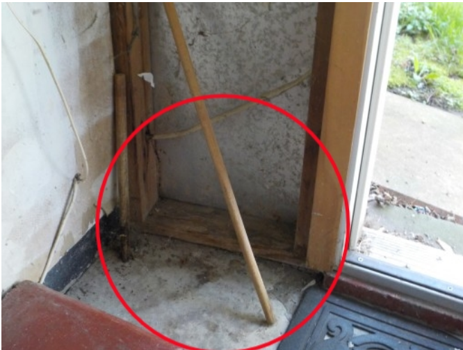
Interior wall shows movement.
