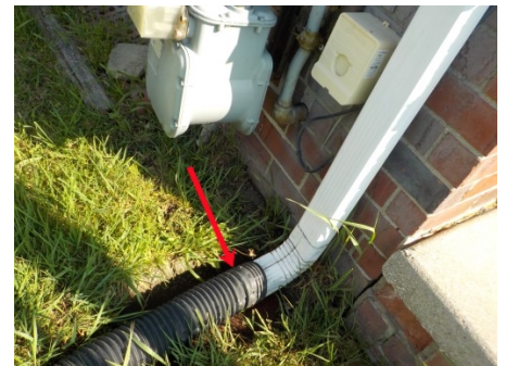
Appears water is falling out of the plastic extensions here.
