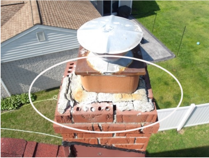
Furnace / water heater chimney crown is age deteriorated.
