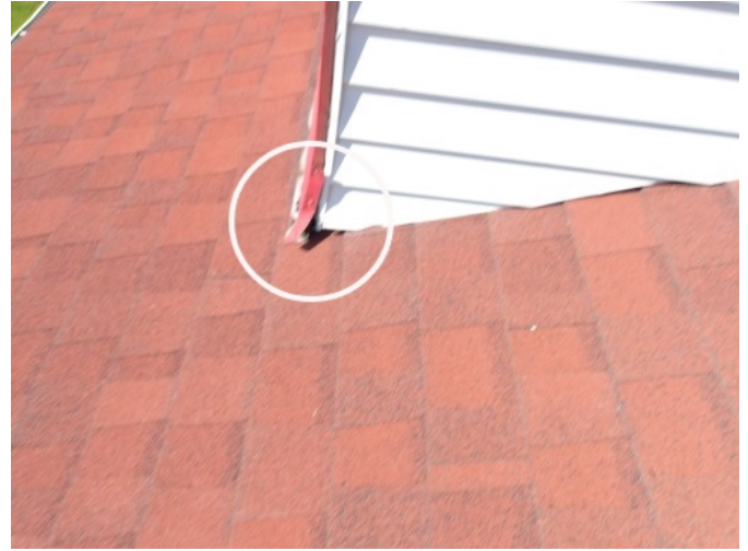
Corner trim damaged at east side corner at the garage.
