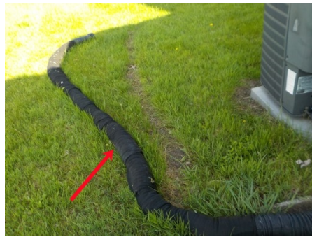
Extension is too long, too many turns.
