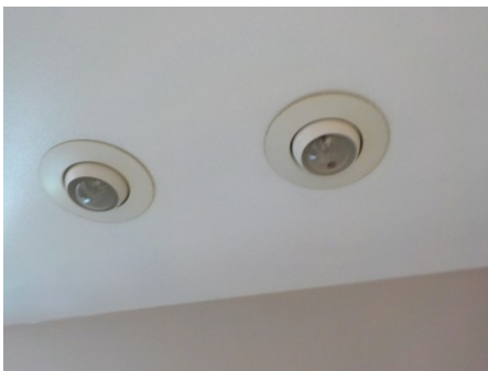
No power to lights above the sink.
