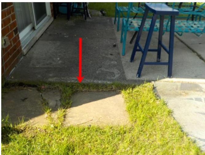
Potential trip hazard at this point
