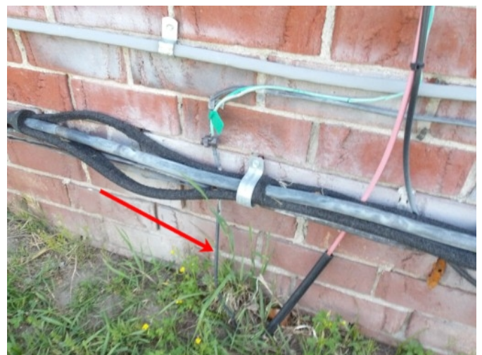
Second earth rod ground
