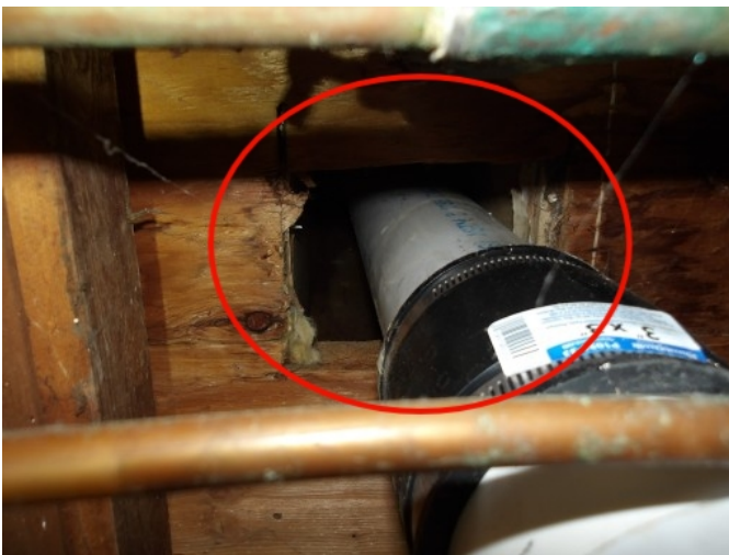
Fireblock / close opening around the main waste line.
