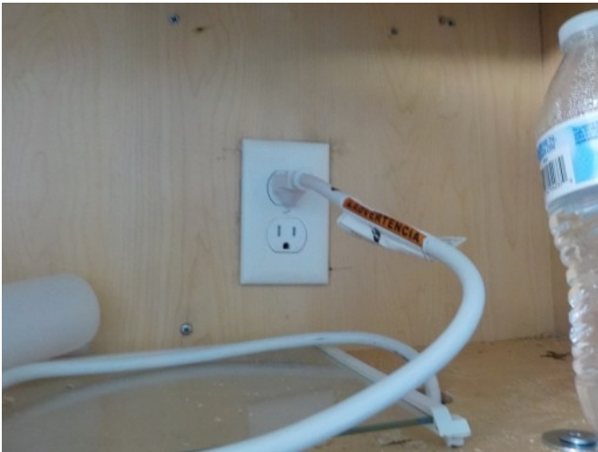
Loose outlet - in cabinet above microwave.
