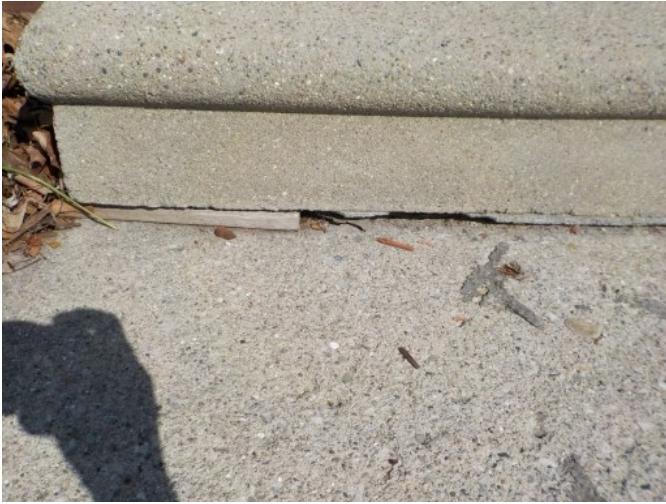
Step is wobbly when walked on, not properly supported.
