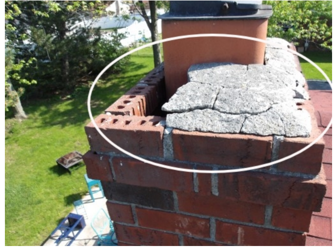
Fireplace chimney crown is age deteriorated.
