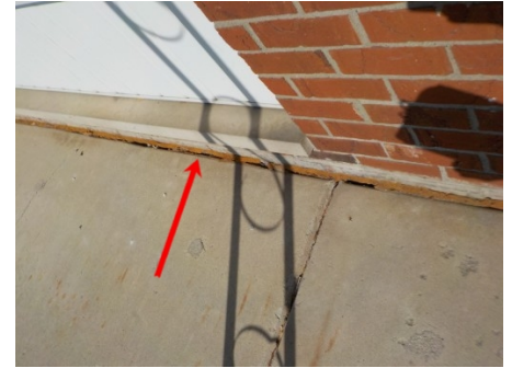
Evidence of movement/separation from structure
