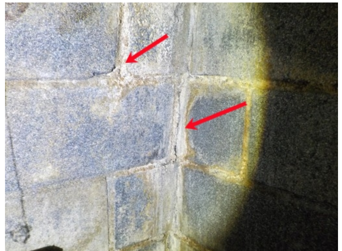
Small cracks will also need repair
