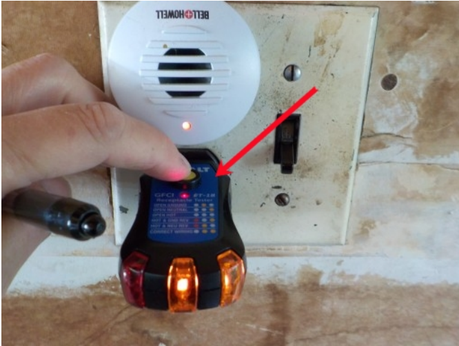
There is no GFCI protection on all wall outlets.
