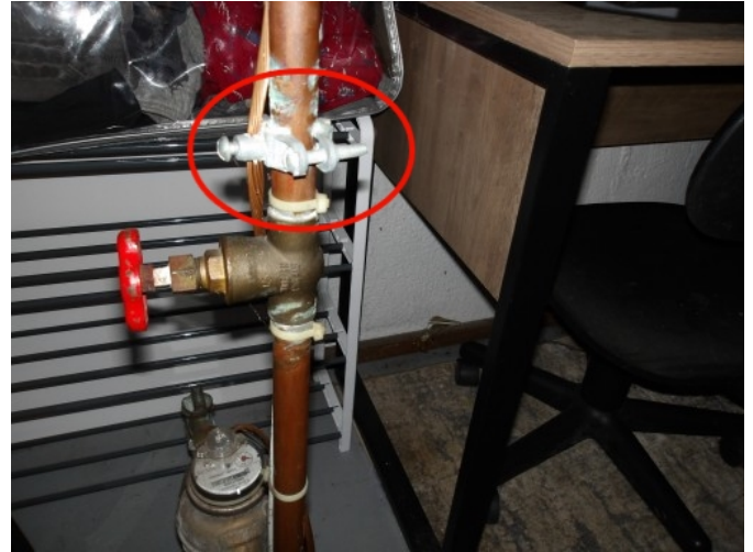
Ground clamp before water meter.
