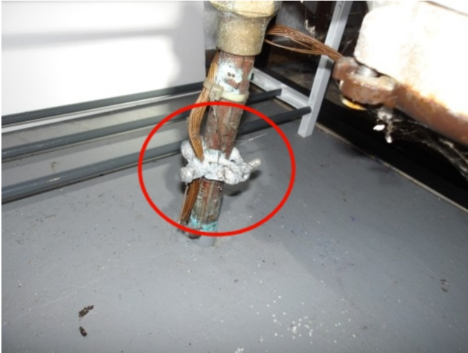
Corroded ground clamp at incoming copper water line.
