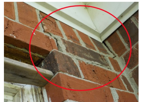
Movement of brick at garage service door.
