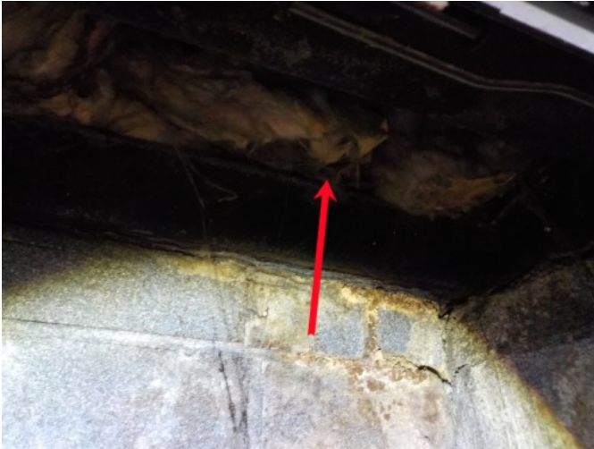
Smoke chamber is stuffed with insulation
