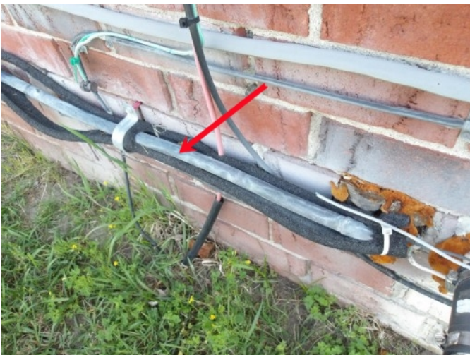
Insulation is deteriorated.
