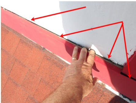
Loose trim needs sealing
