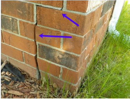
Garage corner has shifted
