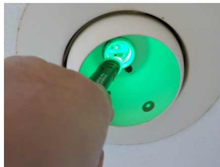
Tester shows no power (green) to light with switch on.
