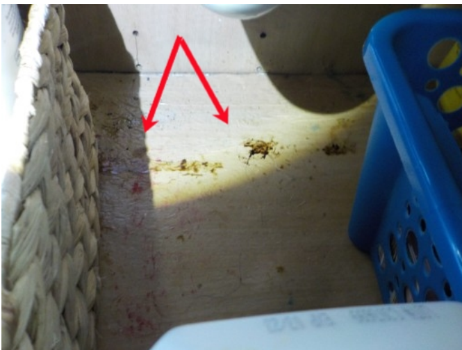
Possible moisture damage and stains.
