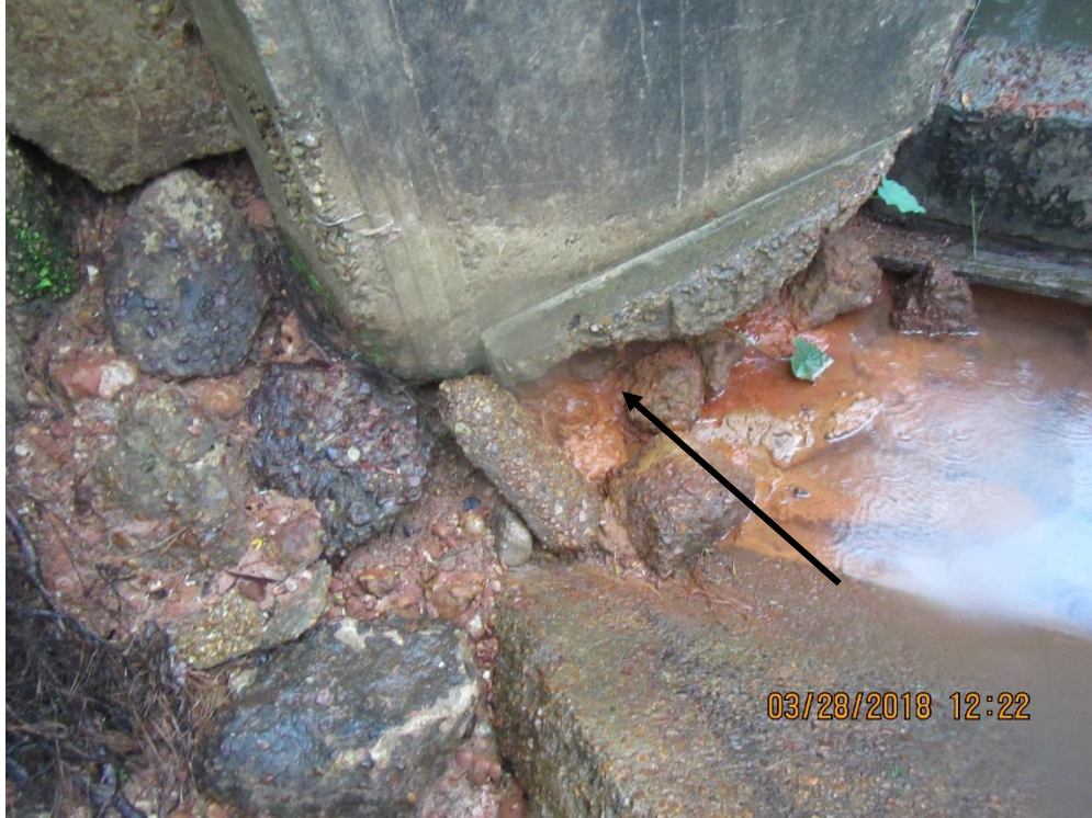
Photo 11: Standing at the end of the right end wall looking southwest; a view of the seepage discharging from under the end wall (Arrow).
