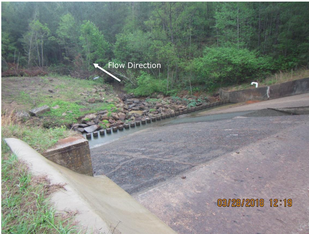
Photo 10: Standing on the left side wall of the spillway control section; a view of the concrete discharge slab and riprap lined earthen channel.
