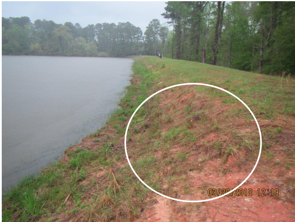
Photo 5: Standing on the right end of the upstream slope looking northwest; a view of the slope that lacked a vegetated cover and exhibited some minor surface erosion (circled).
