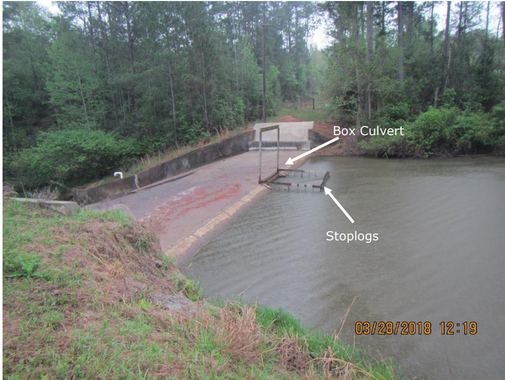
Photo 9: Standing to the left of the spillway inlet looking southeast; a view of the spillway and box culvert inlets.
