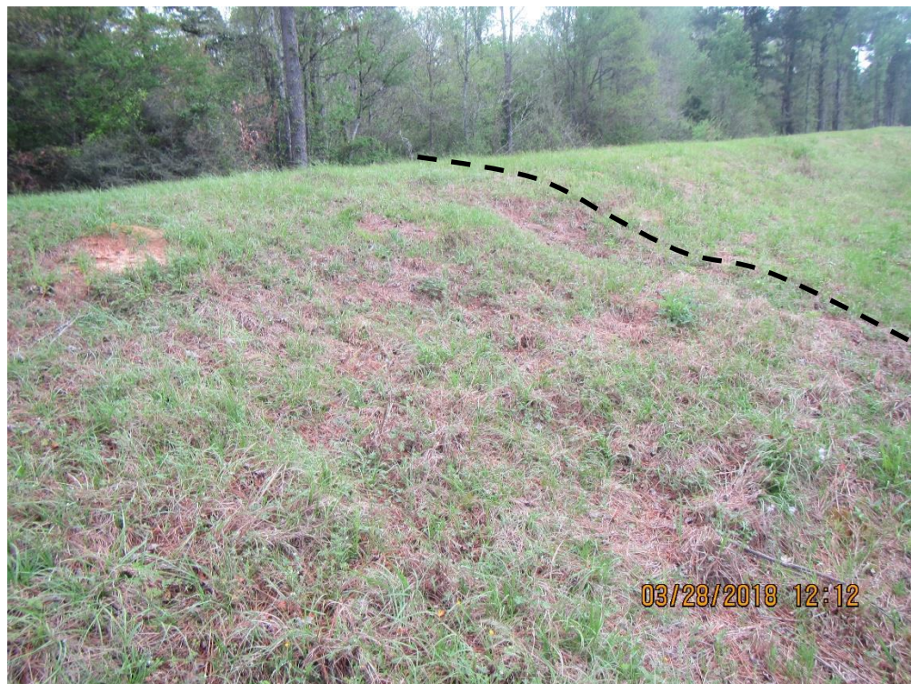
Photo 6: A view of a minor erosion rill (dashed-line) noted along the upstream slope.
