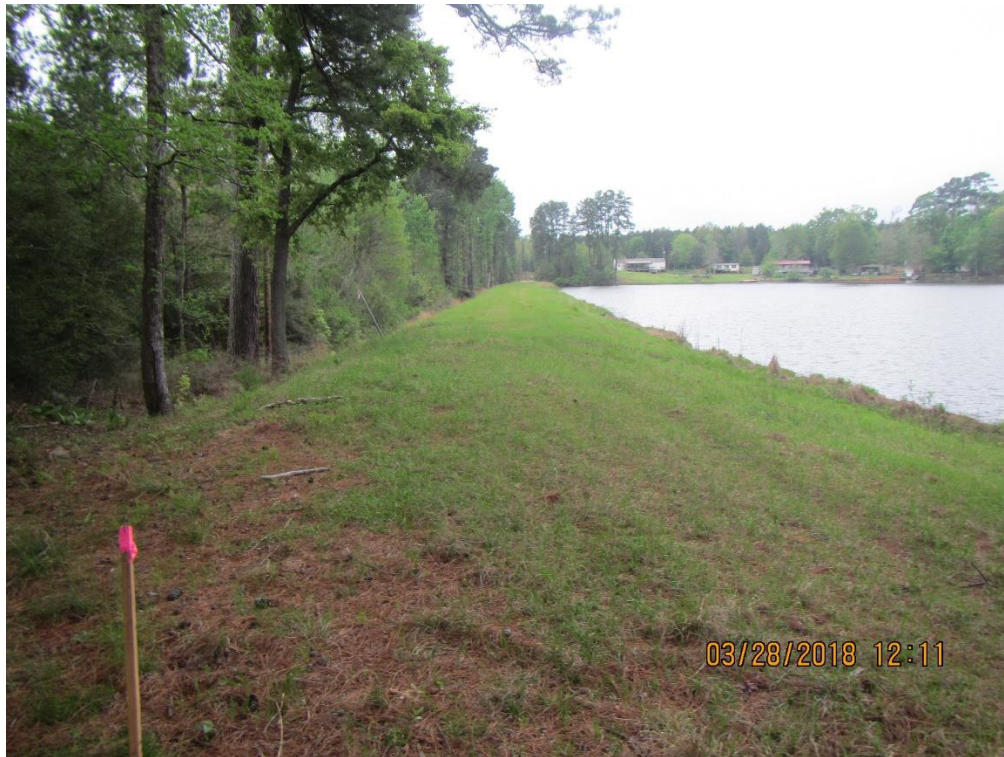
Photo 1: Standing on the left end of the dam looking southeast; a typical view of the well-maintained vegetated cover along the crest.
