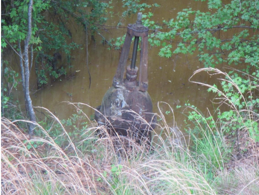
Photo 15: Standing on the downstream slope looking northeast; a view of the reservoir drain valve located along the downstream toe. Note the standing water within the discharge channel of the drain.
