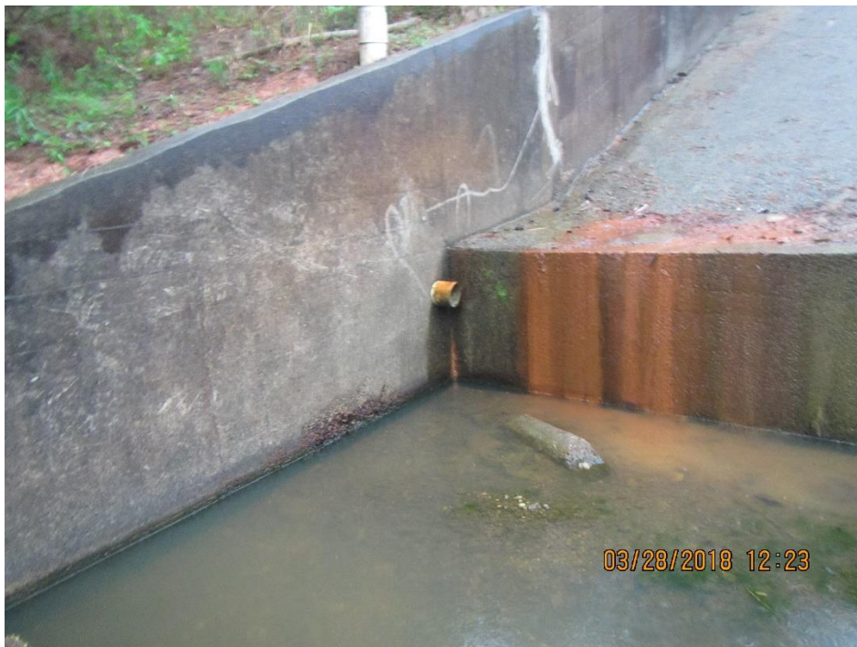
Photo 12: Standing just downstream of the spillway discharge basin looking southwest; a view of one of the 4-inch diameter pipes exiting the sidewalls of the spillway channel.
