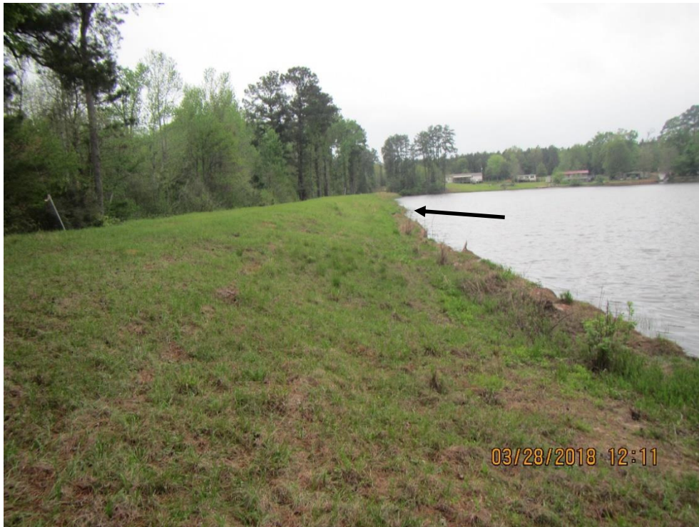
Photo 3: Standing on the left end of the dam looking southeast; a view of the 3H:1V vegetated portion of the upstream slope. Note the approximate location of the bulge is depicted by the arrow.
