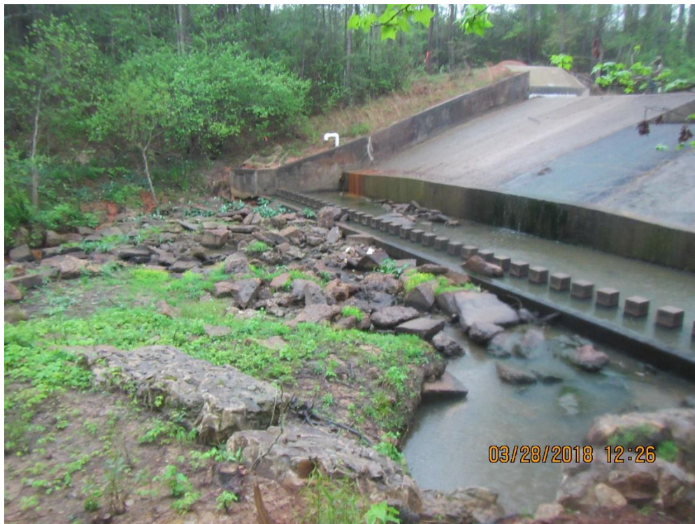
Photo 14: Standing just downstream of the spillway looking south; a view of the riprap lined channel. Note the areas where the riprap was displaced causing erosion and voids within the channel.
