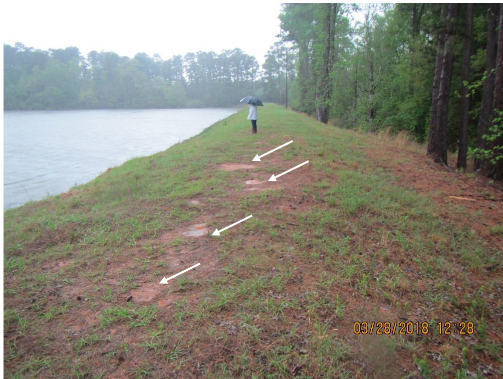
Photo 2: Another view of the crest from the right end of the dam looking northwest. Note the minor bare areas (arrows) randomly along the crest.
