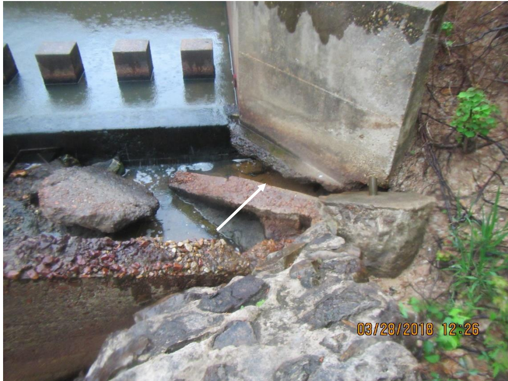
Photo 13: Standing just downstream of the left side wall of the spillway channel looking west; a view of the undermined end wall (arrow).
