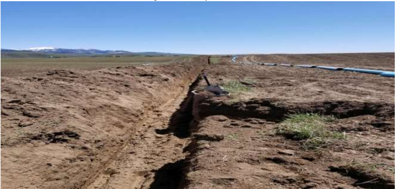
Photo 4. This Photo shows mainline laid out along a trench ready for installation. BLD Photos.
