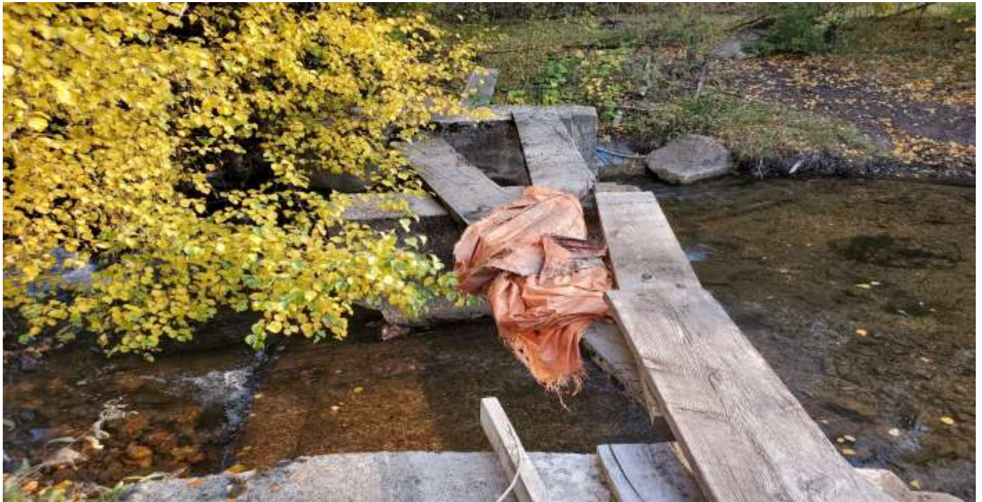
Below: A view lookin from North to South across the old St Charles Diversion Structure. BLD Photos.
