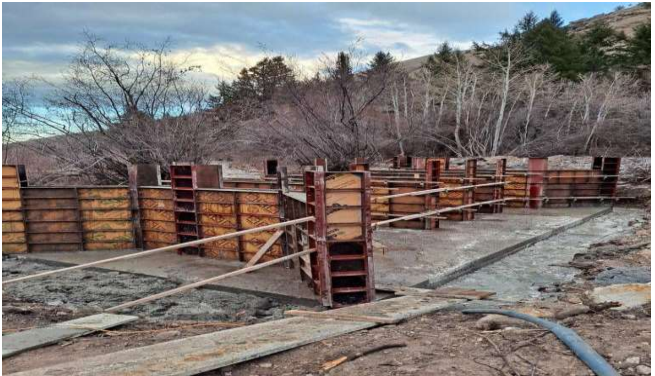
This photo shows the forms as they were set in place to pour the diversion structure on St Charles Creek. BLD Photos.
