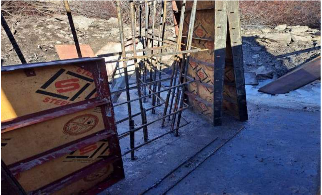
This photo shows the forms set in before the cement pour and how the openings for water flow were established. BLD Photos.
