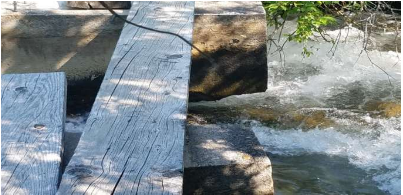
The Old St Charles Diversion Structure was washing out from the downstream side. In the above photo it is visible to see how one of the pillars of the structure was no longer connected to its base. BLD Photos.
