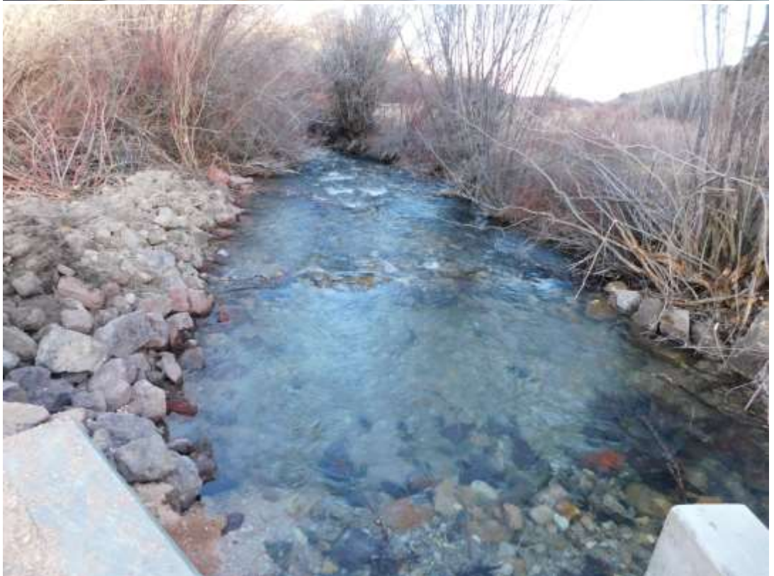
These two photos show the two channels as they spit from the newly installed diversion. The top photo show the irrigation canal and the lower photo shows the main channel. Two step pools were installed below the diversion to be able to slow the water enough for BCT to travel up and down the stream. BLD Photos.
