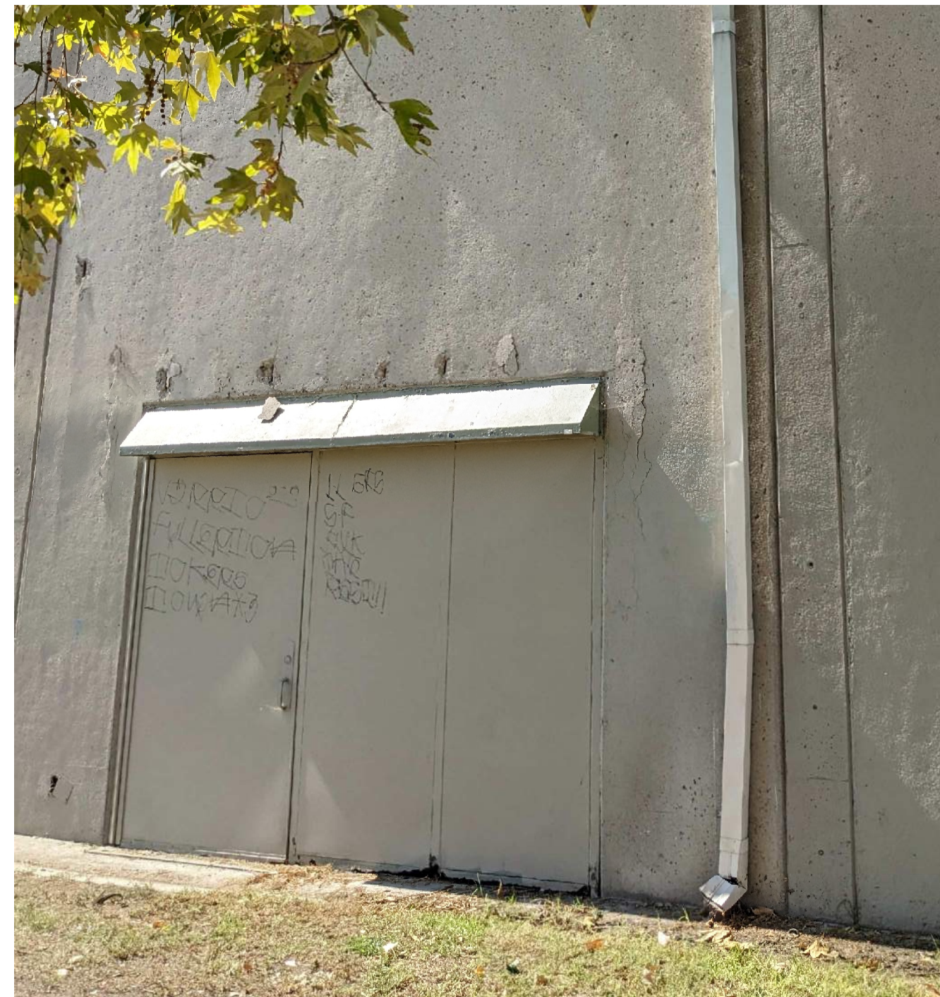
PHOTO OF ENLARGED EAST ELEVATION WHERE SPALLING OCCURS SCALE: N.T.S.
