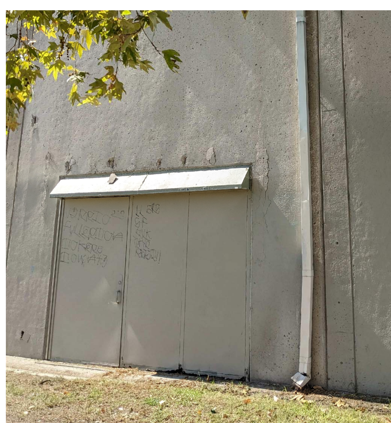
PHOTO OF ENLARGED EAST ELEVATION WHERE SPALLING OCCURS SCALE: N.T.S.
