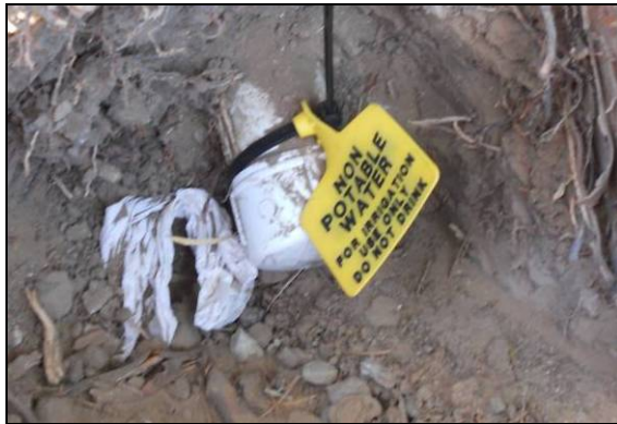
Non-potable water identification tag (yellow)
