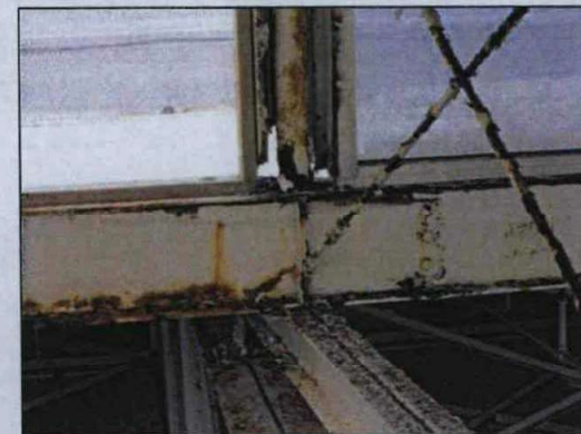
Photo 32. Severely corroded tie-rods.
