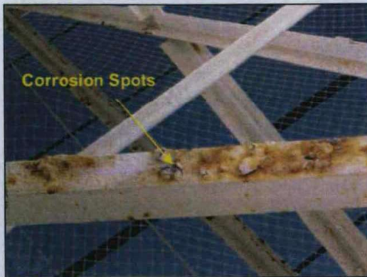
Photo 15. Corrosion spots on diagonal truss members.
