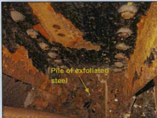
Photo 9. Base of column at Location 1 with massive pile of exfoliated steel at base.
