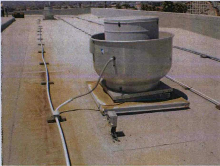
Figure 6. Exhaust Fan (Typical of 6)
