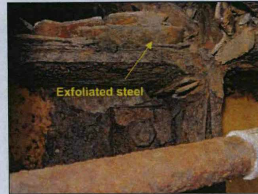
Photo 12. Intermediate moment frame connection at Location 4 with exfoliated steel at top of beam.
