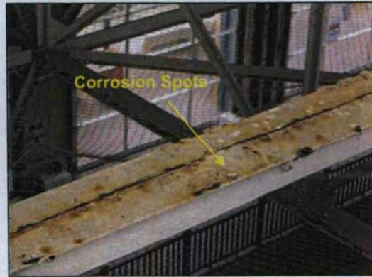
Photo 18. Corrosion spots on top chord truss members.
