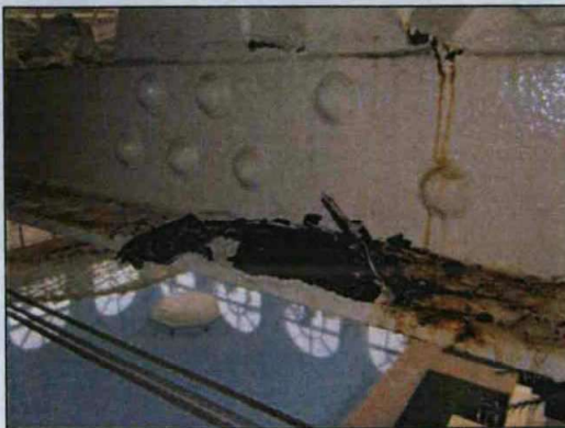
Photo 17. Corrosion spot on bottom chord truss members with minor pitting.
