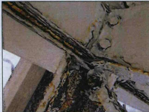
Photo 29. Detail of typical exfoliation of beam flanges at connection point between top longitudinal and transverse beams.
