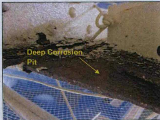
Photo 19. Bottom chord gusset plate with moderate pitting.
