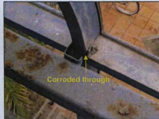
Photo 24. Lateral-brace tube bracket corroded through.
