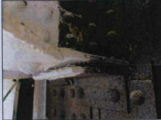
Photo 8. Intermediate level column-beam connection at Location 1 with pitted steel.
