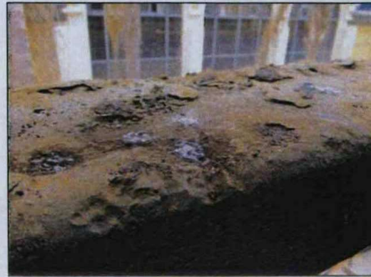
Photo 22. Detail of corrosion nodules on lateral-brace tube after removal of corrosion products (weakened steel).
