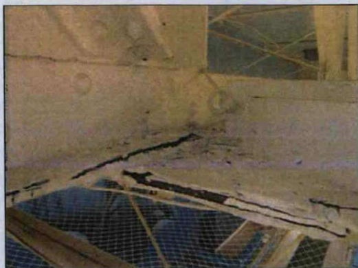
Photo 3. Delaminating white coating on truss frame, corrosion underneath coating.
