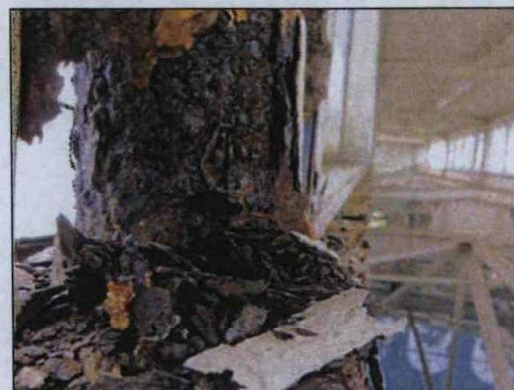
Photo 31. Pipe column in Bay 6 corroded through about 270 degrees of circumference.
