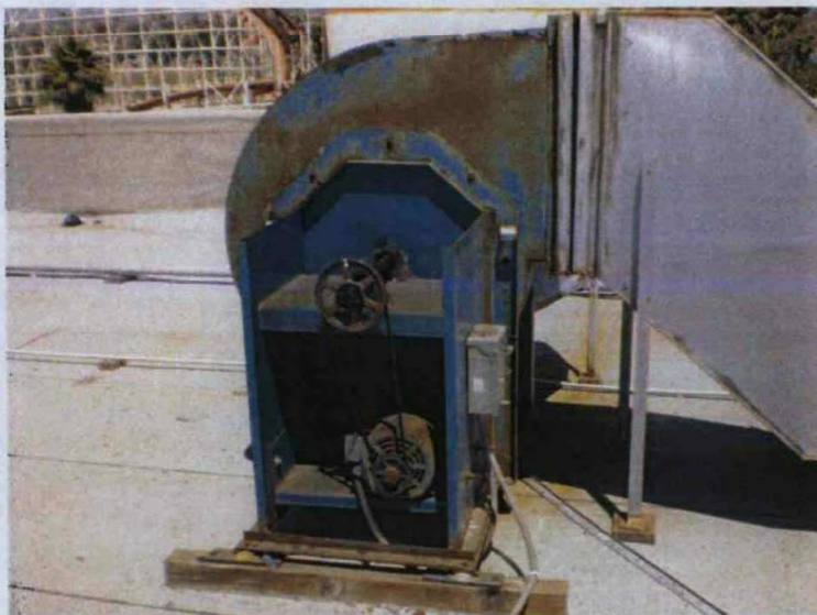
Figure 4. Supply Fan (Typical of 2)
