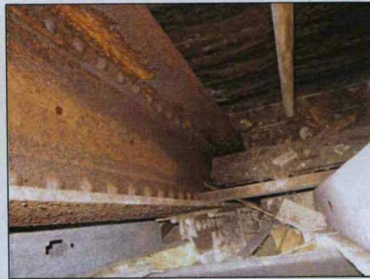
Photo 6. Column at Location 1, looking down at intermediate level beam connection.
