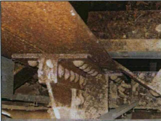
Photo 7. Intermediate level column-beam connection at Location 1 with pitted steel.
