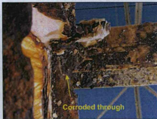
Photo 26. Bottom longitudinal beam and bottom transverse beam severely exfoliated steel. Bay 2 shown.
