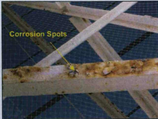
Photo 15. Corrosion spots on diagonal truss members.
