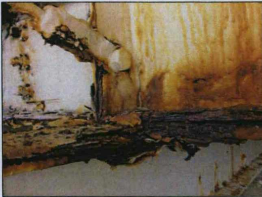
Photo 27. Typical exfoliation of beam flanges at bearing point between bottom longitudinal and transverse beams.
