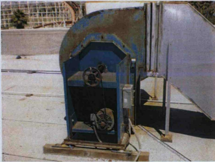
Figure 4. Supply Fan (Typical of 2)
