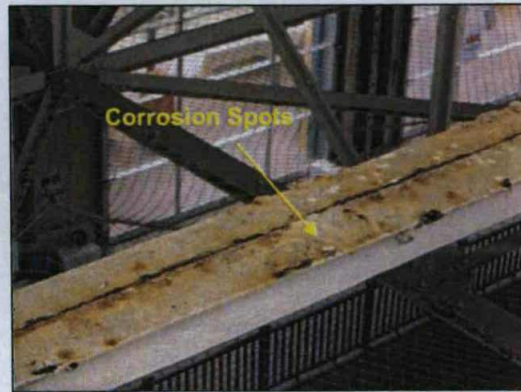
Photo 18. Corrosion spots on top chord truss members.
