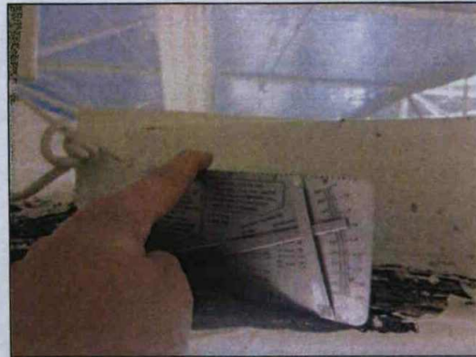
Photo 20. Bottom chord gusset plate pit-depth measurement at approximately 0.150 inches deep.
