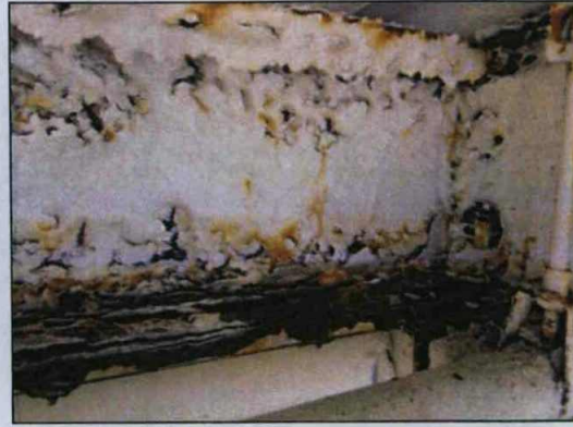
Photo 4. Peeling white coating on clearstory frame, corrosion underneath coating.
