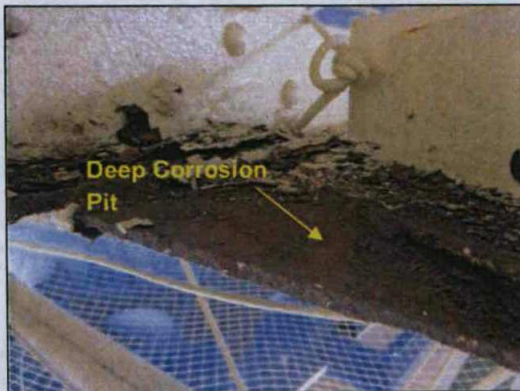
Photo 19. Bottom chord gusset plate with moderate pitting.
