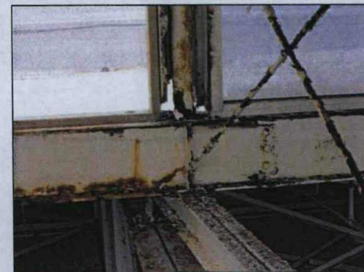
Photo 32. Severely corroded tie-rods.
