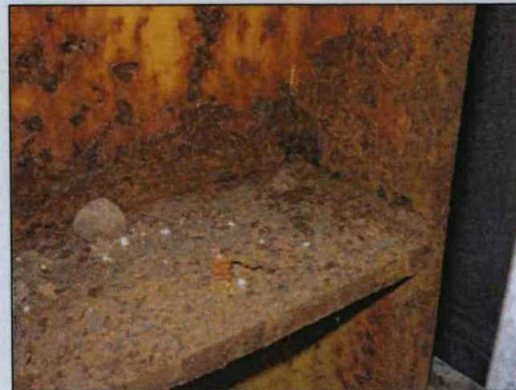
Photo 11. Intermediate moment frame connection at Location 4 with pitting in panel zone.
