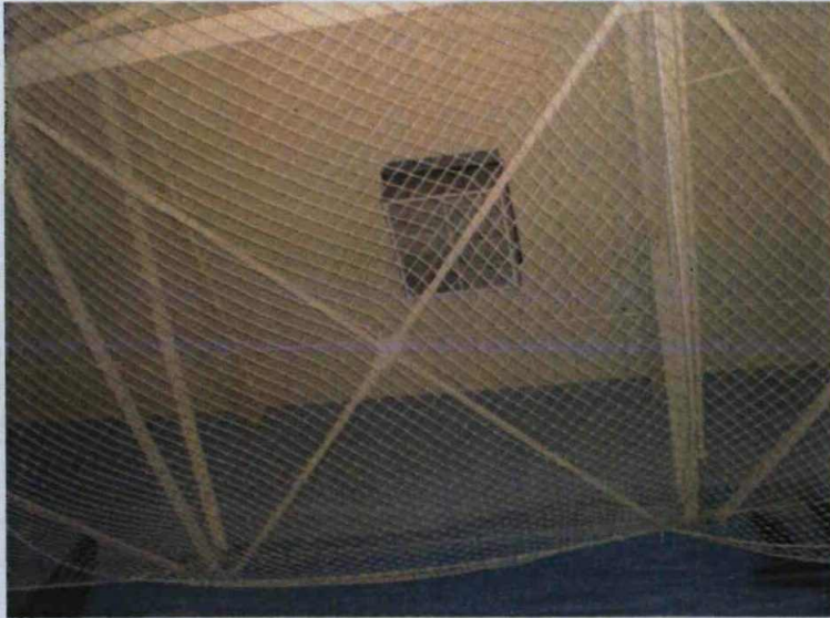
Figure 9. Supply Air Grille
