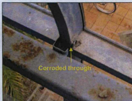
Photo 24. Lateral-brace tube bracket corroded through.
