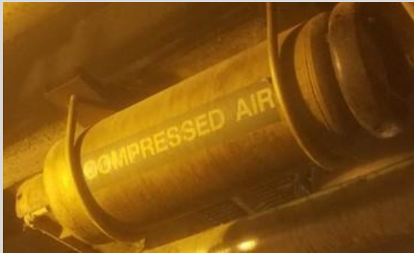
External air reservoir connected to actuator in picture below.
