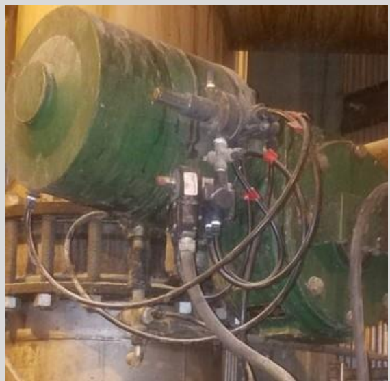
Complex ad-hoc piping and integration with various components to achieve fail-safe with external air reservoir.
