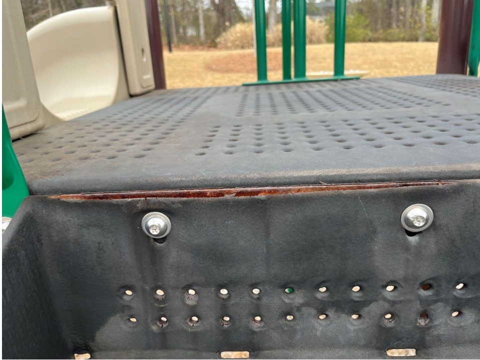
17. View of corroded stairs at tot lot.
