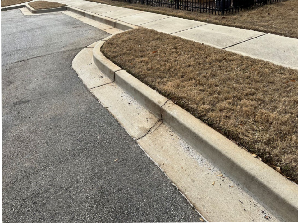
3. View of linear crack at section of curb in amenity area lot.
