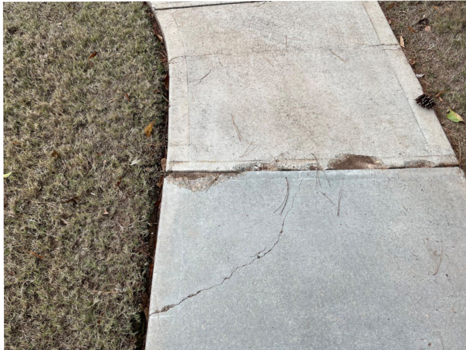
4. View of linear crack at sidewalk near pool and clubhouse.
