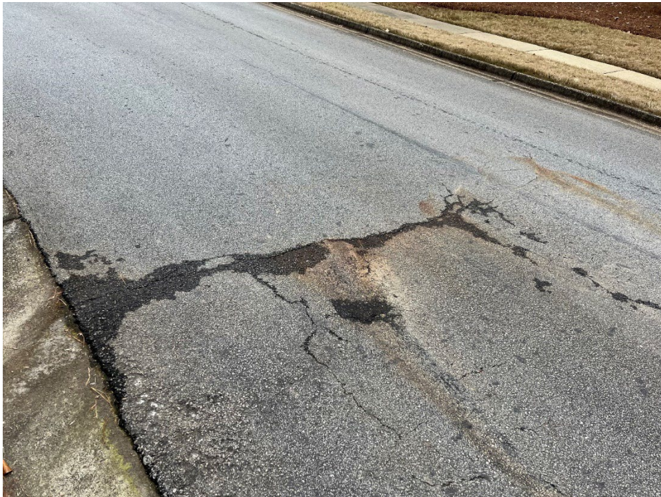
2. View of linear cracks in private roads near guard house.
