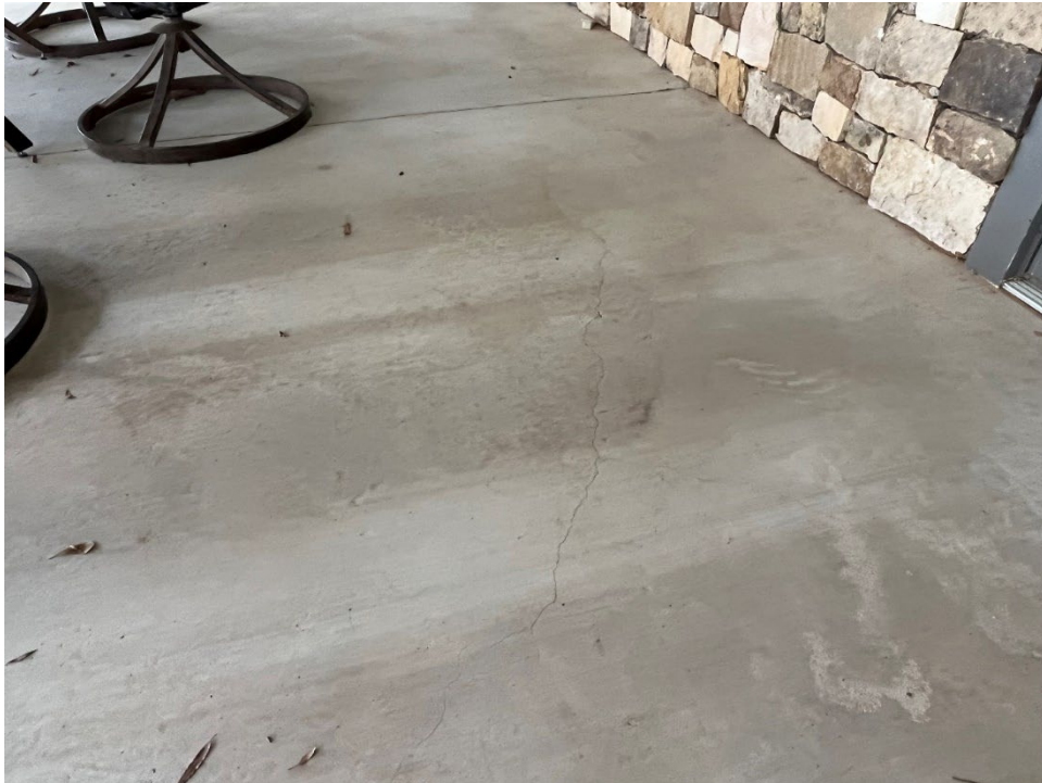
12. View of linear crack at pool deck area
