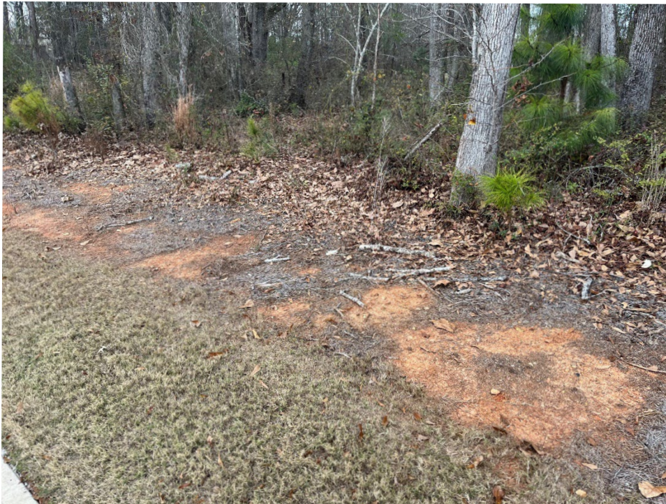
10. View of area with erosion and exposed soil near community garden.
