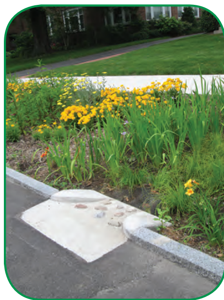
Energy dissipater between road and bioretention.
