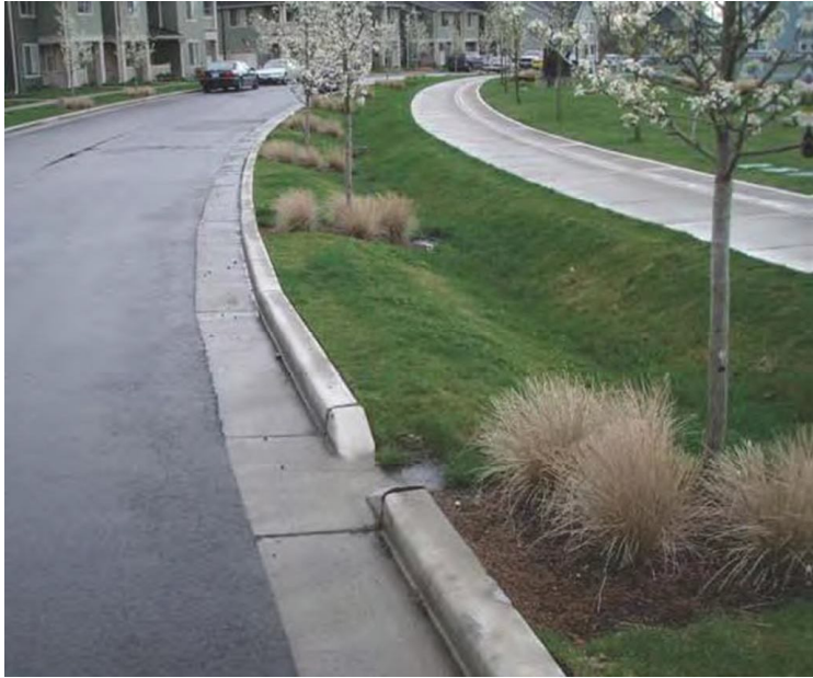
Curb opening to grass swale in residential development
