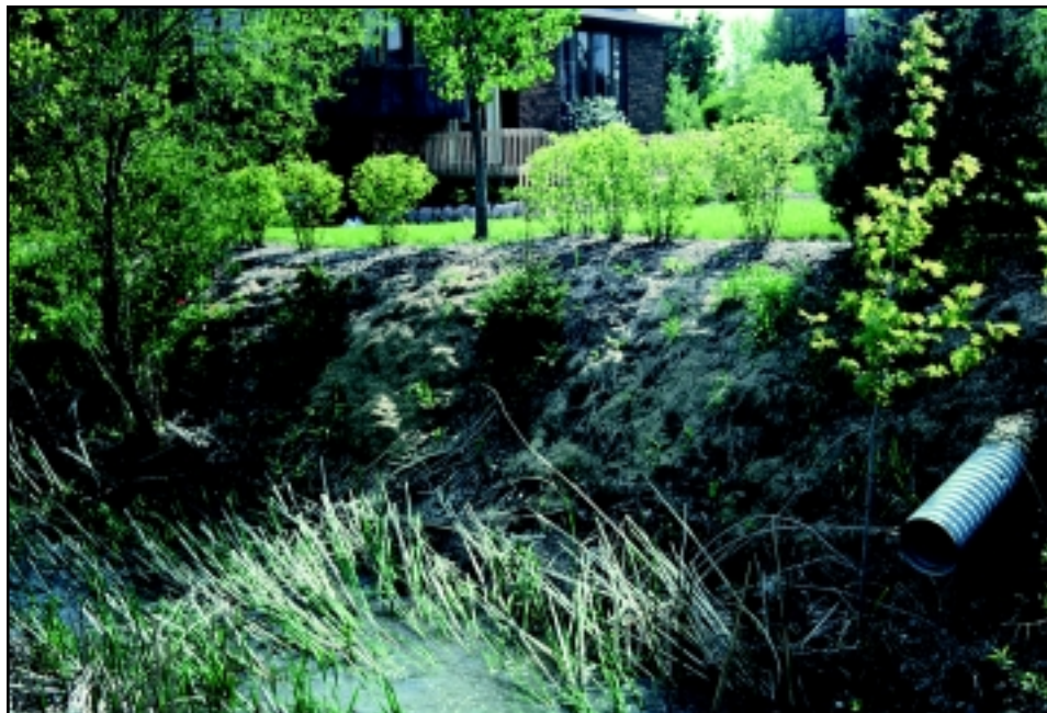
Underneath the lawn clippings is an exposed streambank. Invasive plants like the buckthorn shrub (to the right of the picture) and reed canary grass (in the water) offer no stabilizing roots to form. These invasive plants should be removed and replaced with native vegetation. And of course, no dumping!
