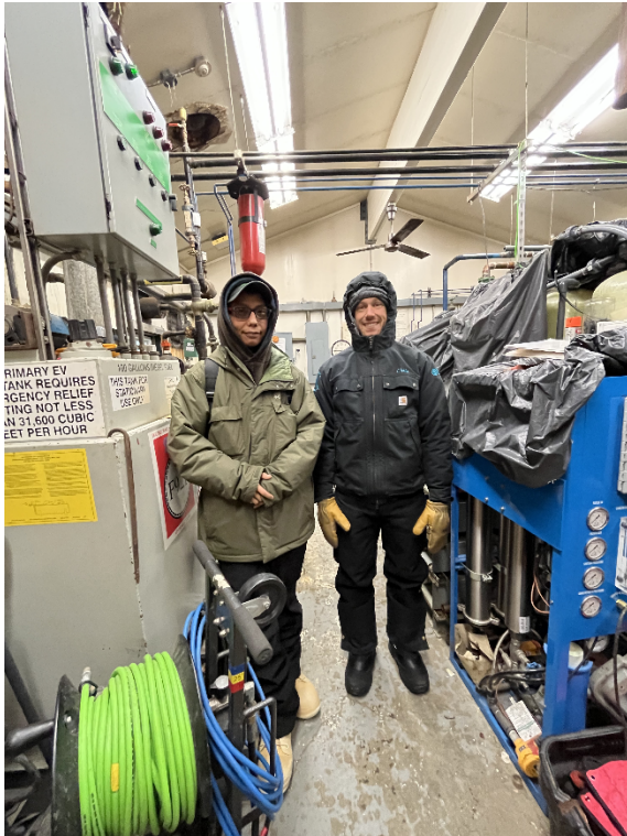
Diomedes Water Treatment Plant. Photo: Agnew::Beck Consulting.
