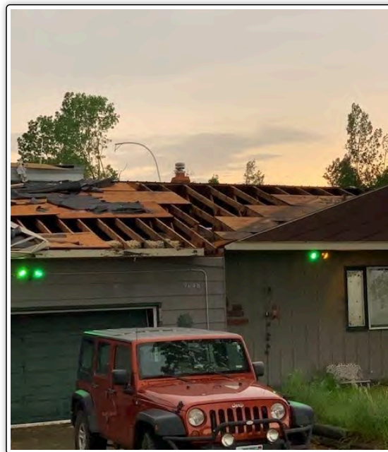
Damage in Ellendale, North Dakota
