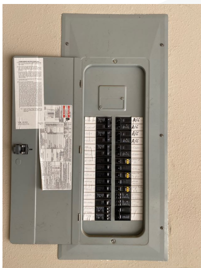
Electrical Service Panel
