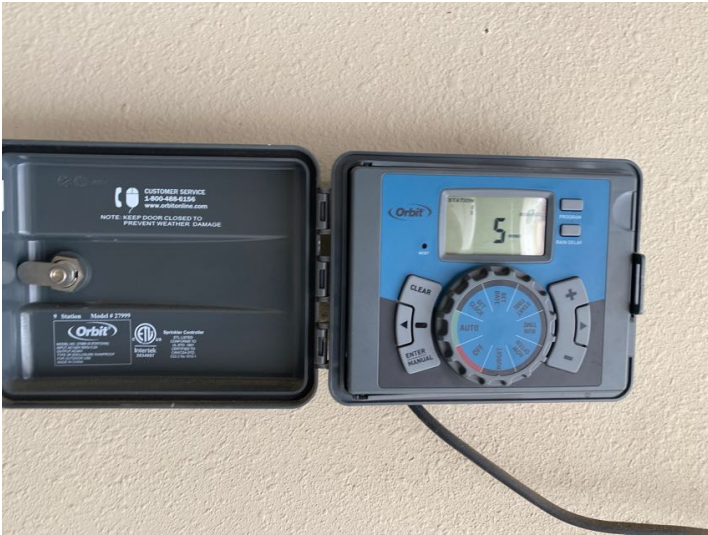
Sprinkler system head unit
