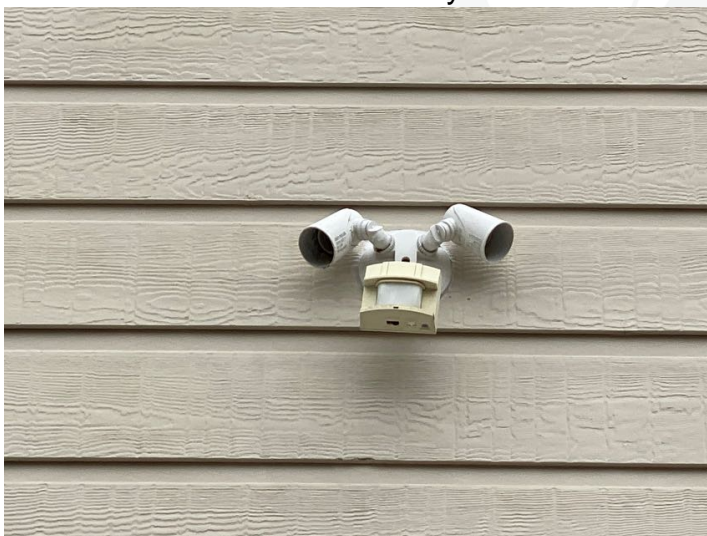
Light fixture not working properly, may have a short or may be in need of light bulb replacement.
