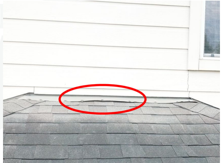
Flashing is lifting
