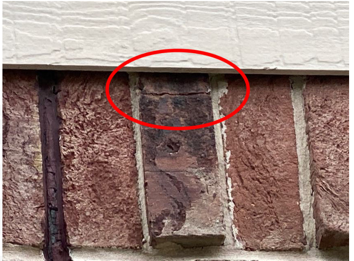
Cracking found in the exterior brick work
