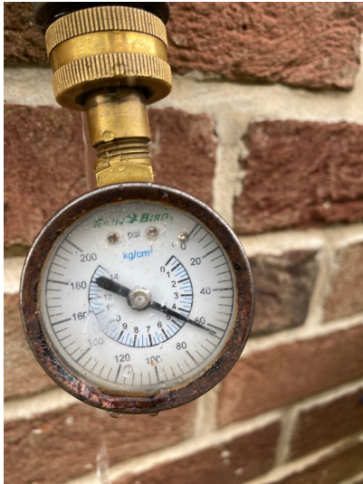
Static Water Pressure Reading: 63 PSI
