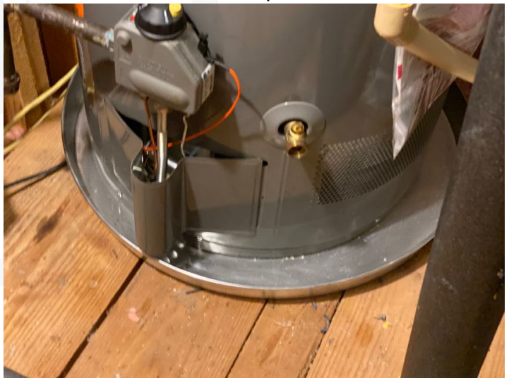
water heater drain pan
