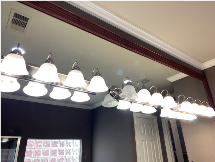
Light fixture not working properly, may have a short or may be in need of light bulb replacement.
