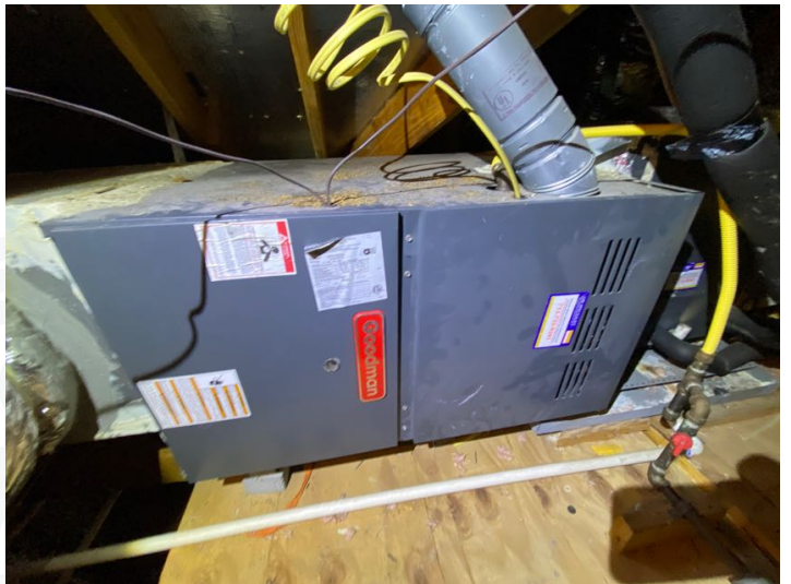
Downstairs heating equipment functions as intended
