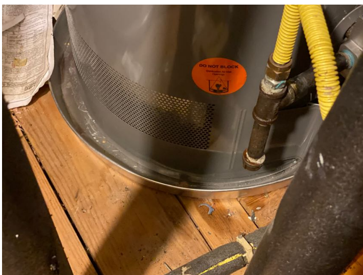
water heater drain pan
