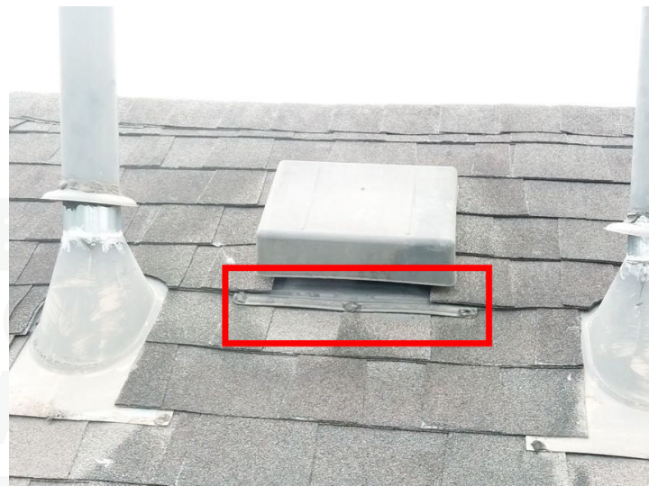
Flashing is lifting
