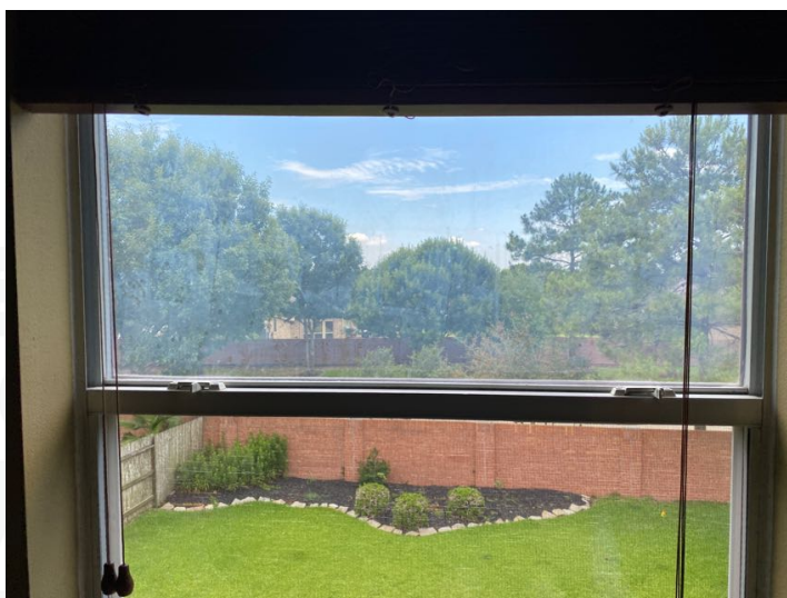
Fogged double pane windows present, When the window seals fail, your window actually has two seals. The desiccant within the window panes saturates with water. Now the insides of your window panes will fill with tiny amounts of water that we call: fog. This is an indicator of window failure, allowing the elements into the structure.
