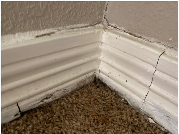
Deteriorated baseboards observed in the primary bedroom corner of a wall possibly due to apparent moisture damage coming from the primary bathroom shower.
