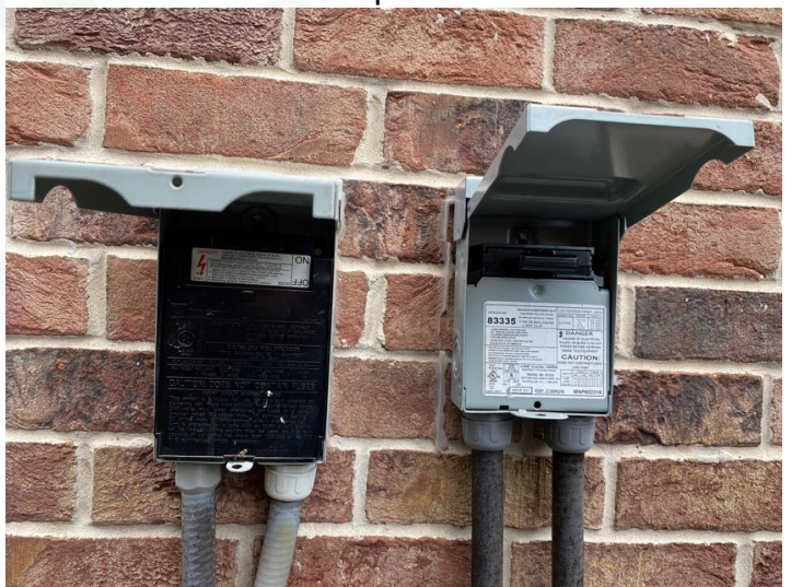
AC unit emergency shut off switches
