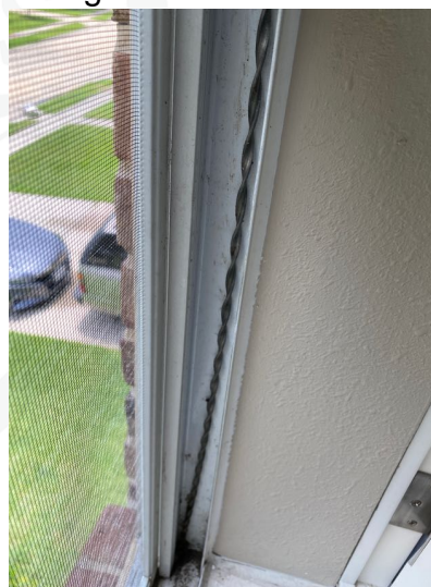
Broken/Damaged window channel balance rod assembly.
