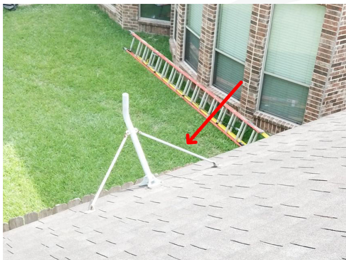
Satellite dish appears to be improperly installed. Fasteners appear to have been driven through the shingles compromising the roof covering.
