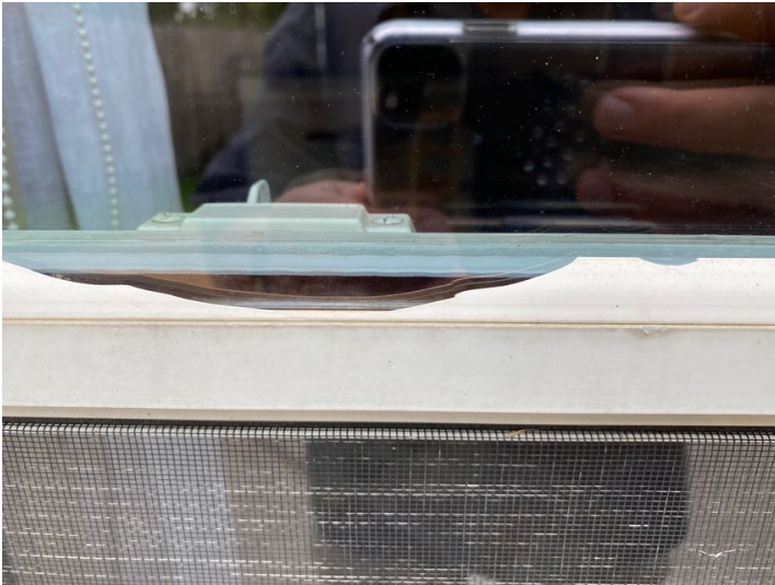
Damaged window frame beading observed.
