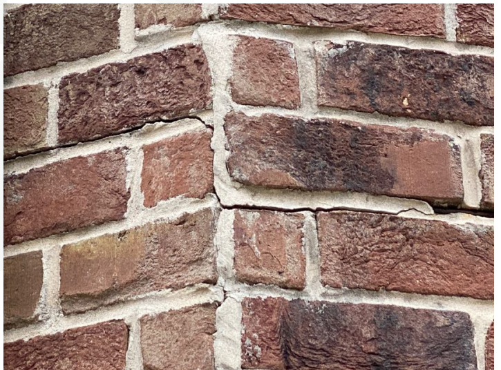
Missing or deteriorated mortar joints in between the brick(exterior)
