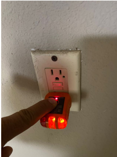
Garage electrical outlets are not GFCI protected
