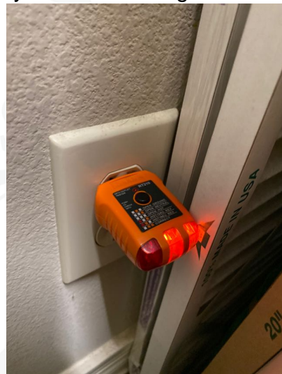
Laundry room electrical outlets are not GFCI protected
