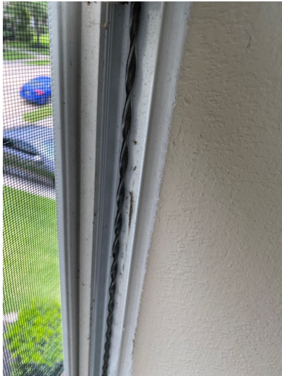
Broken/Damaged window channel balance rod assembly.
