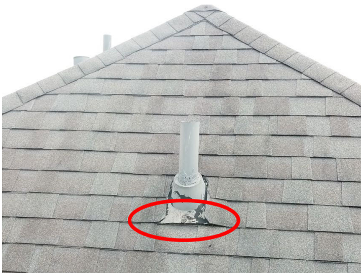
Plumbing vent pipe Perma-Boot flashing is lifting
