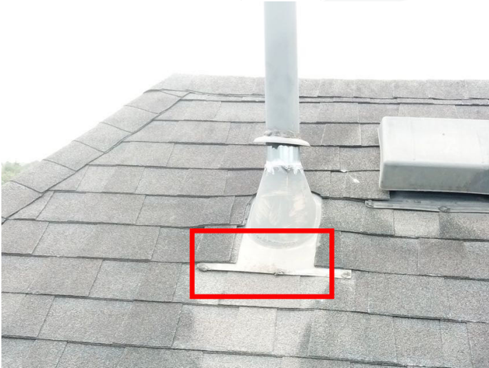
Flashing is lifting
