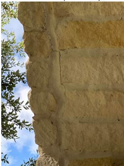
Missing or deteriorated mortar joints in between the brick(exterior)
