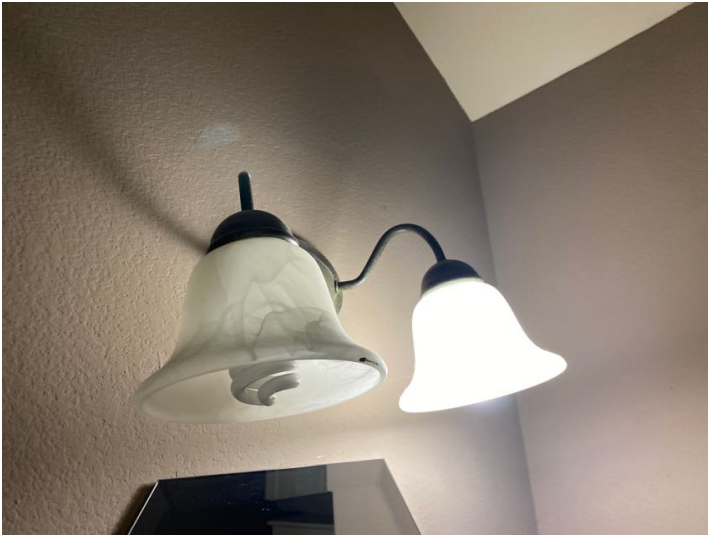
Light fixture not working properly, may have a short or may be in need of light bulb replacement.
