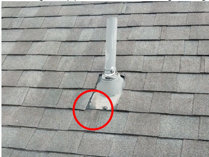
Plumbing vent pipe Perma-Boot flashing is lifting
