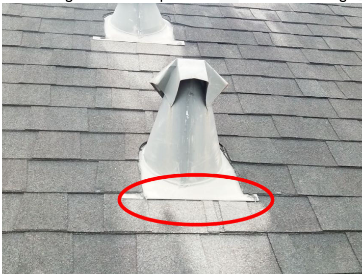
Flashing is lifting
