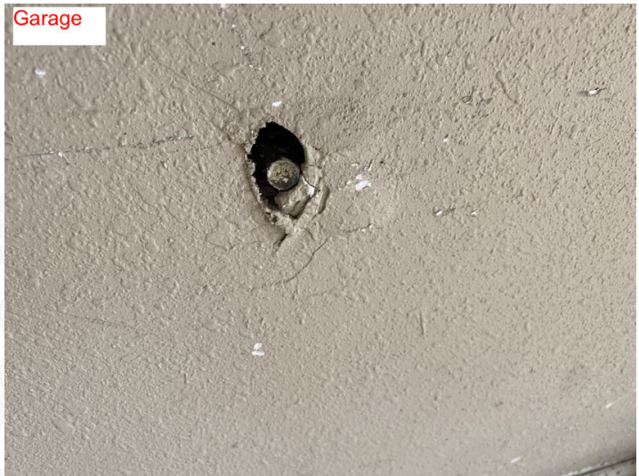
Damaged drywall observed.
