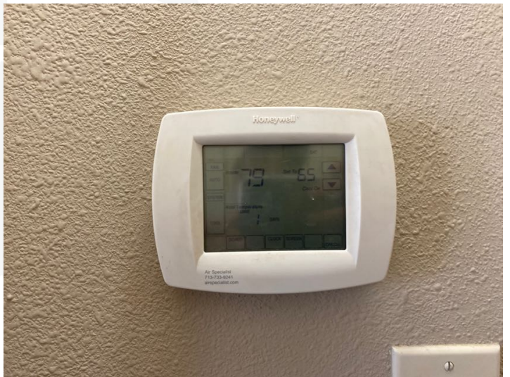
Thermostat(s) is/are functional
