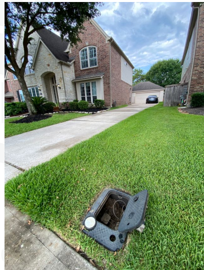
Location of water meter
