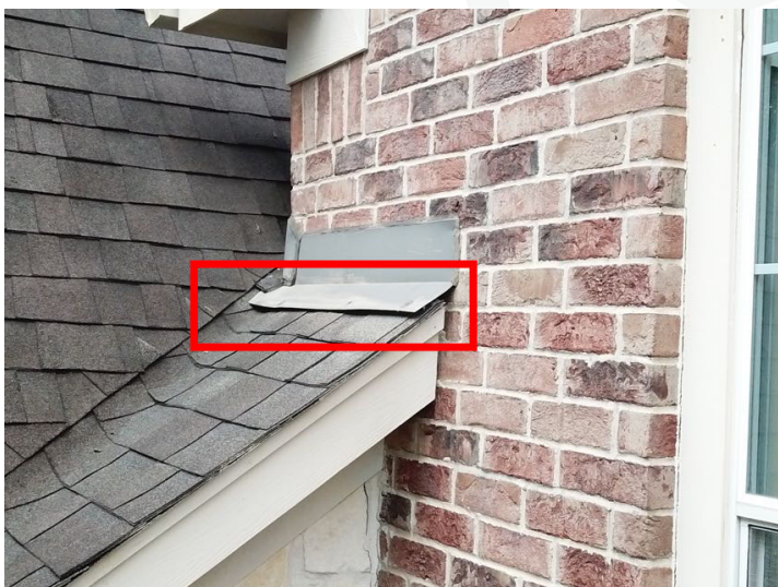
Flashing is lifting
