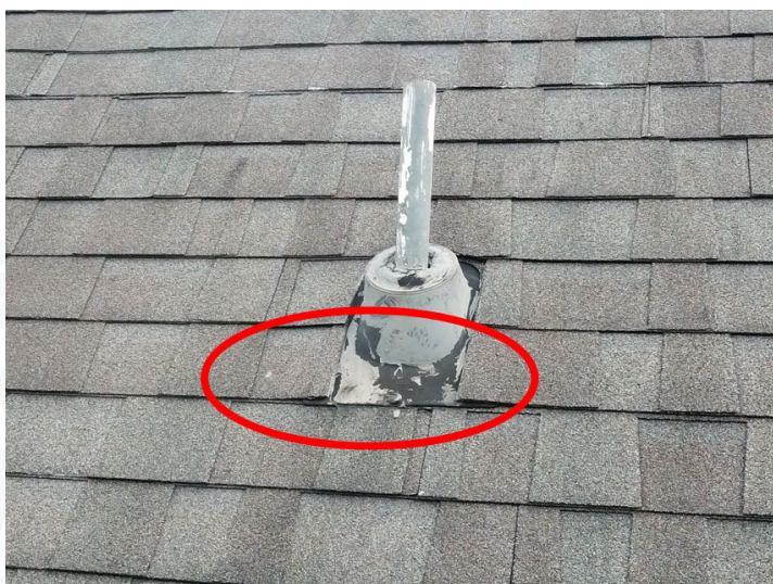
Plumbing vent pipe Perma-Boot flashing is lifting
