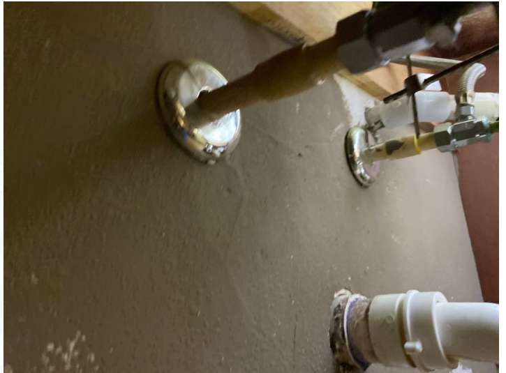
Type of Supply Piping Material: CPVC (Chlorinated Poly-Vinyl Chloride)
