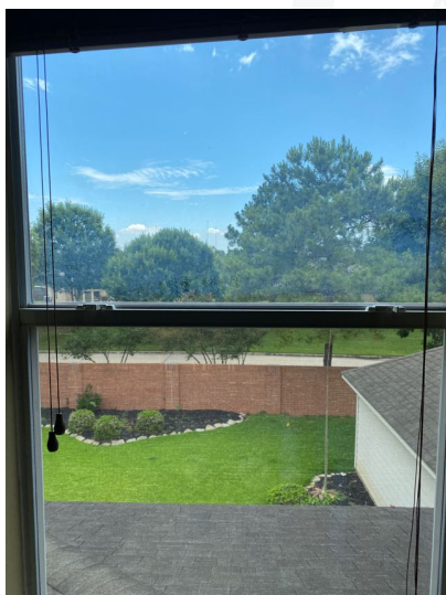
Fogged double pane windows present, When the window seals fail, your window actually has two seals. The desiccant within the window panes saturates with water. Now the insides of your window panes will fill with tiny amounts of water that we call: fog. This is an indicator of window failure, allowing the elements into the structure.
