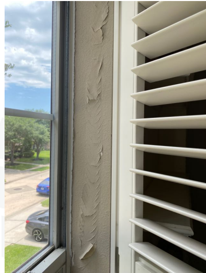
Peeling paint observed around upstairs office area window, this may be due to possible moisture related issues.
