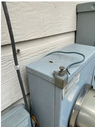
Electrical meter box is not properly secured to the wall.
