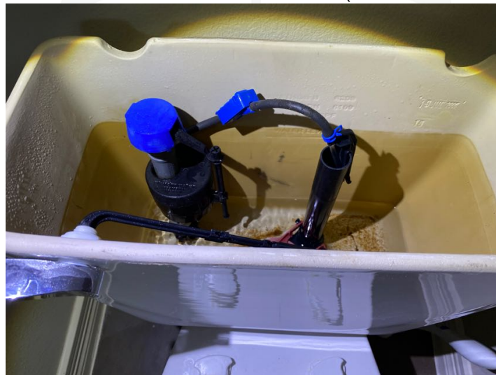
Toilet in the upstairs Jack and Jill guest bathroom does not flush properly. There appears to be an issue with the flush assembly causing it to run continuously after flushing.
