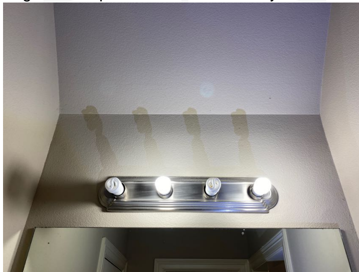
Light fixture not working properly, may have a short or may be in need of light bulb replacement.
