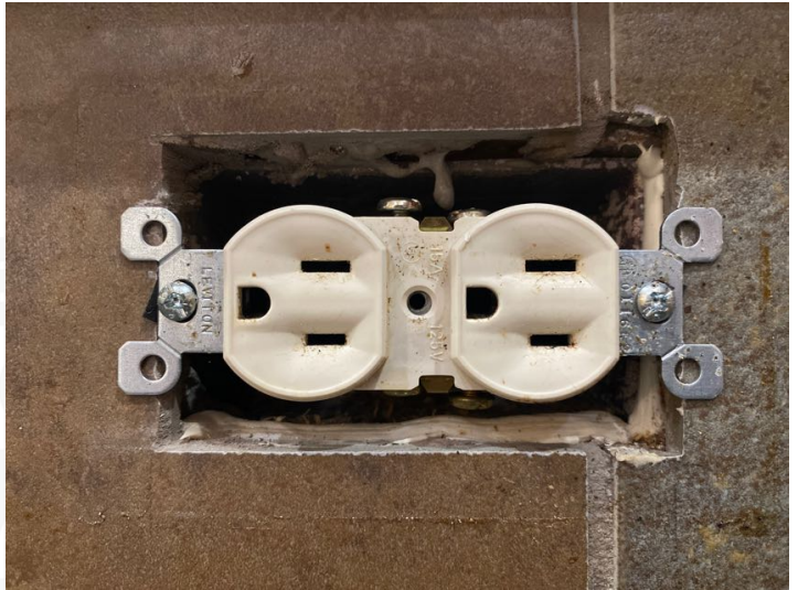
Missing box extender for electrical outlet in the kitchen area.
