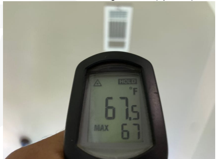
Delta T test at the register vent(downstairs)
