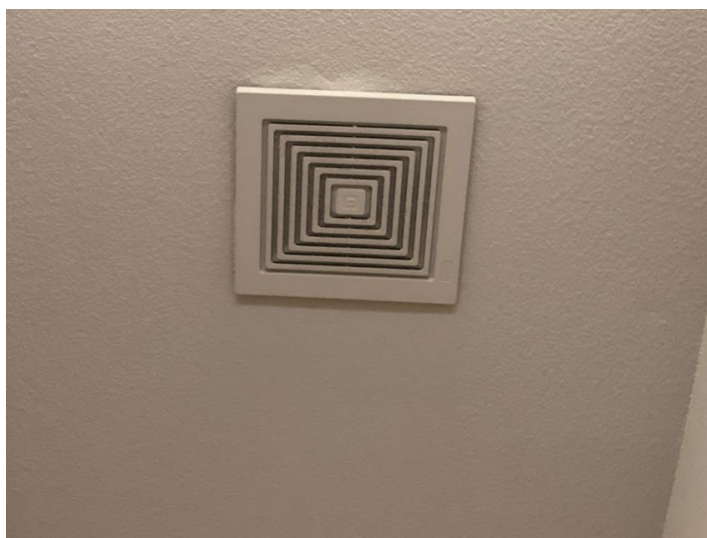
All bath and laundry fans operated normally
