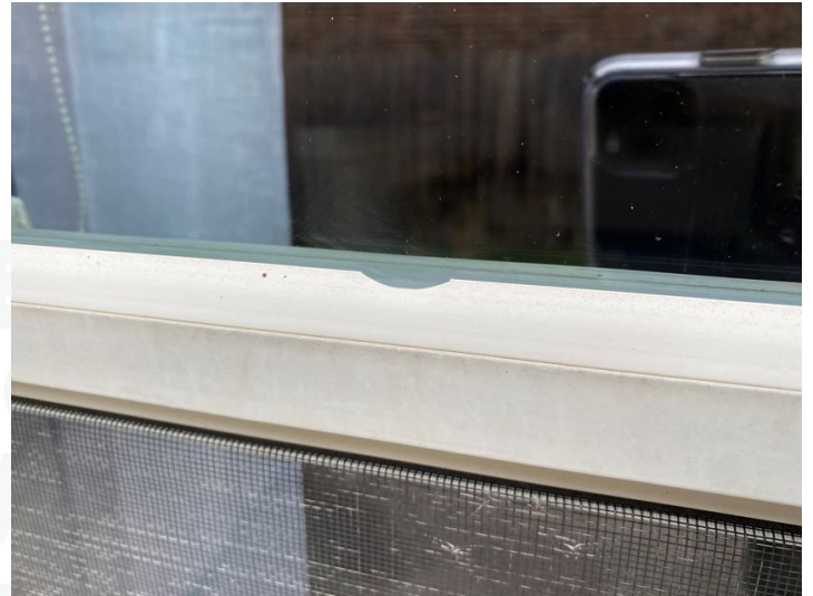
Damaged window frame beading observed.
