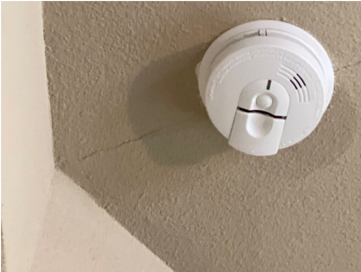
Small cracks on ceiling
