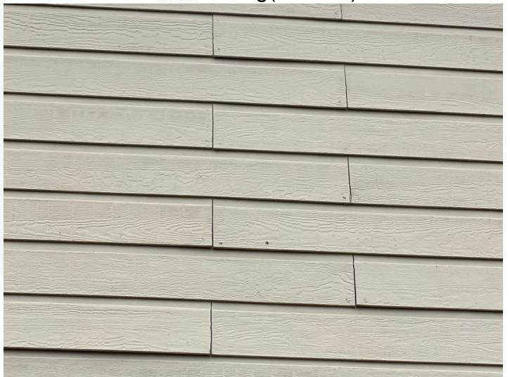
Missing or deteriorated caulking in between joints in the siding(exterior)
