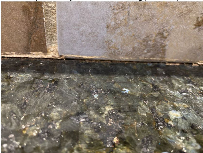
Missing or deteriorated grout lines around the kitchen sink area , this can allow water to penetrate behind the tiles and damage walls and or floor areas.
