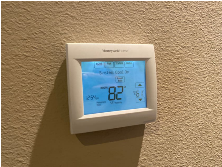
Thermostat(s) is/are functional
