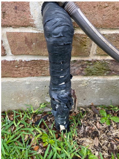
Main water shut off valve
