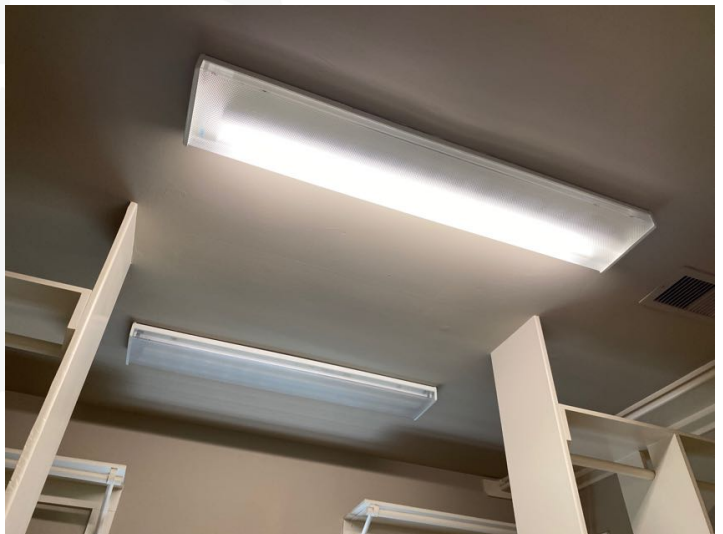
Light fixture not working properly, may have a short or may be in need of light bulb replacement.
