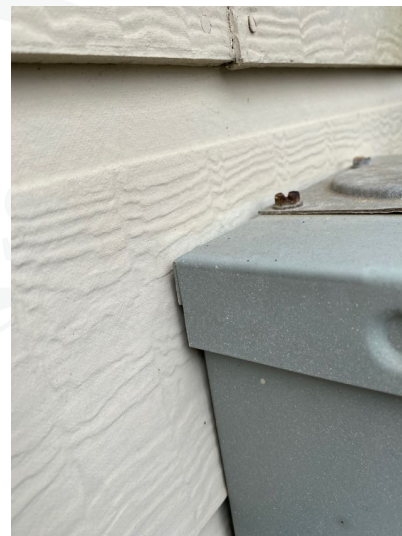
Electrical panel main disconnect box and electrical meter box lacks waterproof sealant at the top rear and side rear portions of the electrical panel to prevent moisture penetration from the rear of the electrical panel.
