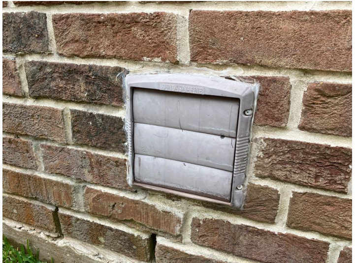
Self filtering with vent to the exterior
