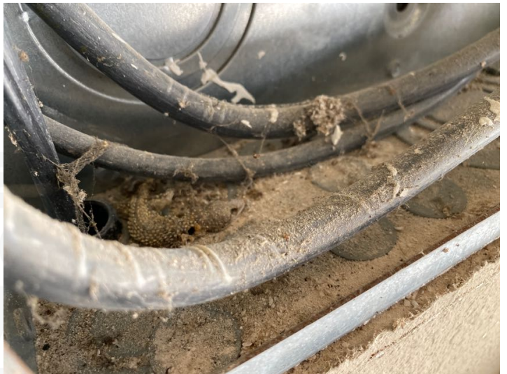
Debris/dust in the bottom of the electrical service panel.
