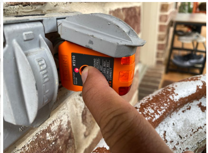
External house electrical outlets are not GFCI protected
