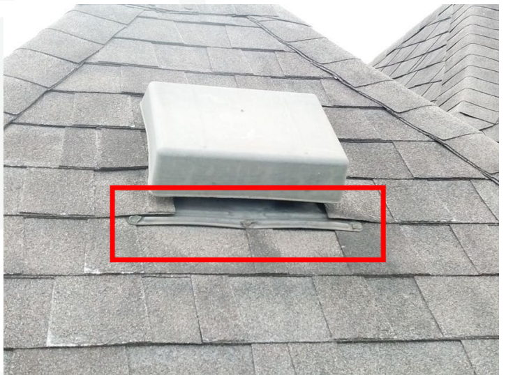
Flashing is lifting
