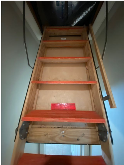
Missing insulation on the attic access door.
