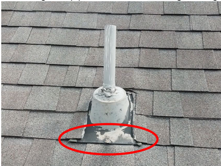
Plumbing vent pipe Perma-Boot flashing is lifting
