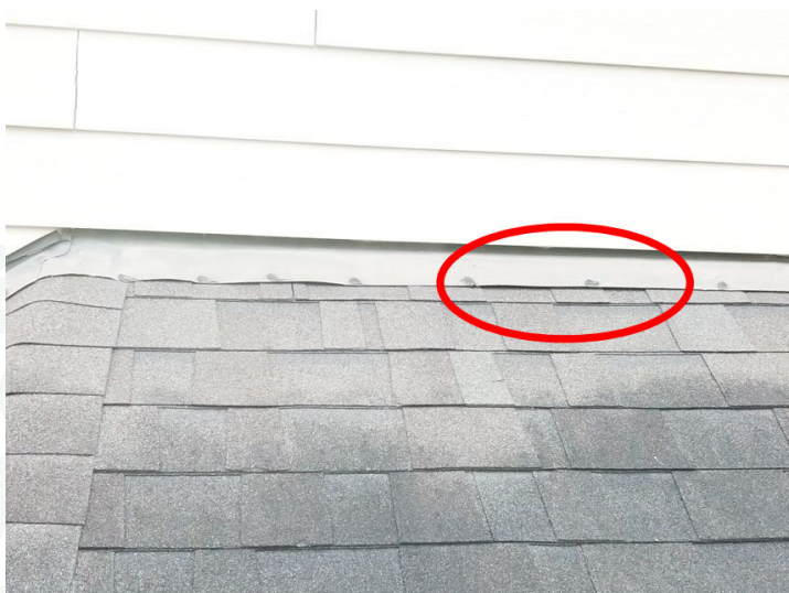
Flashing is lifting
