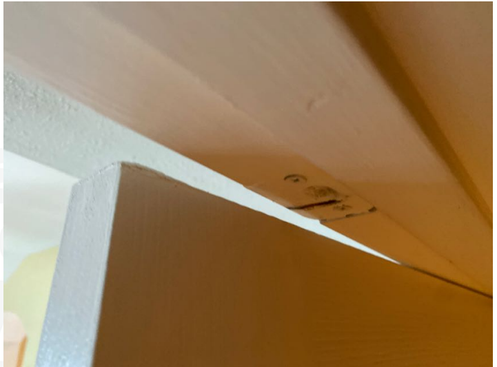
Doors to the upstairs media room do not latch properly
