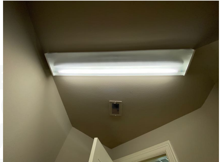
Light fixture not working properly, may have a short or may be in need of light bulb replacement.
