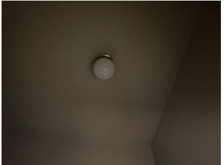
Light fixture not working properly, may have a short or may be in need of light bulb replacement.
