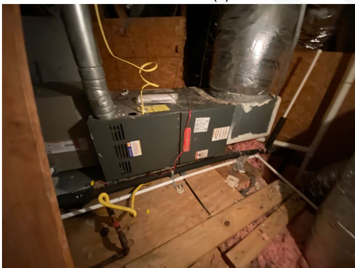
Upstairs heating equipment functions as intended
