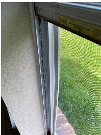
Broken/Damaged window channel balance rod assembly.
