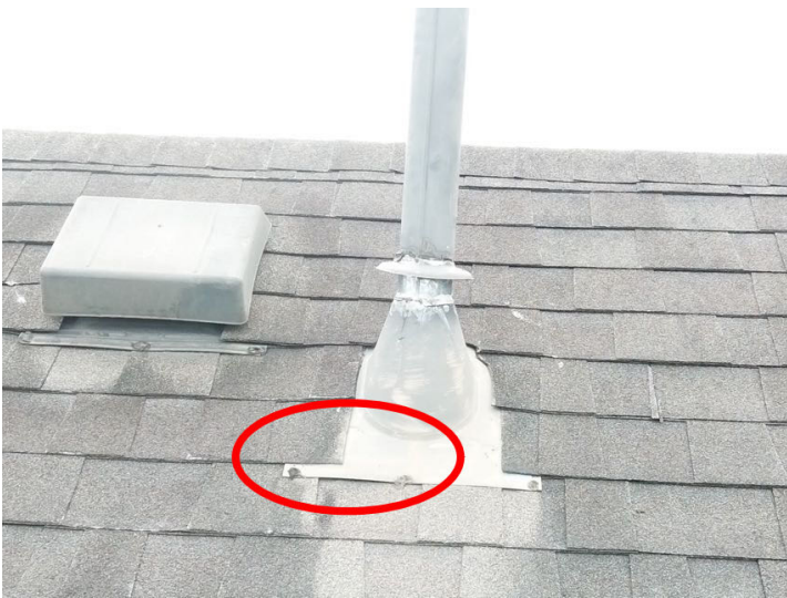
Flashing is lifting
