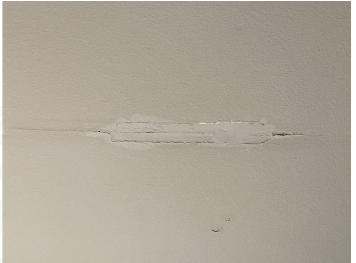
Ceiling damage observed in the primary bathroom.
